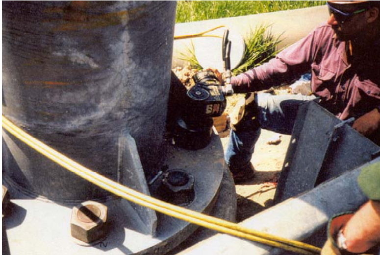
Figure 15. A Hydraulic Torque Wrench Tightening Anchor Rod Nuts to Achieve Needed Rotation.
