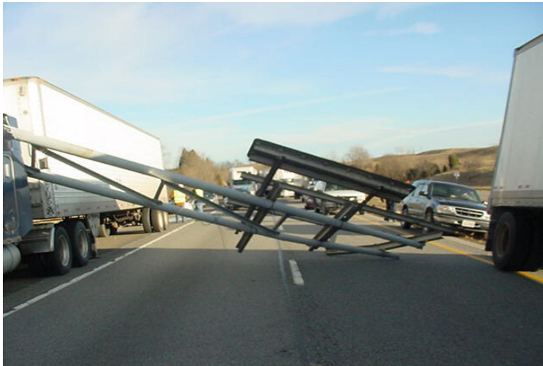
Figure 1. Cantilever Sign Structure Failure.
