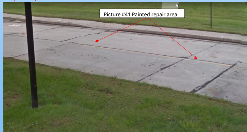
#42 2014 – I-80 Goehner WB rest area – Completed repair area in the 'thru' truck lane (parking on right in photo) this area is now closed off with tall delineators. All parking (trucks only) is to the north as of 2020. See photo #41 for painted repair area. In 2020 repair is still doing well since the access is closed.
