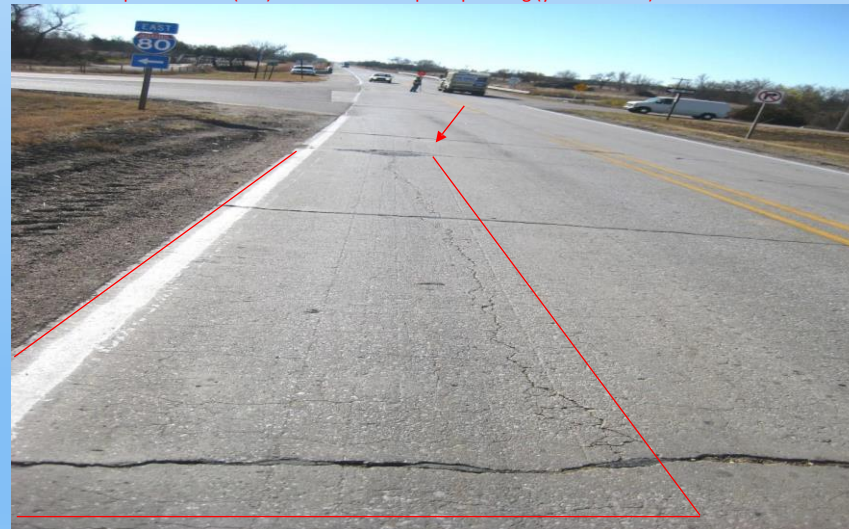
#22 N-10 (47.34 to 47.71) Looking south in the NB outside edge at a 32'x 5' repair with a delaminated crack and a 16'x 12' repair in the NB at the spall (red arrow). 2010 Why repair? Longitudinal crack has areas that are breaking up and is not stitchable. At the I-80 Interchange...
