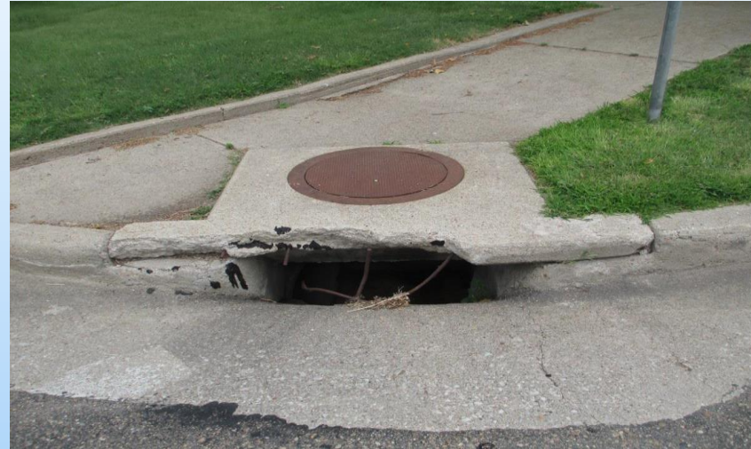
#9 L-31D (1.09-0.87) In Franklin - inlet lid, 6' wide (NE radius at 12 th Ave.). This lid was listed for replacement but the lid face was repaired with grout instead (per google maps)
