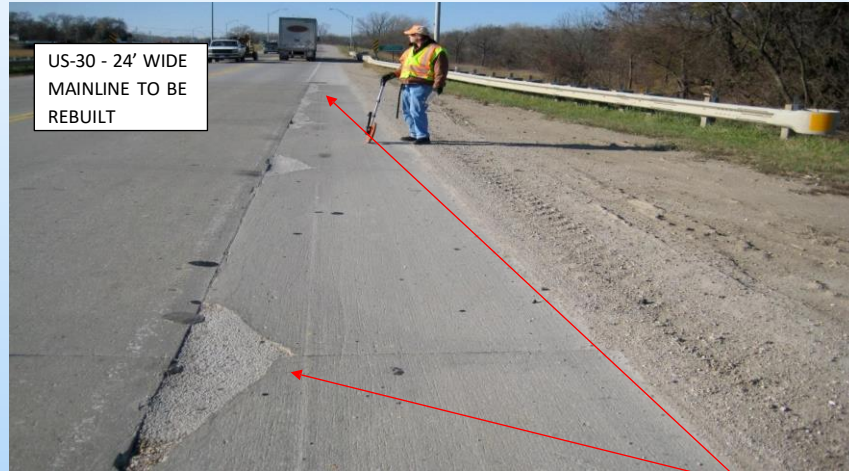
#7 US-30 (450.44 to 450.0) WB Looking west in the WB outside shoulder, inside edge at a 95'x 4' repair with spalls, staining, cracking, AC patching, and delamination. Note the 24' top will be rebuilt. 2009 - Why repair? Since mainline is to be rebuilt the shoulder needs to be able to be tied into the new adjacent pavement – patched areas and staining indicate that the inside edge needs to be repaired to prepare for the tying of the new pavement.
