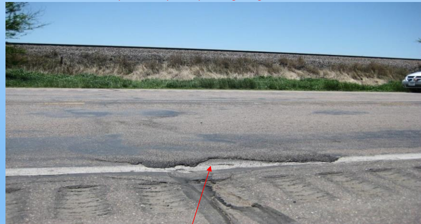
#34 US-6 (164.0 to 165.0) Looking south at AC shoving from the WB outside edge into the WB outside shoulder, inside edge. 2"+ (to 4") high lumpy AC makes for a rough ride. 2009 – Just because it looks like a needed repair area is it really an underlying concrete problem? No repair here – asphalt problem!
