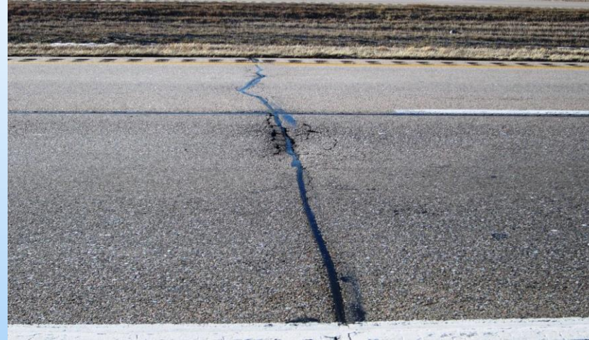
#35 I-80 WB RP 347.17 Looking south in the DL IE at a 4'x 5' repair (sunk) and a 4'x 12' repair in the PL that is borderline but looks slightly sunk. 2013 – Interstate 80 – if areas are sunken or raised is indicator of a needed repair to underlying concrete. Note that in the black text I state that the area in the passing lane is borderline repair and the area looks slightly sunk. This indicates the repair area could go either way – no repair or to repair – but taking based on visual cues...
