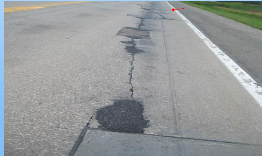
#24 N-35 (56.0 to 57.0) Looking west in the WB outside edge at a 45'x 6' repair that includes the AC existing repairs also adjacent to this repair is a 50'x 7' repair (red arrow). 2011 Why repair? With asphalt patching in the exposed section we try to remove the AC patching and replace with concrete for uniformity. Crack was removed with repairs.
