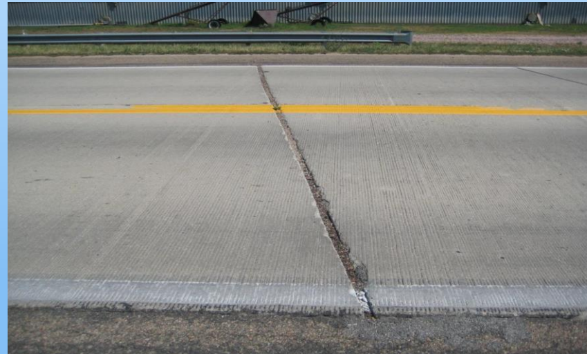
#14 N-2 (287.0 to 287.35) Sta. 424+03 PRJ open 1 1/2" and doing 5' x 24' joint repairs. Why repair? The old way was to remove all these pressure relief joints as they were encountered – I was never given a good reason why these needed to be removed. I leave them alone if no other issues involved. Note if open 6" plus than consider a repair/ removal.
