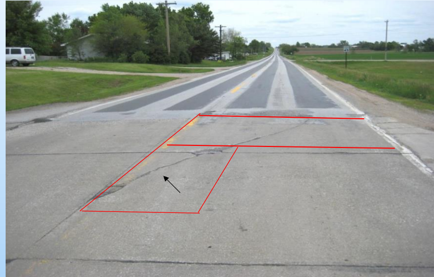
#19 N-103 RP 56.40 Looking north in the NB at a 12'x 4' & a 12'x 12' repair and Exposed Concrete to Full Depth Asphalt... 2010 Why repair? Repair area is at transition from concrete to full depth asphalt and diagonal crack in repair area may be due to this. Crack is should not be stitched due to transition.
