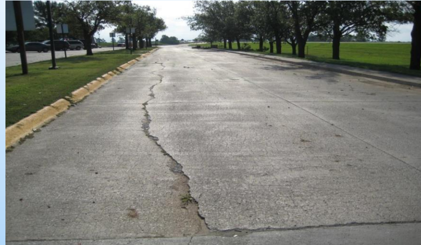
#43 I-80 WB Rest Area Sta. 17+18 Looking east in the truck lane, outside panel at not repairing longitudinal crack, is slightly faulted but does not have delamination or spalling. 2009 – I-80 Goehner WB rest area – Long longitudinal crack in the ‘thru’ truck lane’ – no repair in this area and hasn’t changed much in 10 years. Still looked good on the 2019 Repair survey. See Picture #44 for 2014 view of the area.
