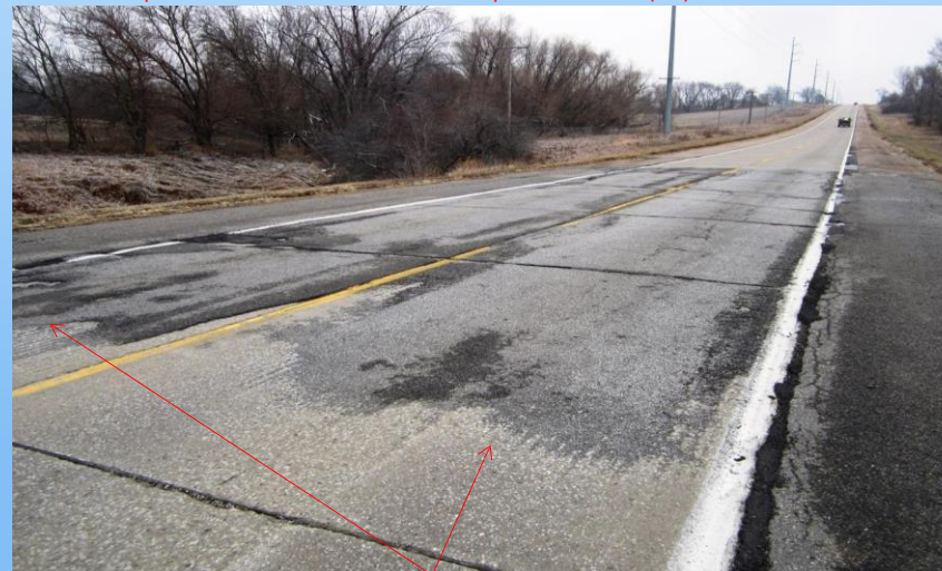
#26 N-31 (26.0 to 27.0) Looking north at a AC 'scab' that was milled before the asphaltic concrete (AC) was laid. This area will require a 90'x 24' repair/ replacement before diamond grinding... 2012 Why repair? If this was an asphalt overlay project we would just walk away from it but the scope is diamond grinding – since we do not diamond grind asphalt it must be removed for uniformity.
