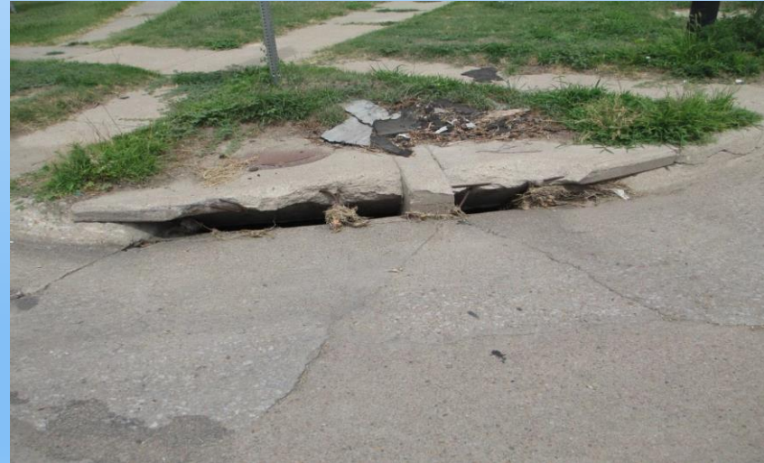
#8 L-31D (1.18-1.09) In Franklin - Inlet, broken lid is 10' wide w/8" solid concrete in middle. 2014 – This is one of the odd inlet covers in D7 – looks like was made in 3 pieces - Look at how low the lid is to the inlet throat. Has been replaced as of 2020 with new ADA ramp installation.
