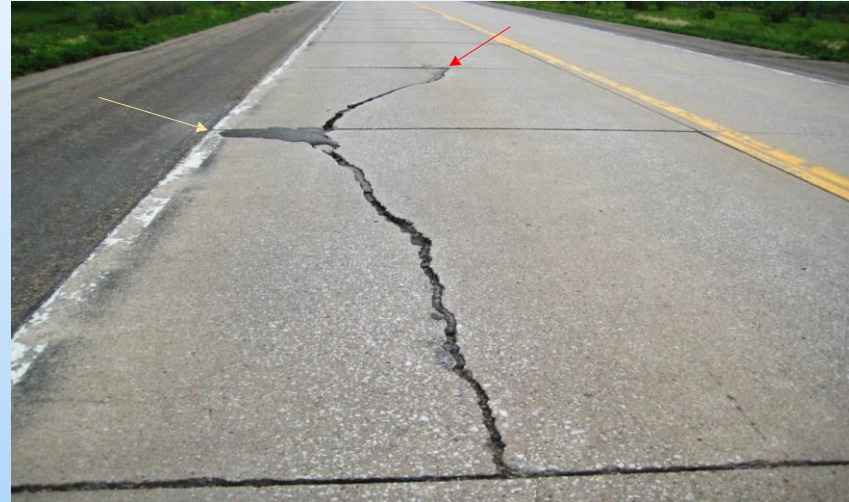
#21 N-92 (411.0 to 411.67) Looking east in the WB outside edge at a 35'x 7' repair with a 1" open longitudinal crack, faulted, and spalled. 2010 – Why repair? Open faulted crack with no concrete shoulder and panel is sunk (red arrow) and has asphalt patching (yellow arrow).
