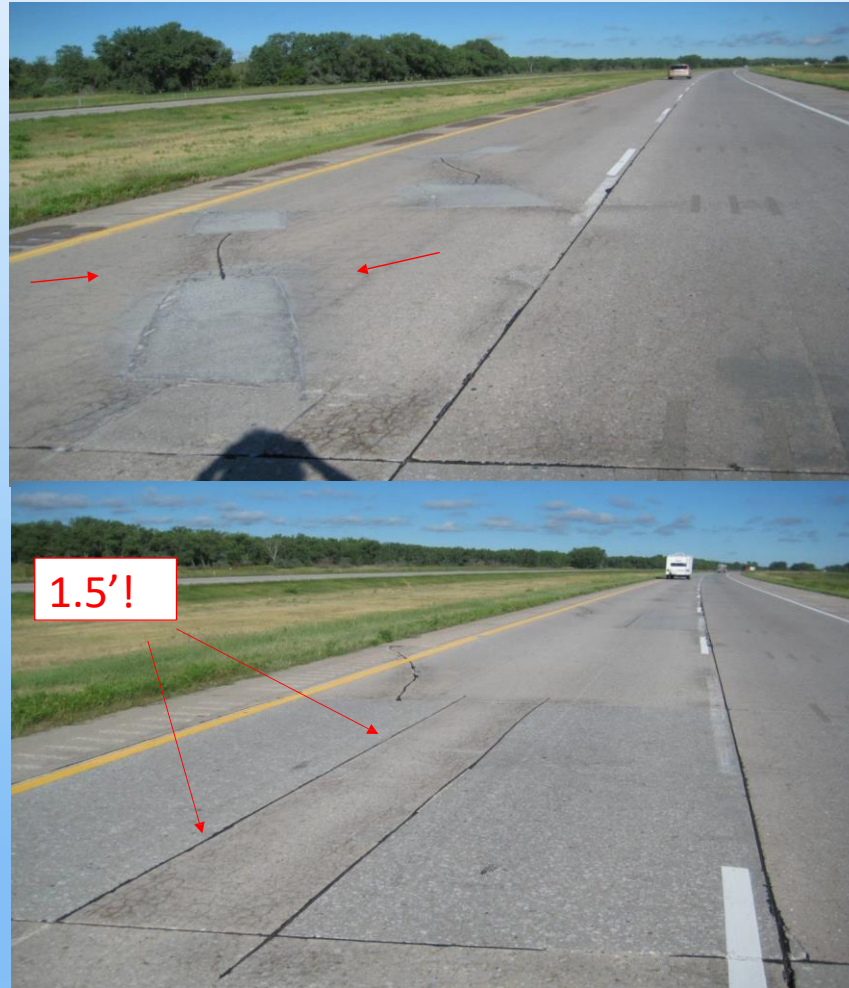
#12 I-80 Looking west in the WB passing lane at two more odd repairs with 1.5' left in between the two existing repairs. This area will not be repaired at this time (no delamination). Why not repair? Other than the staining there is nothing 'wrong' with the area – just odd repair placement.
