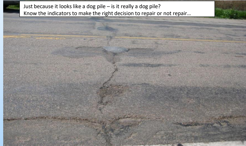
#33 US-6 (160.0 to 161.0) Looking south at AC scoured in the wheel tracks and transverse joints. AC looks like soil in the scoured areas, very brittle. Many areas similar EB and WB. No repairs – definite AC problem! 2009 – Just because it looks like a needed repair area is it really an underlying concrete problem? I see it as: Asphalt is called flexible pavement and it flexes, loading can cause rutting then the oil eventually leaches out and it becomes dry and brittle, it starts scouring (eating itself away). The concrete base is not usually affected by the asphalt degrading unless it not sealed and water infiltrates
