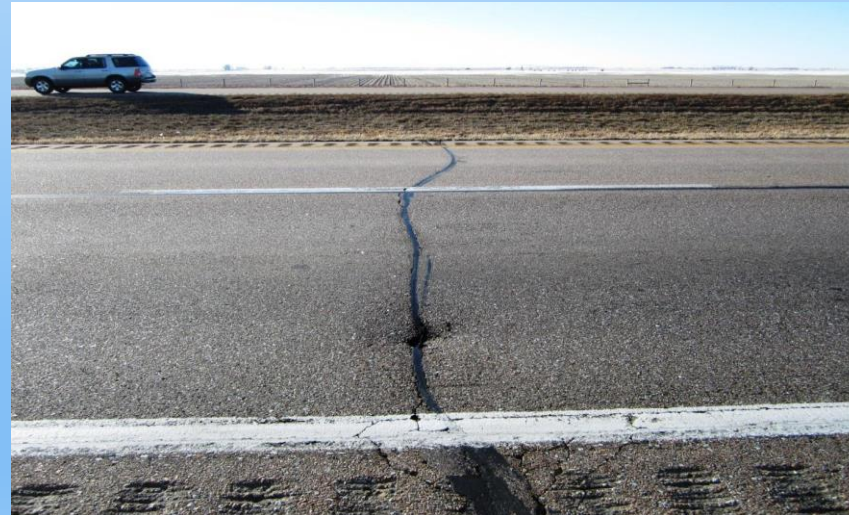
#36 I-80 WB RP 346.91 Looking south at a 4'x 5' repair in the DL OE at a hole with area sunk. 2013 – Interstate 80 – if areas are sunken or raised is indicator of a needed repair to underlying concrete.
