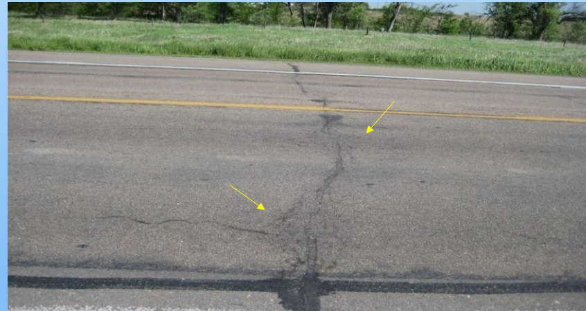
#32 US-6 Looking north at the EB at a typical area with indications of a repair, many areas similar. Will not be taking this area due to depth of AC (7.25" average) and due to the large cost if we listed all these areas. Was hard to let these go unrepaired but ... 2009 – These areas were not sunk or raised – only indication was the 'scallop' cracks (yellow arrows). Scallop cracks cannot be the only indicator – has to have a secondary indicator such as sunk, raised, milled down, or fines pumping. This section is still performing well. forces crack sealed in February 2018 – Schedule for a Mill & Fill in 2023 (CN performing 08/25/2020)
