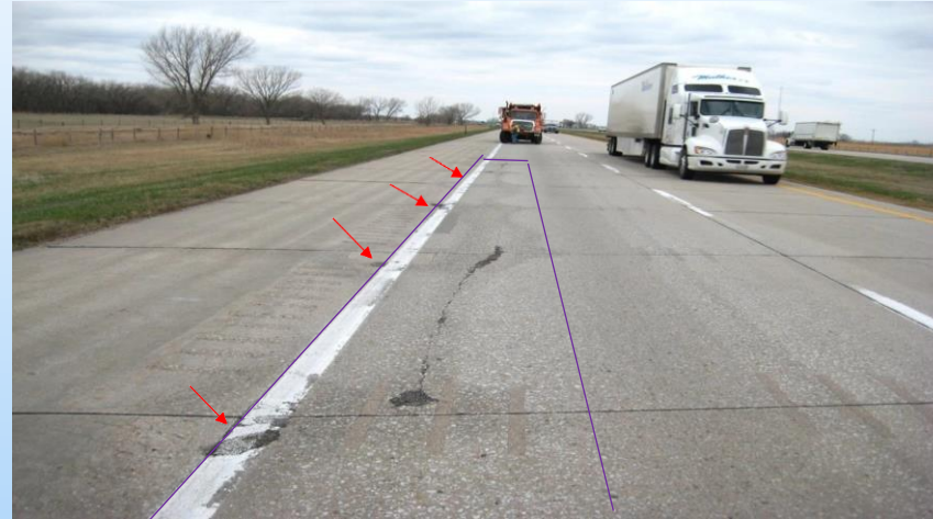
#15 I-80 EB (219.0 to 220.0) Looking west in the EB driving lane outside edge at a 105' x 5' repair (purple lines) with a longitudinal crack with delamination. Note 2' x 2's in the OS inside edge (red arrows)... Why repair? Longitudinal crack is in the outside wheel track running thru the retrofit slots with staining and delamination. Small partial repairs on outside shoulder need to be sounded before deciding if a repair is needed in the area.
