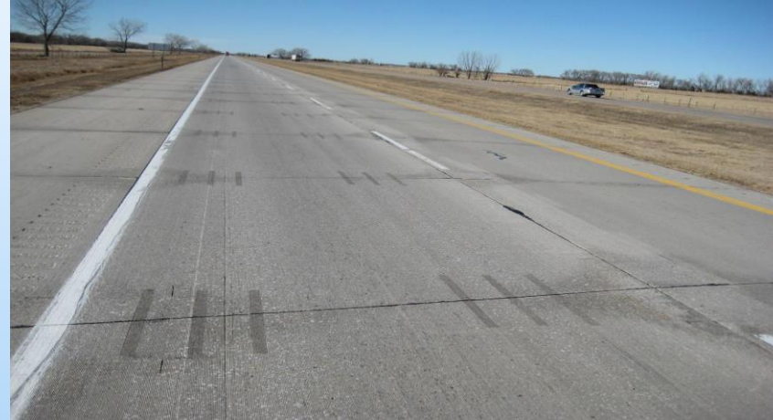
#31 I-80 EB (205.61 to 206.0) Looking west in the driving lane at ASR staining at the joints and retrofits. Note that this 'look' is typical for advanced ASR pavement areas in this project. 2014 – Shows typical ASR staining at the dowel bar retrofits and the outside shoulder at the transverse joints. Have to sound all the areas to determine which can stay and which will be repaired.
