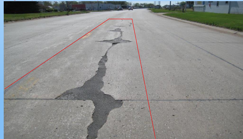
#28 US-275 (20.75-21.0) Looking east, inside panel inside edge, repair needed 60'x6'. 2012 Why repair? We are not able to stitch this wide crack and have it hold plus with all the asphalt patching in the crack – this is an indicator that it needs to be removed and repaired.
