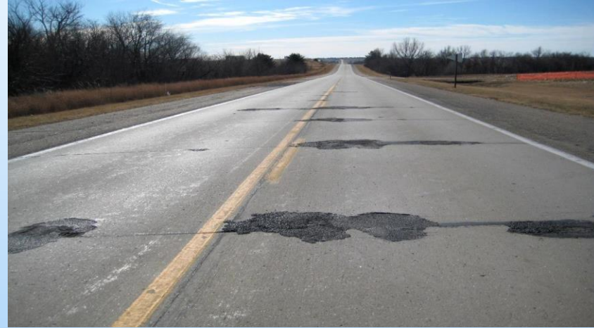
#29 US-73 (9.0-8.21) looking south at several joint repairs needed in both lanes. Why repair? These are larger patched areas that will need to be repaired – especially if to remain exposed concrete. If to be AC overlaid – some of the smaller areas adjacent to the larger patches could be omitted from the repair listing. If to be concrete surface milled most repair areas could be omitted...
