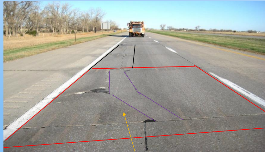
#16 I-80 EB (220.0 to 221.0) Looking west in the EB driving lane at a 21' x 12' repair (red lines) and a 39' x 5' repair (black lines) in the outside edge. Note the odd shaped repair – purple lines (like bottom of lower case 't'). Why repair? Odd shaped repair is partially in wheel track plus cracking and staining. Cannot remove odd shaped repair without going into retrofit slot on left.
