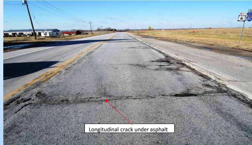
#25 US-6 (309.0 to 309.15) Looking west in the WB at a 40'x 11' repair with large pot holes and AC patching. NW 56 th St. is just behind this picture. 2011 Why repair? Large pot holes w/ possible longit crack under asphalt in same area. Remove full under pavement width (11'). Alternate I-80 route...
