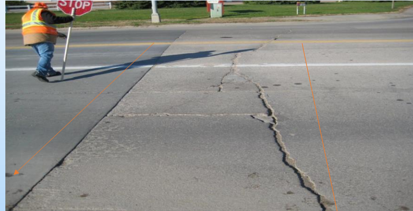
US-283 (57.70 to 58.0) & (Ash St. to Washington St.) Looking west in the NB at three repairs: a 9'x 12' repair in the left turn lane and the inside panel, a 9'x 14.5' repair in the outside panel. All with open or faulted cracks. From 2009 – Why take these areas? With a large solid existing repair on the left that has no indications of any needed repairs – the 'continuation' of the repair area makes the most sense with open 'Y' & 'T' and Transverse cracks.
