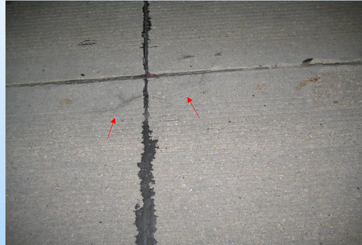
#45 I-680, I-80 to Fort St. Many areas like this delaminated and did a 4' x 4' joint repair. (ZIP days - 6"x 3" to 4" wide area and doing a 4'x4' joint repair? Seems over excessive!) Partial depth repairs in D2 are forbidden! I would leave this to be sealed – rather than take a chance on a PR repair. This area is a doweled concrete pavement section...
