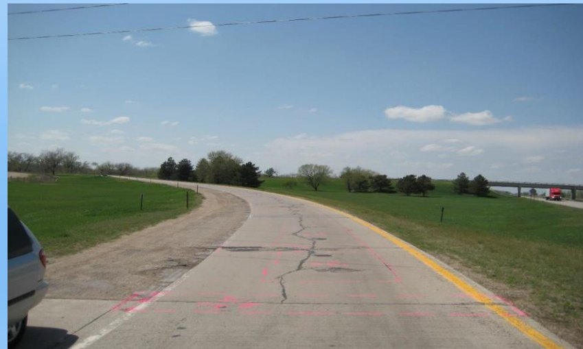
#20 I-80 Exit #231 Darr Interchange Looking up Eastbound on ramp at all the repairs painted and rotten AC shoulder. 2008 Exposed Interstate ramps should be repaired – these are essential to moving of traffic on and off the interstate –also hard for maintenance forces to repair w/o backing up traffic.
