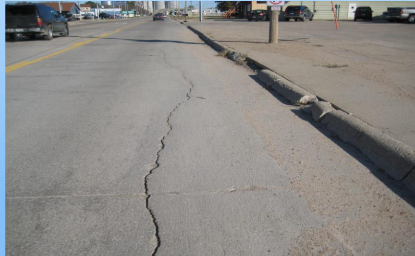
#2 US-283 (57.70 to 58.0) & (Ash St. to Washington St.) Looking north in the NB outside panel, outside edge at a 67'x 6.5' repair that includes the integral curb. Why repair and not stitch? Note the staining adjacent to the longitudinal crack – the stitching bars may not hold on this stretch due to loading (US- 283 In Lexington – truck route!). Adjacent broken curb is included in the full depth repair.
