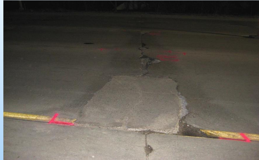
#39 US-75 NB Looking east in the NB Lane #1 at a 6'x 12' repair that includes the delaminated existing repair. Note the staining and spalls... 2011 – Painted repair in Lane 1 with failed repair and adjacent staining and delamination. Odd repair mix...
