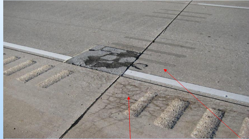
#9 I-80 EB (201.0 to 202.0) Looking northwest in the EB driving lane, outside edge at a 4' x 5' joint repair with a AC existing repair and note the 2.5' x 2' partial depth repair in the outside shoulder. Why repair? Partial depth in retrofitted area sunk and has been replaced with AC. The outside shoulder inside edge is delaminated but not spalled – partials are not allowed in retrofitted area.
