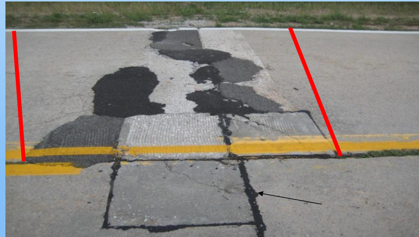
#6 US-30 Looking north in the WB at a 7'x 12' joint repair that includes existing repairs, area milled with AC patching. Note the cracked delaminated partial repair in EB inside edge. Area with red lines has failed with multiple AC patches – always list this type of area for removal – cracked partial was listed to be repaired with another partial depth repair. If to be overlaid may just leave the partial...
