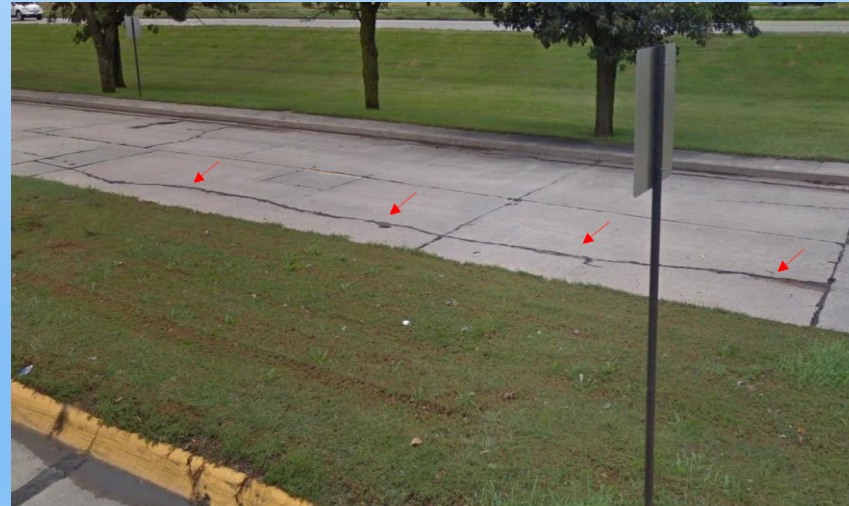
#44 2014 – I-80 Goehner WB rest area – Long longitudinal crack in the ‘thru’ truck lane’ – still hanging tough after 10 years –due to old RCP with the wire mesh – mesh still holding concrete together.
