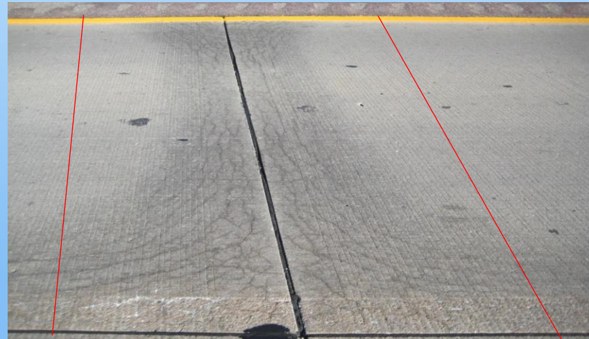
#30 I-80 (371.03 to 372.0) Sta. 983+62 Looking north in the EB passing lane at a 4'x 12' joint repair with alkali gel, discolored, and delaminated. 2010 – Question from the field was 'Why leave some of the stained areas on the edge associated with this repair?' Answers 1. To be overlaid & 2. When we sound the pavement we determine the limits – staining doesn't always mean delamination.
