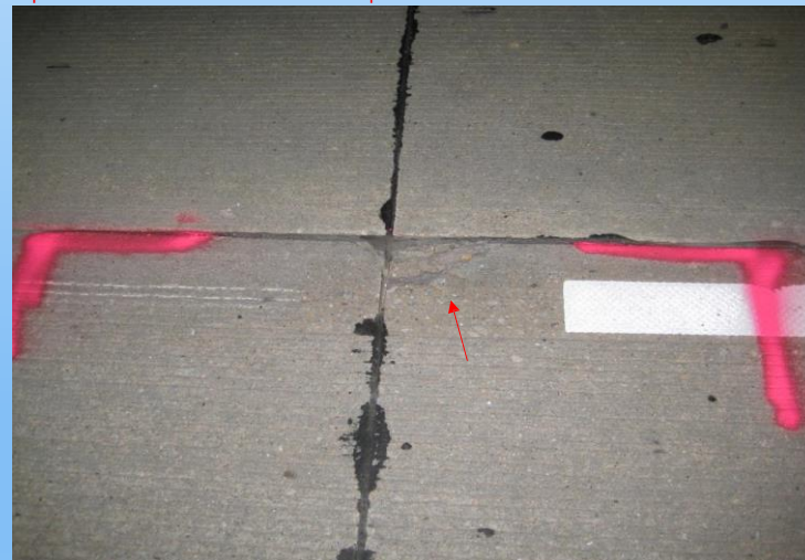
#46 I-680, I-80 to Fort St. Many small spalled and delaminated areas 6"x 3" to 4" wide, doing 4' x 4' joint repairs. (ZIP days - 6"x 3" to 4" wide area and doing a 4'x4' joint repair? Seems over excessive!) I would leave this to be sealed.... This area is a doweled concrete pavement section.
