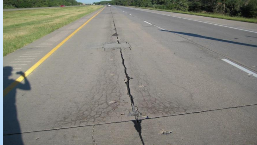
#13 I-80 WB (202.0 to 201.0) Looking west in the WB passing lane, middle of lane at a 137'x 5' full depth repair with spalls, delamination, and staining. Why repair? The cross stitching holes are all delaminated and will need repaired – spalls starting to show on crack - this area will begin to break out
