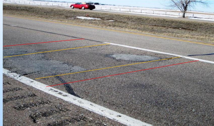
#37 I-80 EB RP 350.89 Looking northwest at a 12'x 12' repair in the driving lane. Looks like a broken existing repair under the surface of the AC with large AC patches. 2013 – Interstate 80 – Failed existing repair area (orange lines) under asphalt. Red lines = Listed repair area. Lines are approximate...
