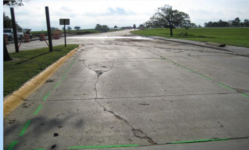
#41 I-80 WB Rest Area Looking east in the truck lanes at a 23'x 11' repair in the outside panel (note the green outline of the repair area) with multiple cracks, spalling, and delamination. 2009 – I-80 Goehner WB rest area – Large repair area in the 'thru' truck lane (parking on right in photo) this area is now closed off with tall delineators – All parking (trucks only) is to the north as of 2020. See photo #42 for completed repair.
