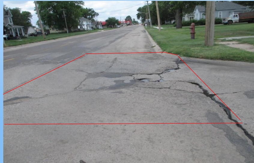
#10 US-136 (52.41-52.24) In Franklin WB-OP, NW radius at 18 th Ave., looking west at 20' x 18' repair needed. This needed repair is in a intersection radius and should be poured in one patch area. Avoid making several smaller patches to make the larger repairs especially in turning areas.
