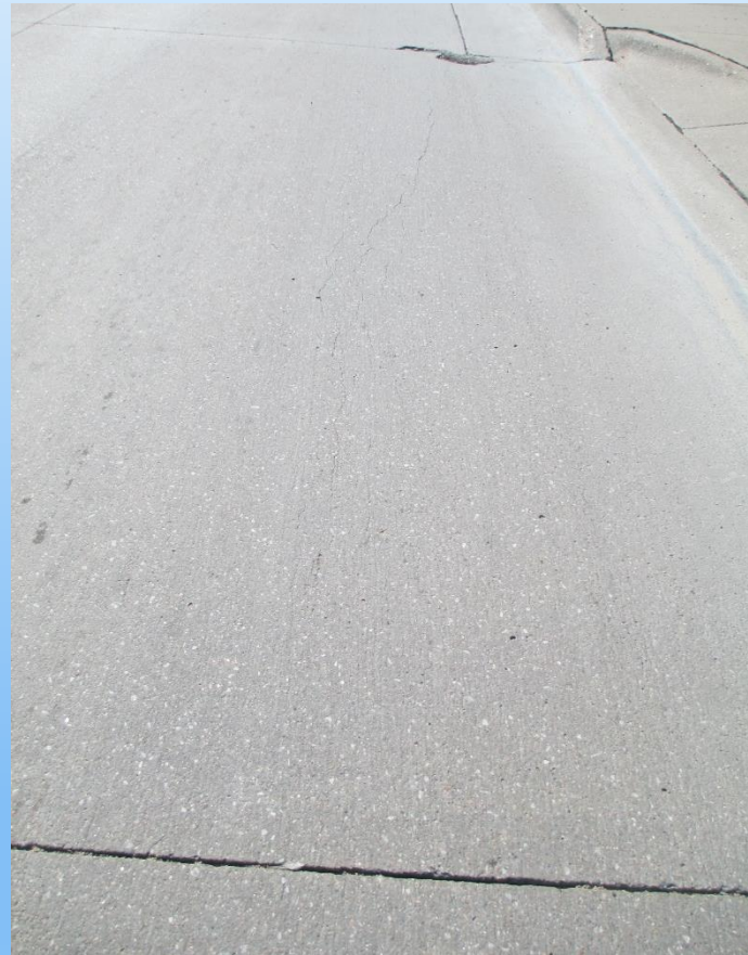
Crack is bound No Cross-stitching
