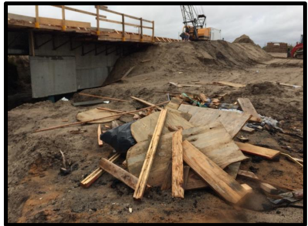
Figure 2: Ensure that construction debris and materials are properly disposed and that these are not accumulating within a Restricted Use Area.
