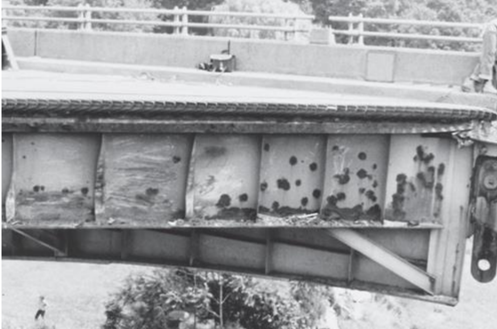
Figure 2.1 Mianus River Bridge collapse (Connor et al. 2005).
