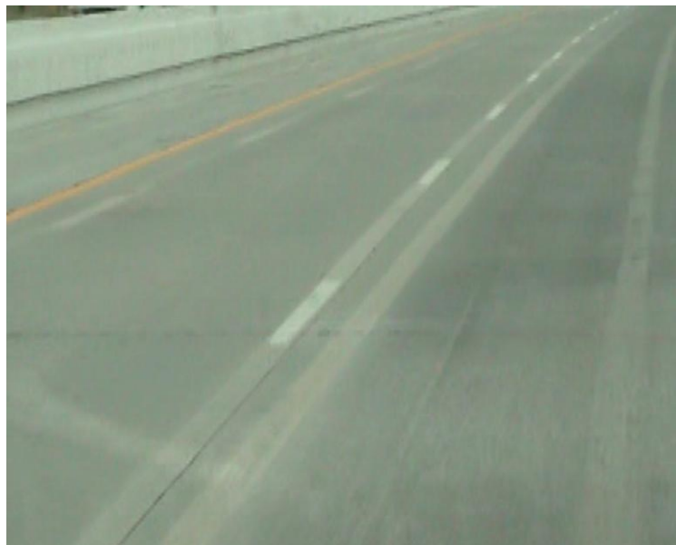
Figure 2.1. Scars on I-80 that can confuse drivers
