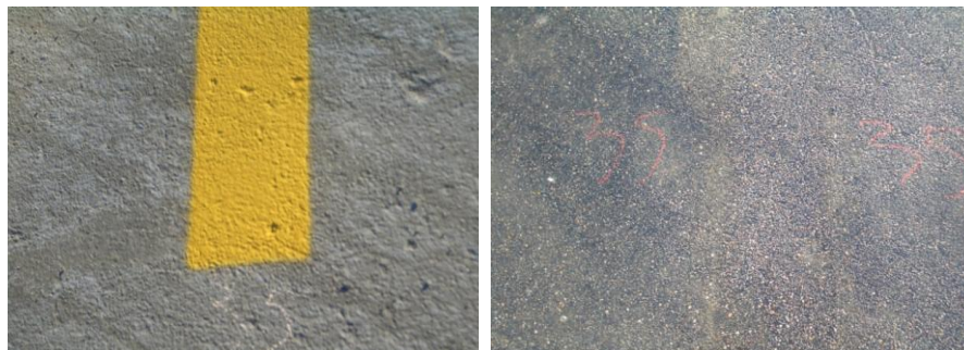
Figure 6.19. Asphalt pavement condition before (left) and after (right) paint has been removed by chemicals
