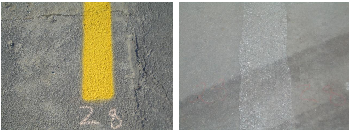
Figure 6.11. Asphalt pavement condition before (left) and after (right) paint has been removed by grinding
