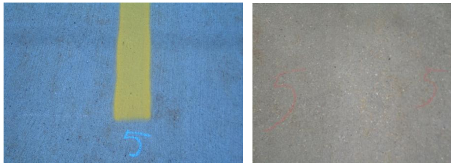
Figure 6.18. Concrete pavement condition before (left) and after (right) paint has been removed by chemicals
