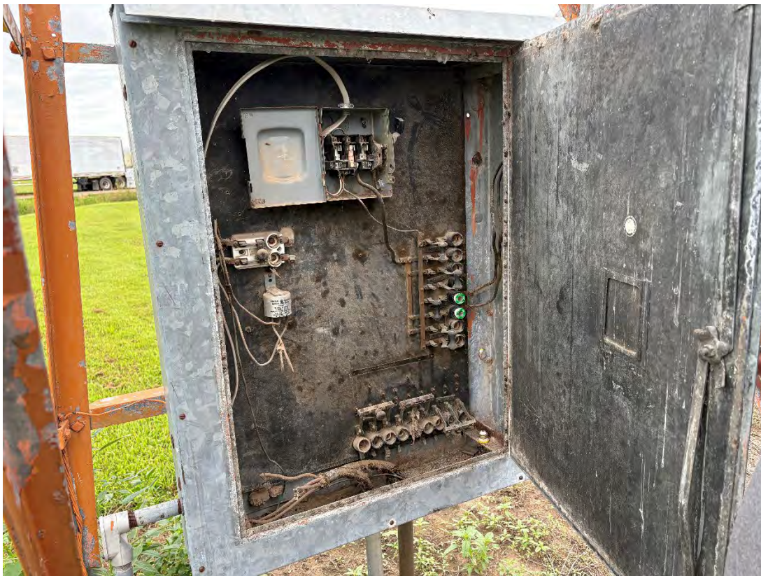
Existing beacon panel.
