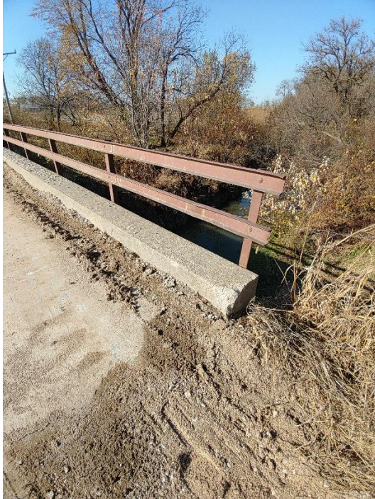
Figure 7: Guardrail does not meet standards
