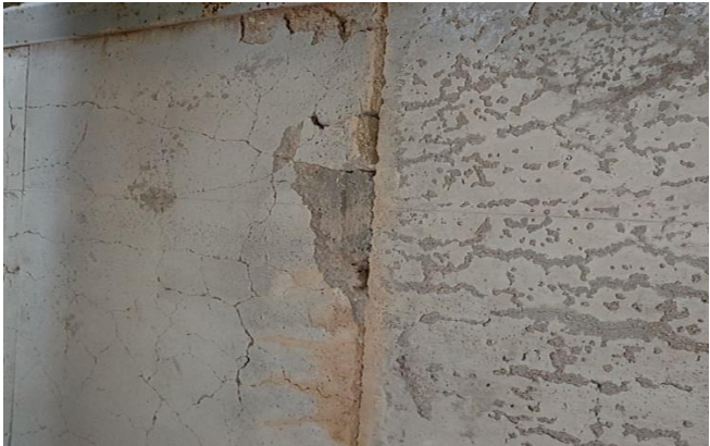
Figure 4: Concrete spalling on underside of deck
