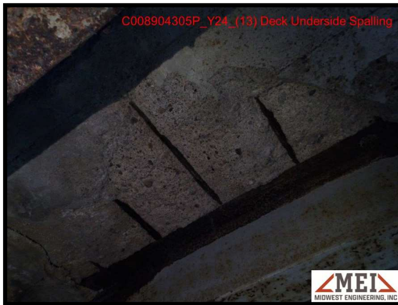
Photo 3: 2024 Deck Spalling at Underside With Exposed Rebar
