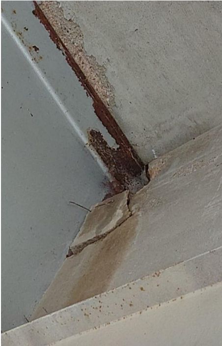
Figure 5: Spalling at Abutment 2
