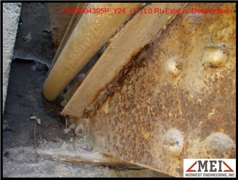
Photo 5: Gusset Plate Deterioration at Bearings
