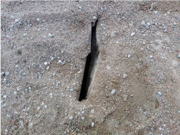
Figure 3: Bridge Deck Separation
