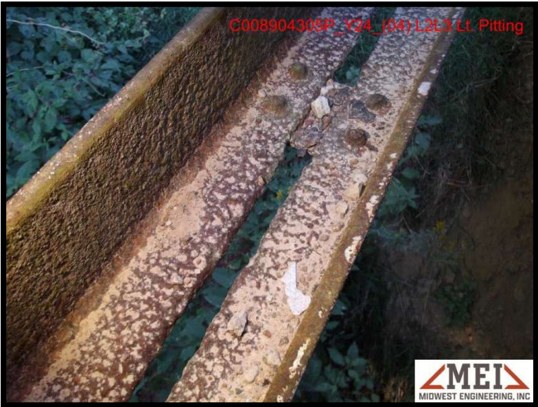
Photo 4: Lower Chord Deterioration
