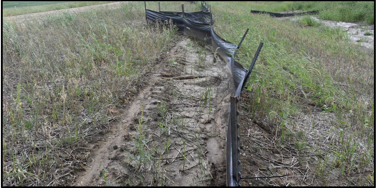
(a) Iowa standard silt fence installation experiencing excessive post deflection
