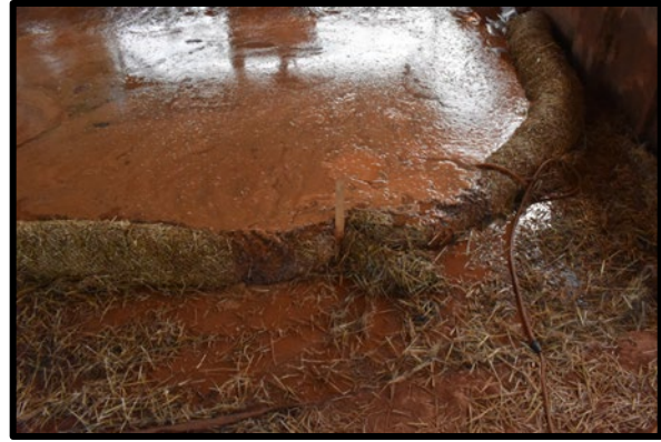
(b) overtopping of installation
