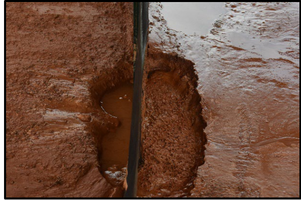
(b) trench failure
