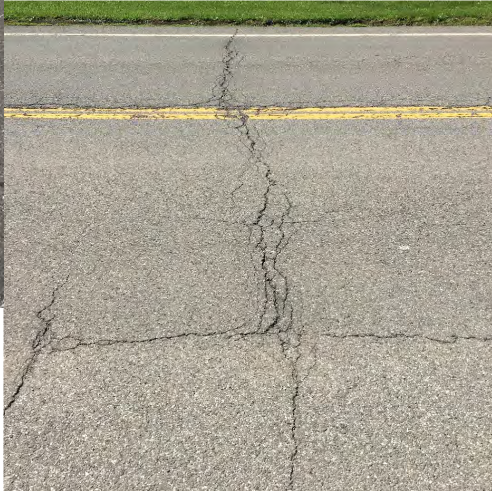
Crack Severity Too High
