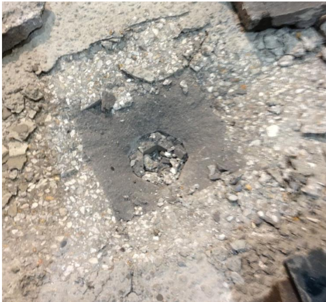
Figure 5.24: Pullout failure mode
