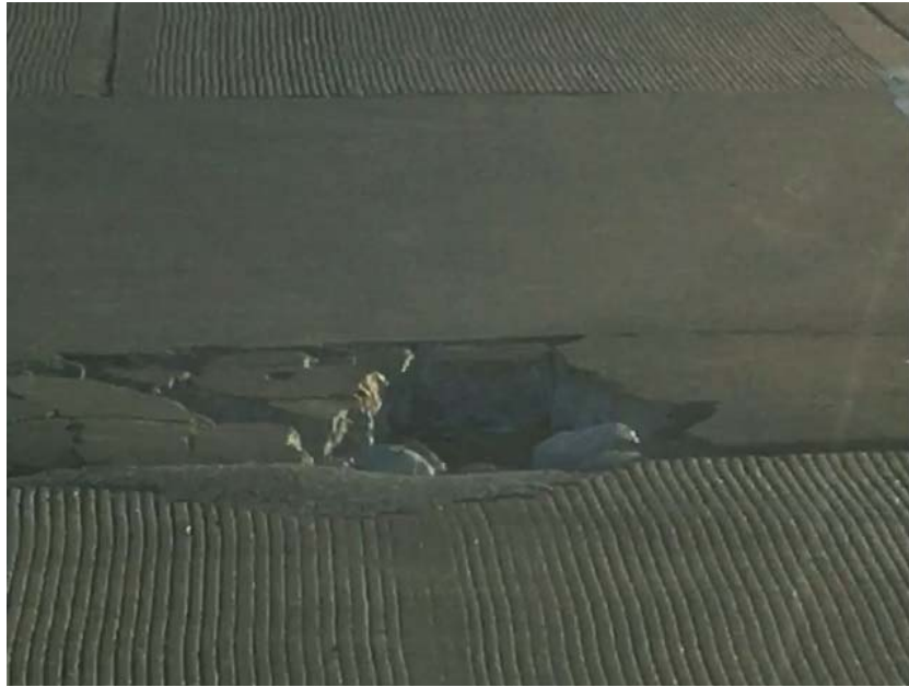
Figure 1-1. Example of premature failure of patching material
