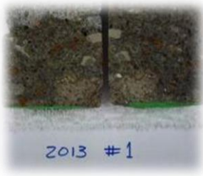
Sealer Penetration Not Visible
