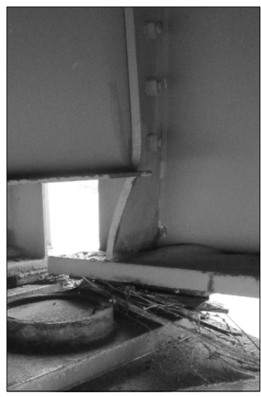
BENT STIFFENER GIRDER D @ PIER NO. 6 BACK
