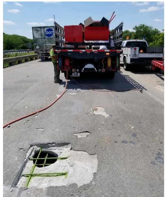
Figure 8 - Bridge Deck Failure Example
