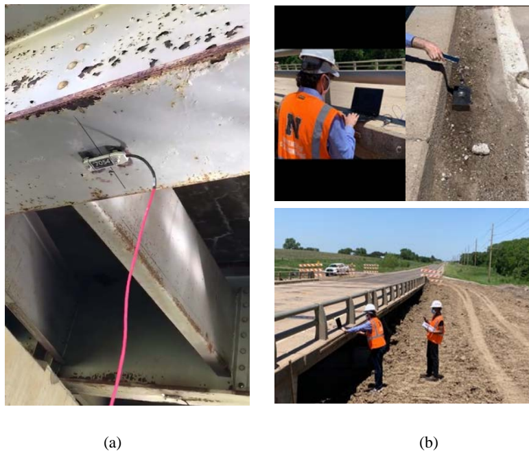
Figure 13: Static and dynamic testing details, Fairbury Bridge: (a) strain transducers on stringer bottom flange; (b) dynamic test using an iPhone 7+.
