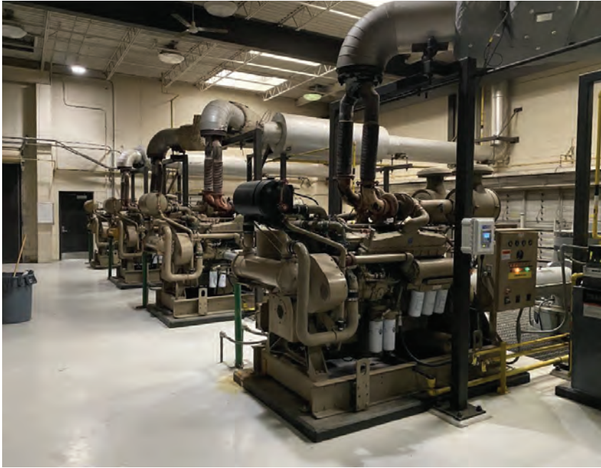
Existing 1984 Diesel Engines at end of useful life in Locust Street Pump Station
