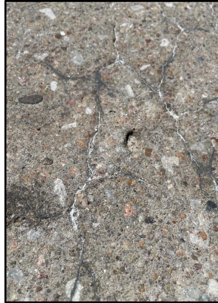
Alkali-Silica Gel in Cracks
