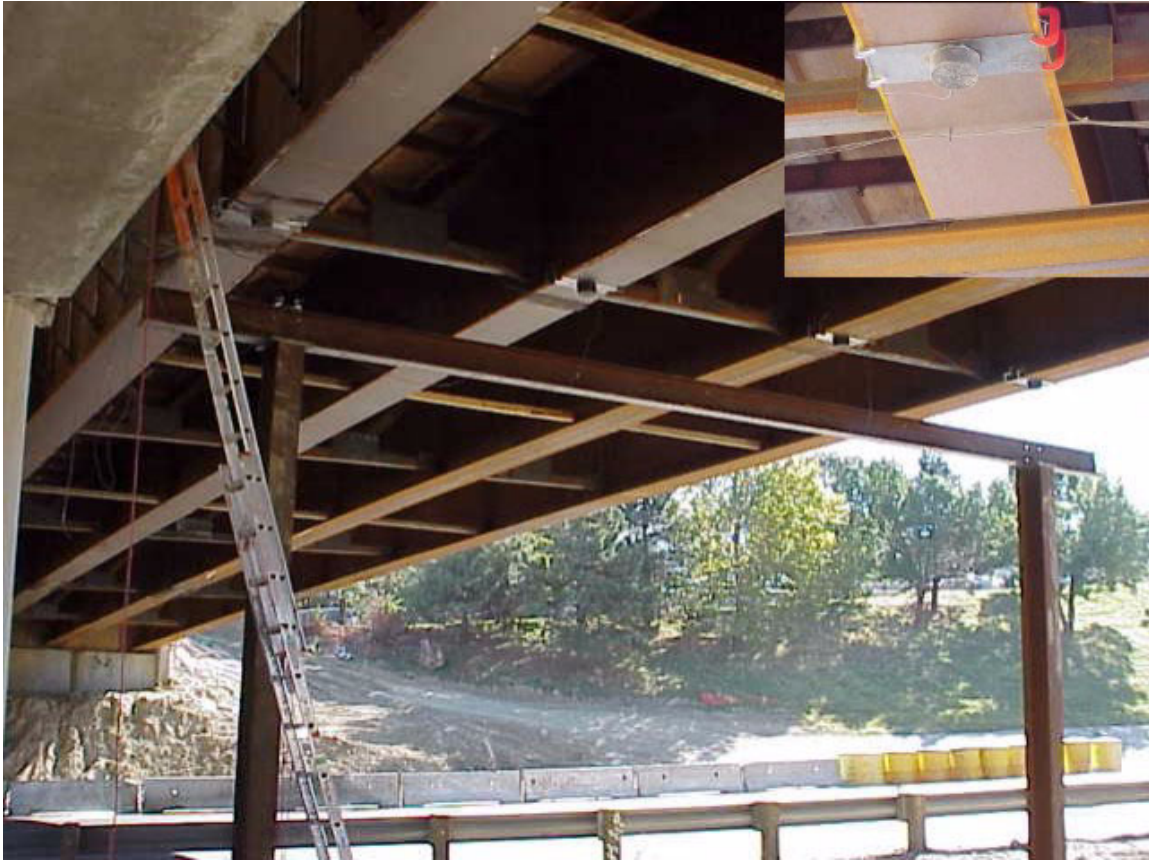
Figure A-15: Test frame used to measure deflection. Note pots mounted on the underside of girders
