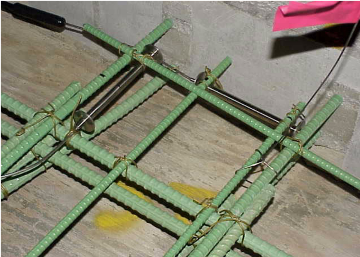
Figure 3-34: Concrete Embedment gage in place. These gages record concrete strain.
