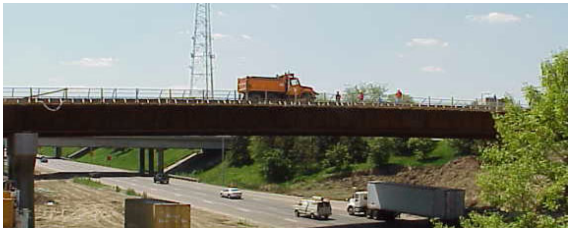
Figure C-2: Southward view of Phase II lane A live load test. The truck is stopped at a predetermined location. The pier can be seen at the left side and the West abutment is on the right
