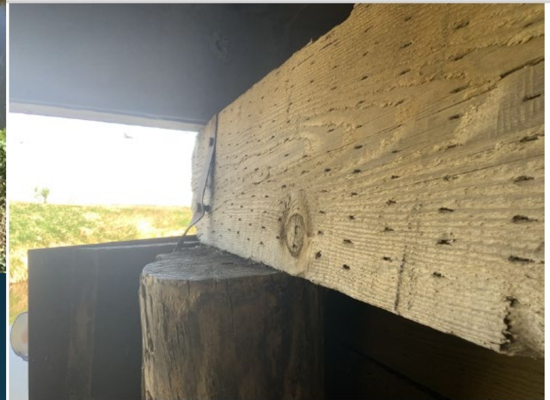
Split, Piles 1 and 2 of the east abutment only bearing approximately 20%
