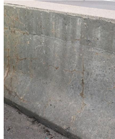
Figure 1 - Concrete median barriers along I-80, I-480, and I-680 showed ASR deterioration.
