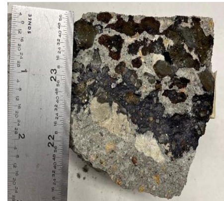
Figure 6 - The power washed section core after sealer was applied.
