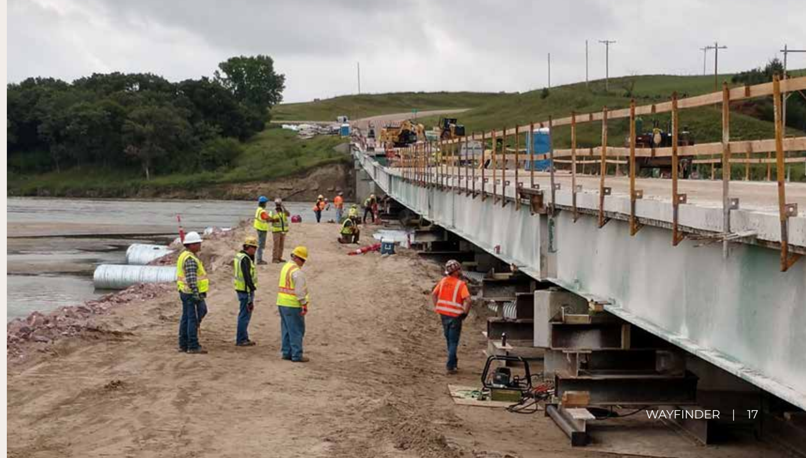
Kiewit using three teams working together to move the N-11 bridge back to the original location. Photo by Greg Henrikson, NDOT District 8
