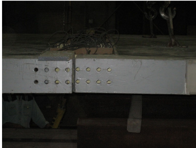
Figure 75 Anchorage plate at the crown location.
