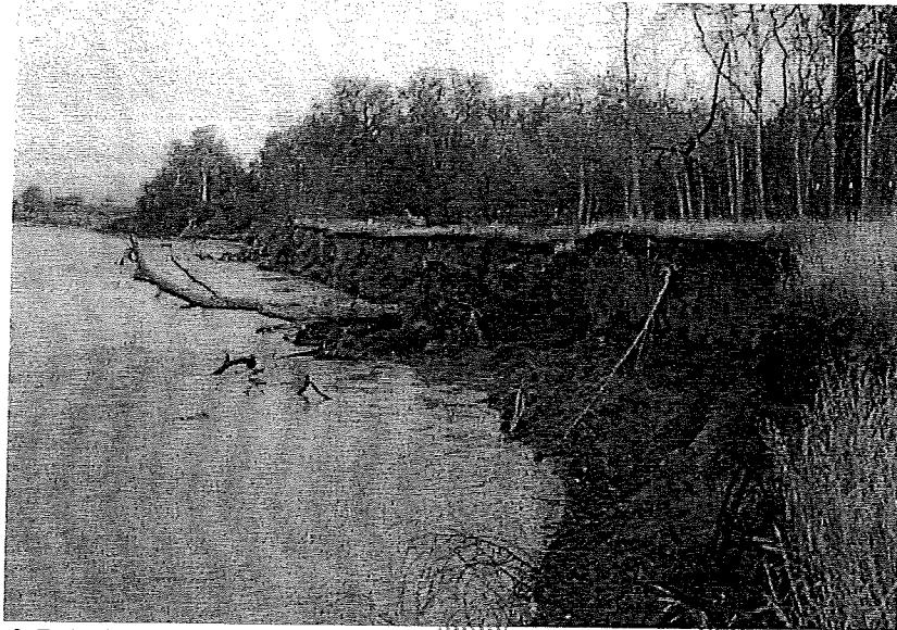
Figure 2.7 Active bank erosion showing vertical bank cuts and falling vegetation (Lagasse et al. 2012)
