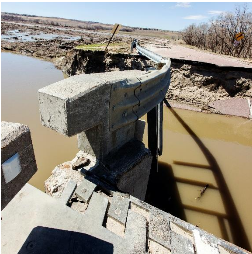
Figure 4-5: Highway 12 Mormon Canal Bridge Washout
