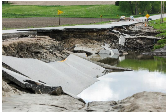
Figure 4-4: Highway 91 Flood Damage
