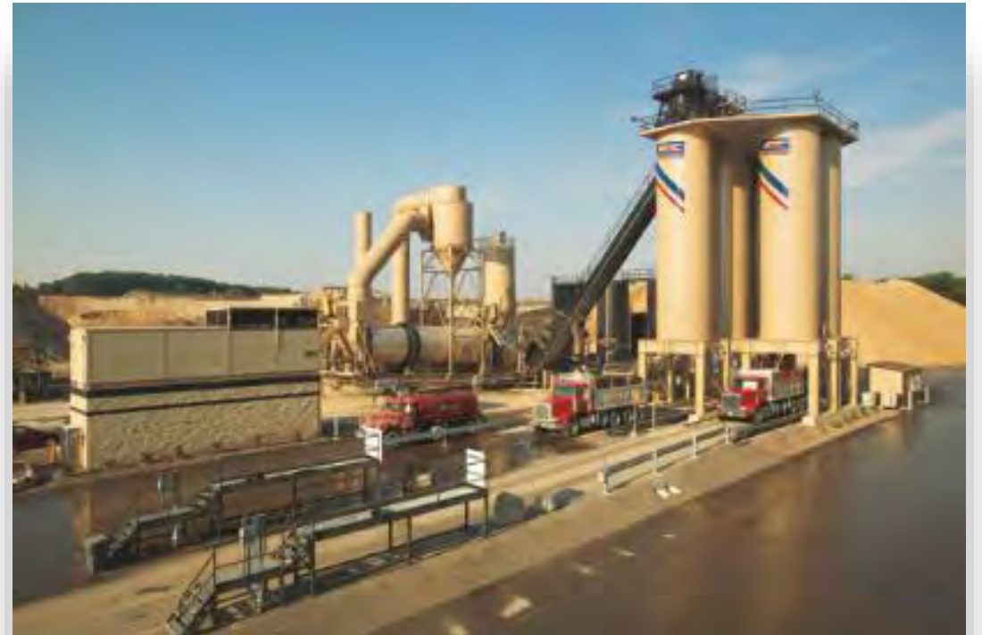
Continuous Flow or Drum Mix Plant
