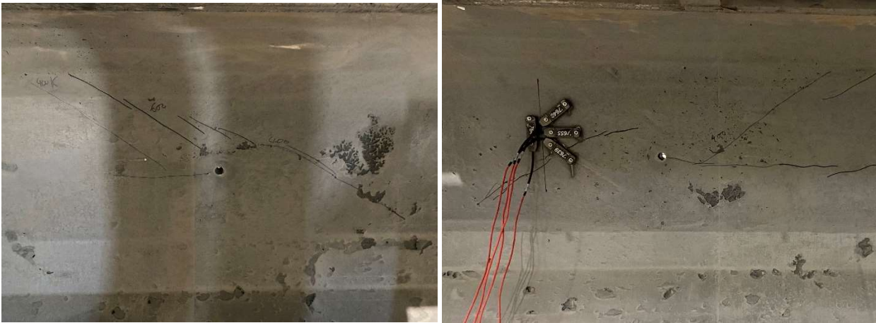
Figure 5.24: Diagonal tension cracks at both girder sides
