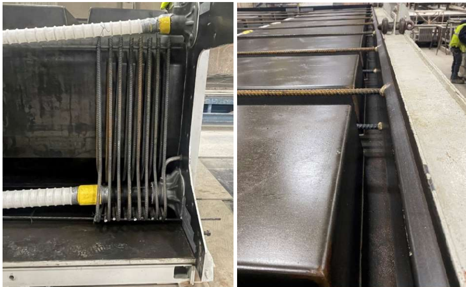
Figure 4.14: End zone reinforcement for PT specimen (left) and edge form with lip (right)
