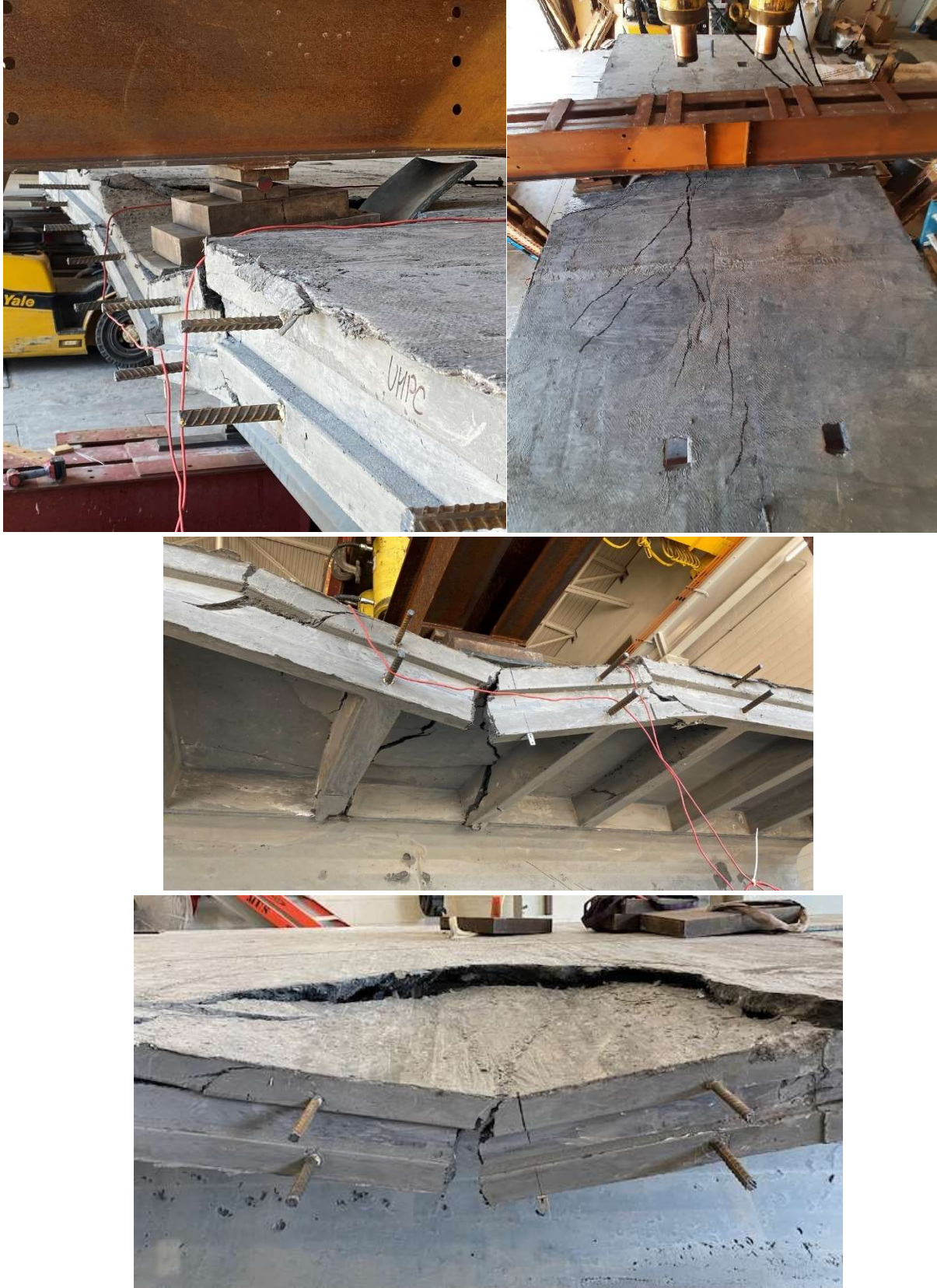
Figure 5.30: Ribbed slab overhang failure by punching shear
