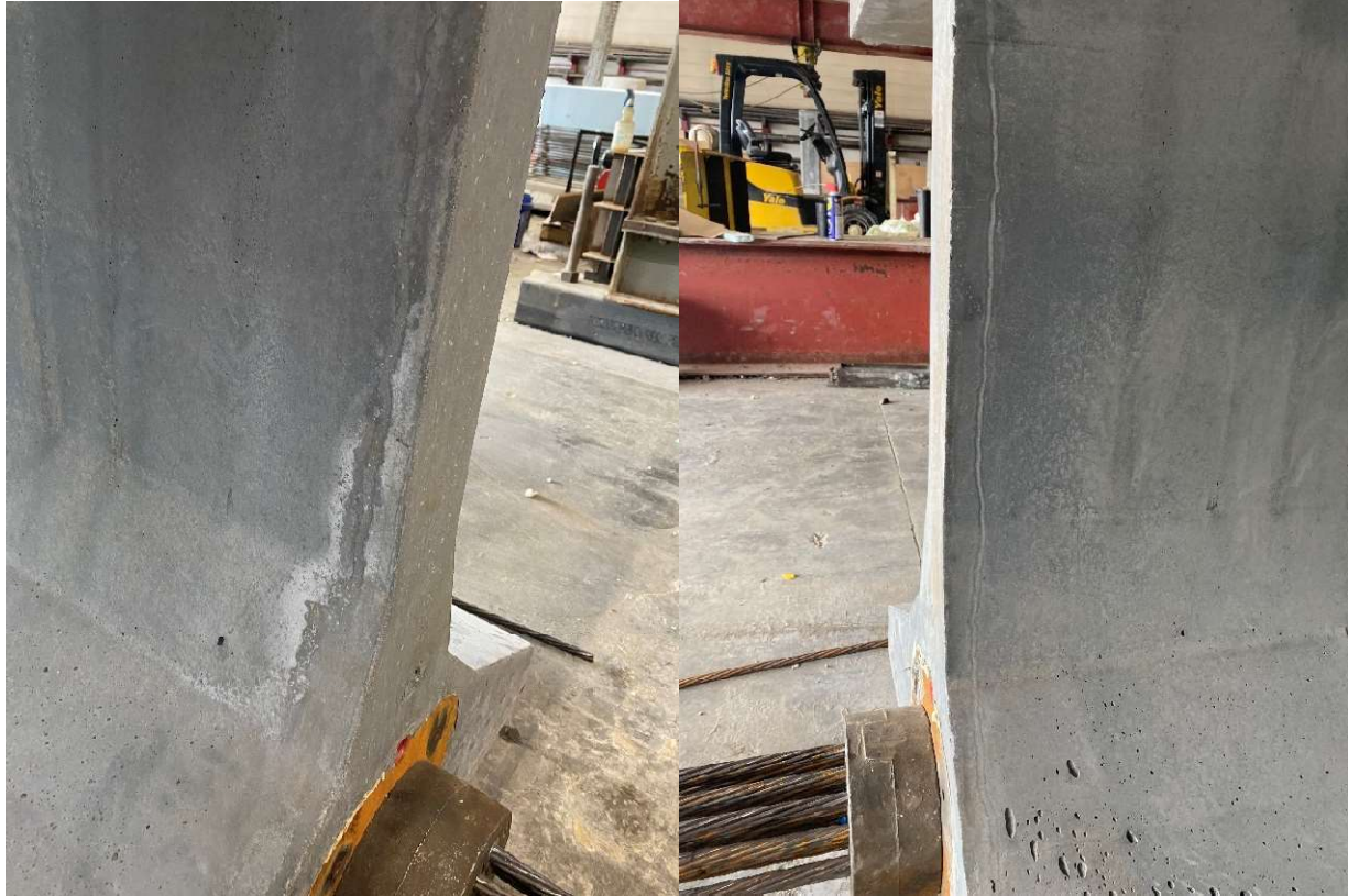
Figure 5.40: Specimen ends after post-tensioning showing no cracking
