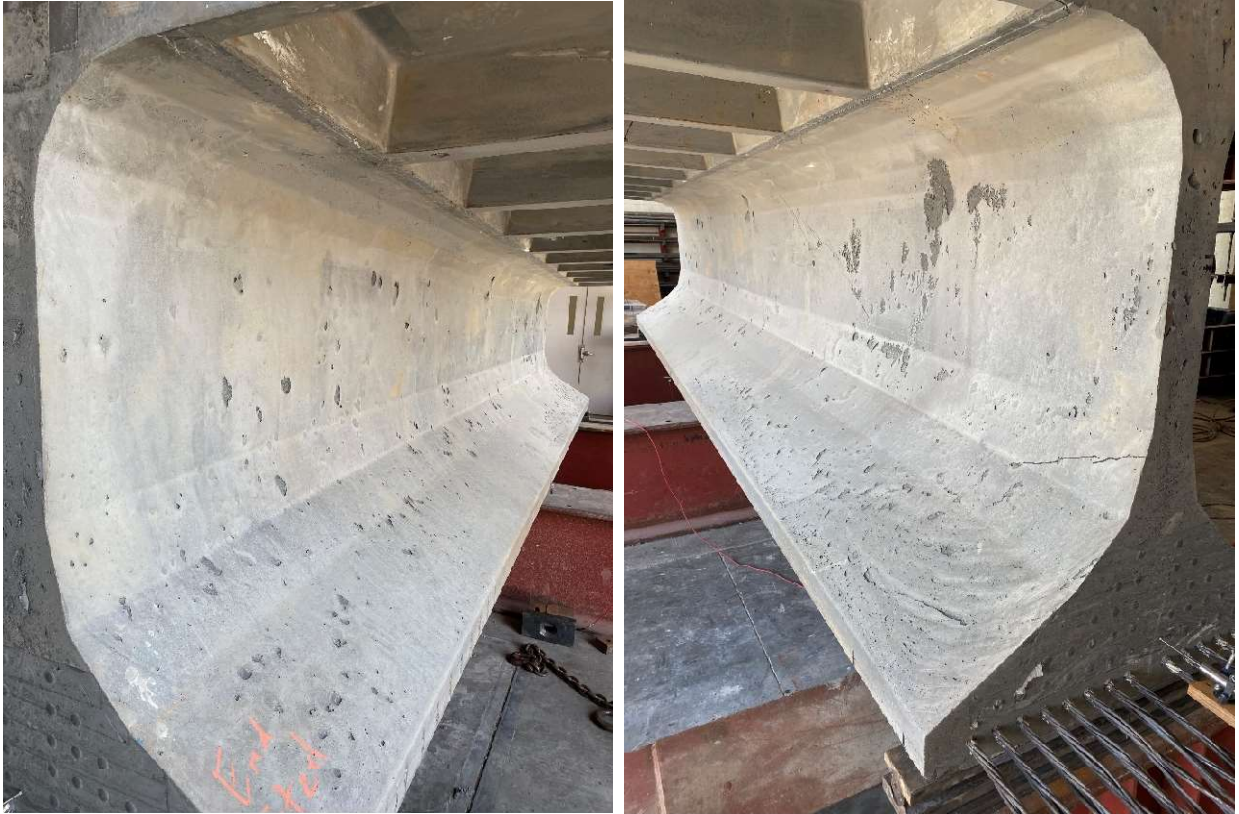
Figure 5.25: End zone cracking at both girder ends
