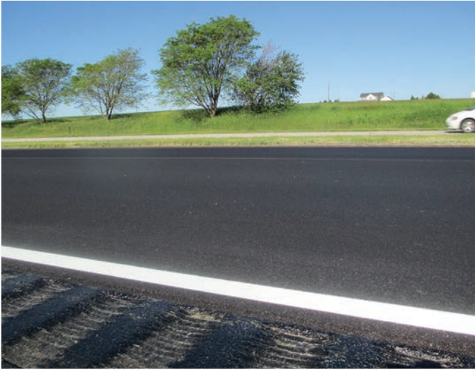
Five years later, the first 1-inch thin-lift overlay pavement using SLX mix, built on US-77 – Lincoln South, is performing well.
