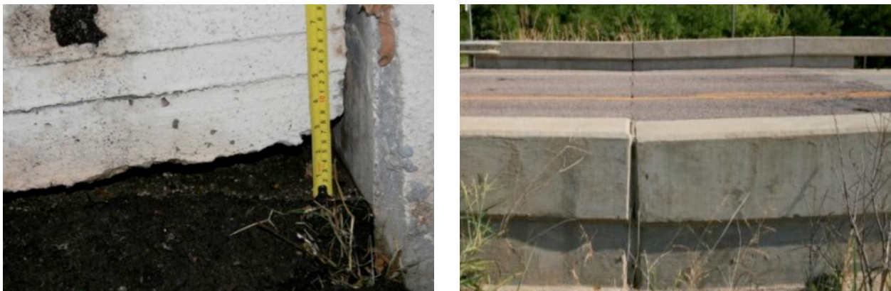
Figure 2.15 Some examples of the differential settlement problems encountered in the approach slabs in Oklahoma (after Miller et al., 2013).
