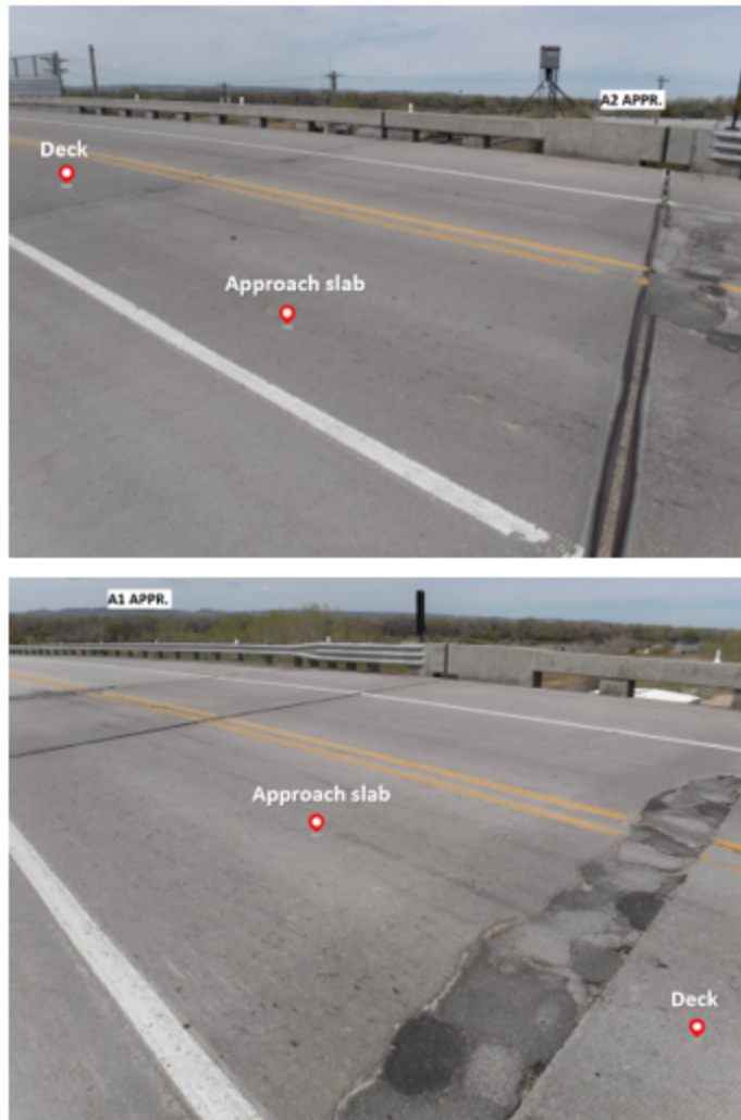
Figure 2.9 An example of minor problems encountered in the approach slab with the new design in Nebraska.
