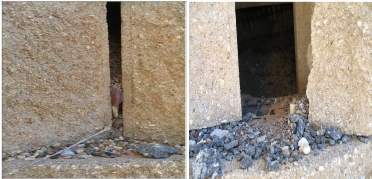
Figure 2.17 A modular block failure and erosion in the embankment fill under the approach slab. (after Puppala et al., 2012).
