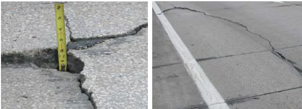
Figure 2.20 An example of problems encountered in the approach slabs in Kansas (Thiagarajan and Gopalarathnam, 2010).
