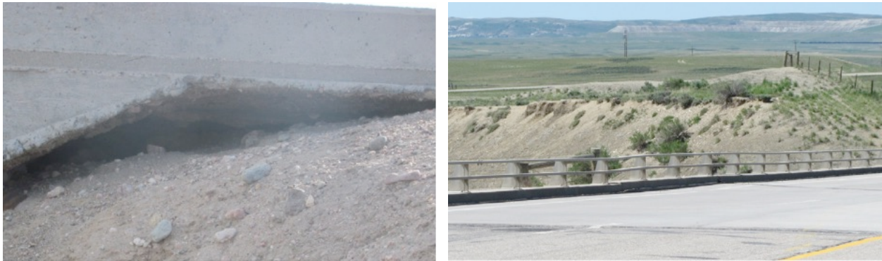
Figure 2.22 An example of problems encountered in the approach slab in Wyoming (Ng et al., 2015).
