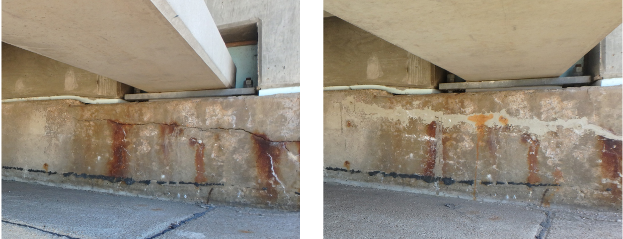
Figure 7.38—Epoxy Crack Injection (Before on the Left, and After on the Right)
