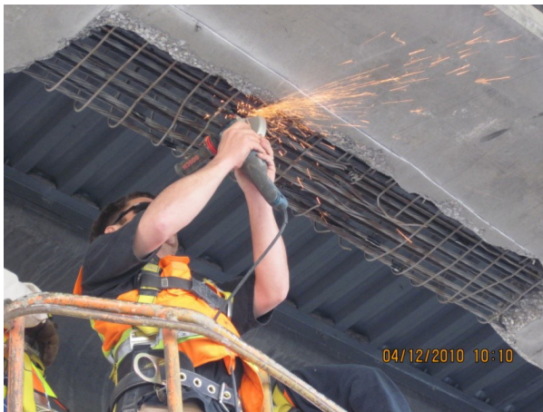
C. Cutting Damaged Strands
