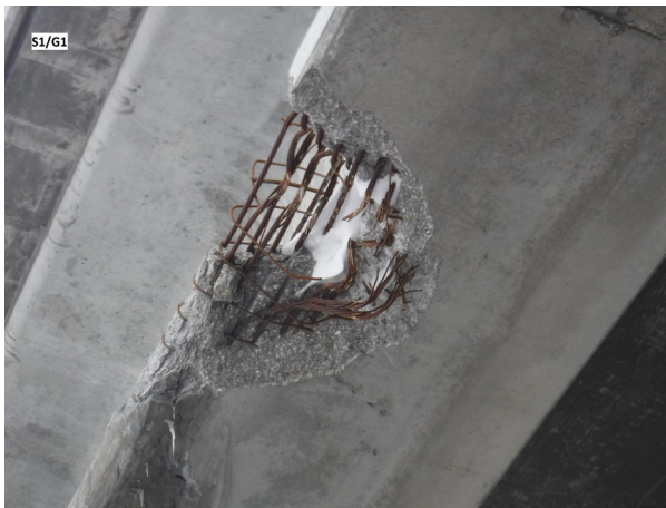
A. Strand Impact Damage
