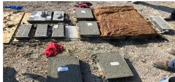
Figure 5 - Mini-prisms and ponding blocks, field curing. Half of the samples were exposed to ambient conditions, while the other half were cured according to NDOT standards.
