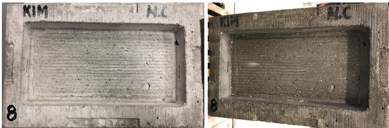
Figure 19- B8 before testing (left) and after testing showed light sign of scaling after 85 F-T cycles.
