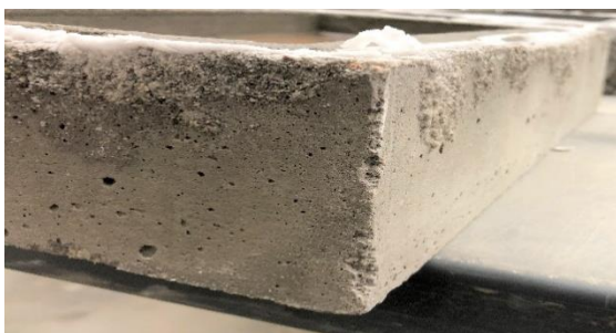
Figure 12 - The concrete blistered where NaCl deposits were.
