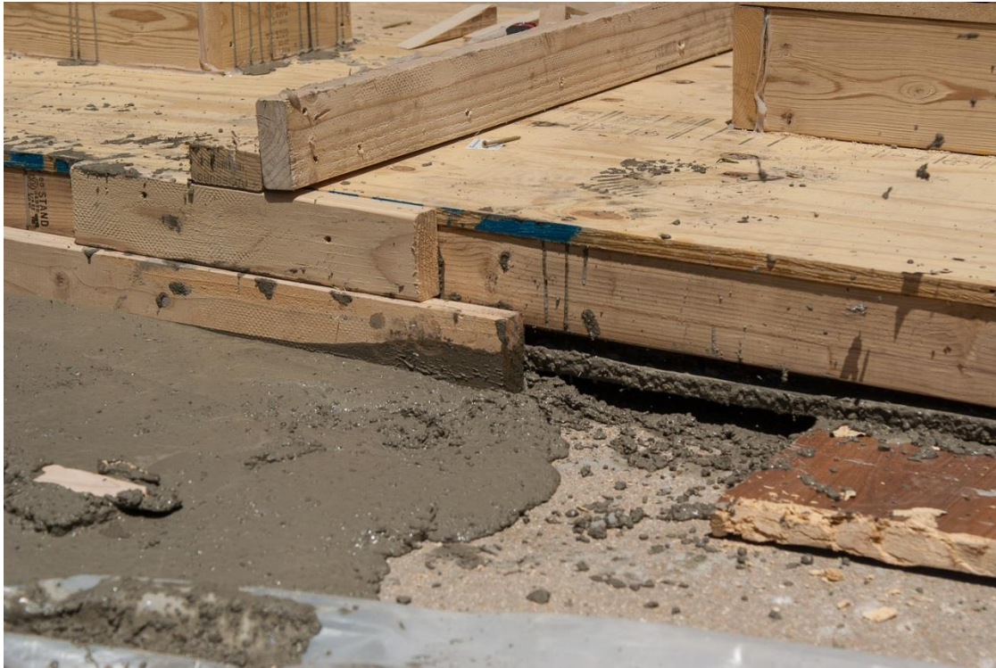
Figure 2.3 – Leakage of concrete after formwork failure due to high concrete pressure at one end
