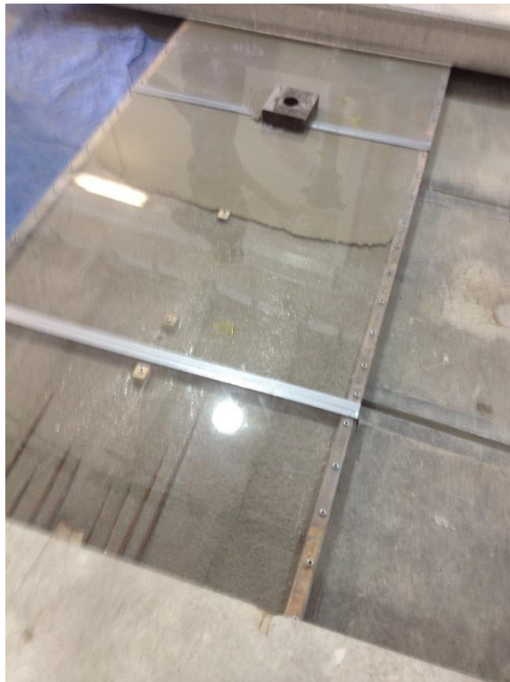
Figure 3.6 – SCC flowing from one port to the other and completely filling the channel
