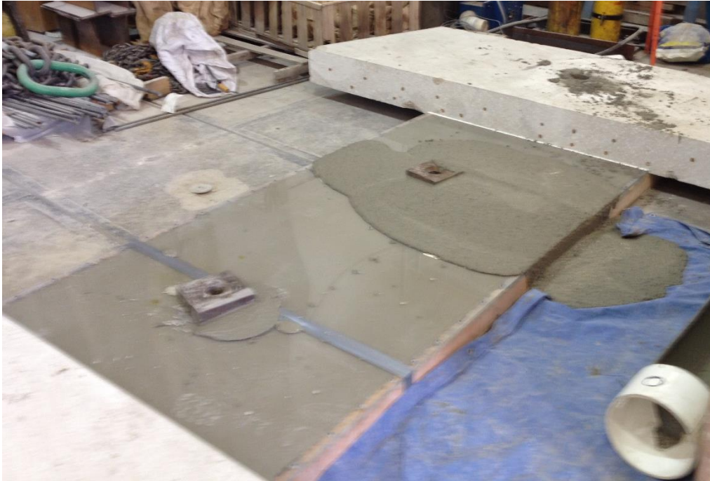
Figure 3.7 – Concrete overflowing at one of the joints between Plexiglass sheets
