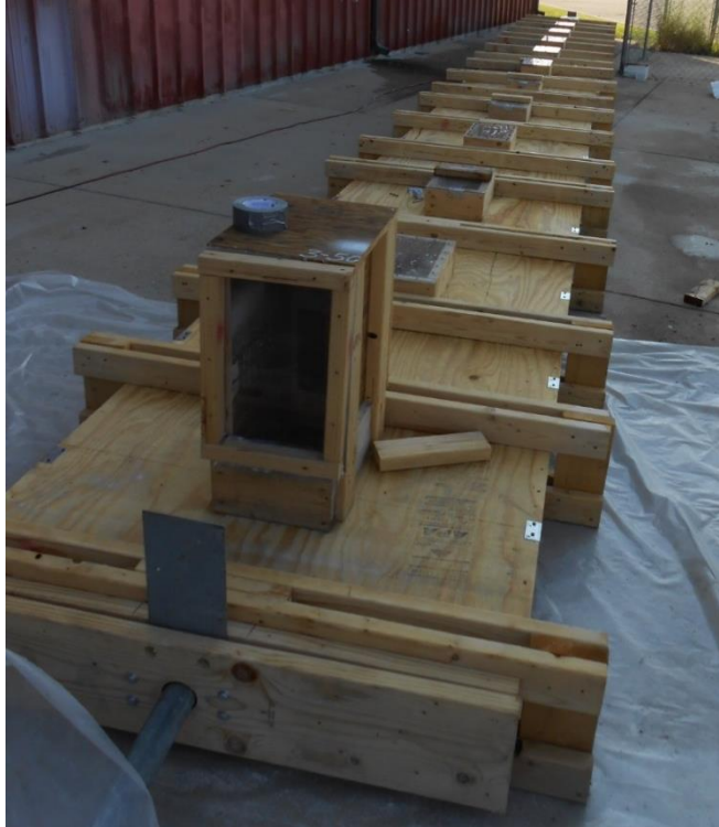
Figure 2.5 – Photo of the formwork, pump connection, and pressure indicator at one end
