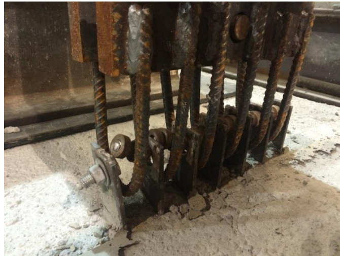
Figure 4.13: Rupture of the threaded rod
