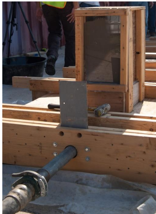
Figure 2.8 – Pumping line connected to the one end of the formwork and concrete pressure indicator tower to monitor pressure build-up exerted on the formwork
