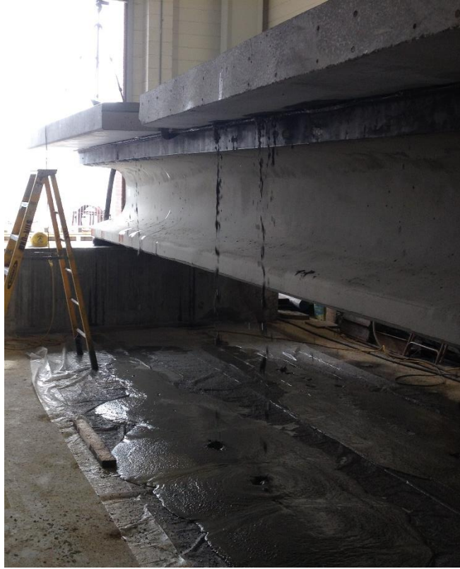
Figure 2.26 – Concrete leakage during pumping due to deck uplift
