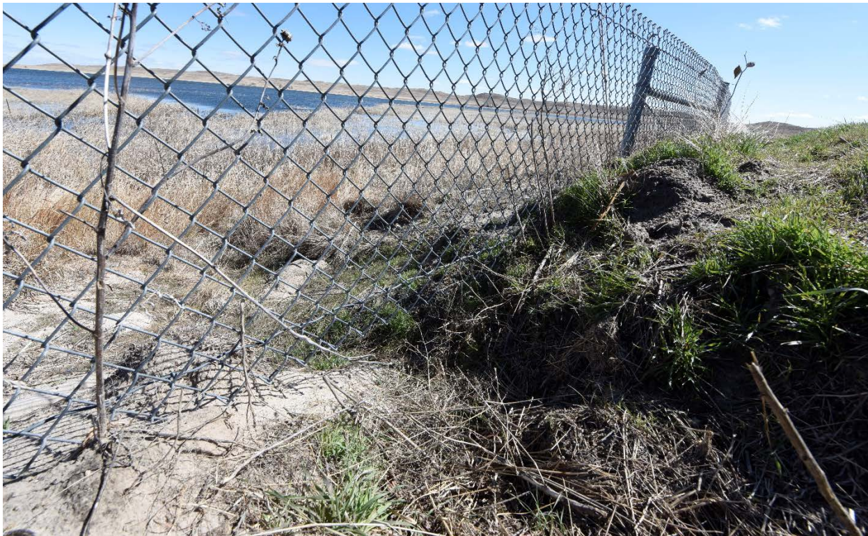
Figure 10: Gaps under the fence caused by erosion (Twin Lakes), April 2016.
