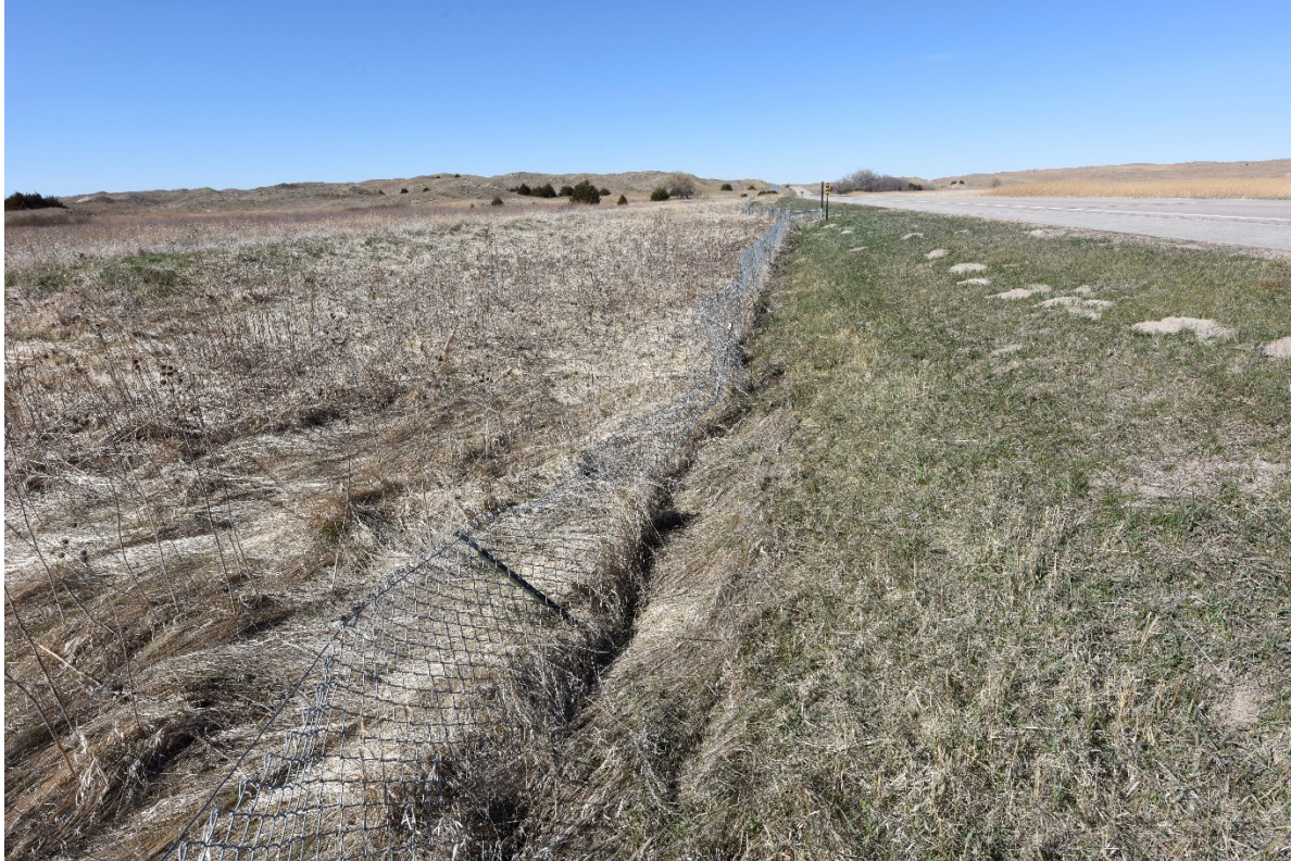
Figure 8: The turtle fence has broken posts because a vehicle ran off the highway (Ballard's Marsh), April 2016.
