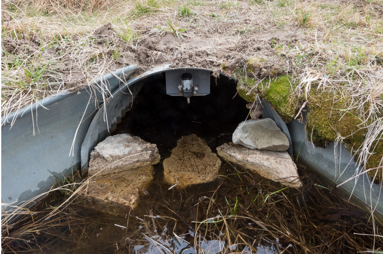
Figure 12: Turtle ramp made from concrete debris forced the turtles directly under the cameras and to the water surface (Pony Lake). Note that this culvert is not connected to a turtle fence.
