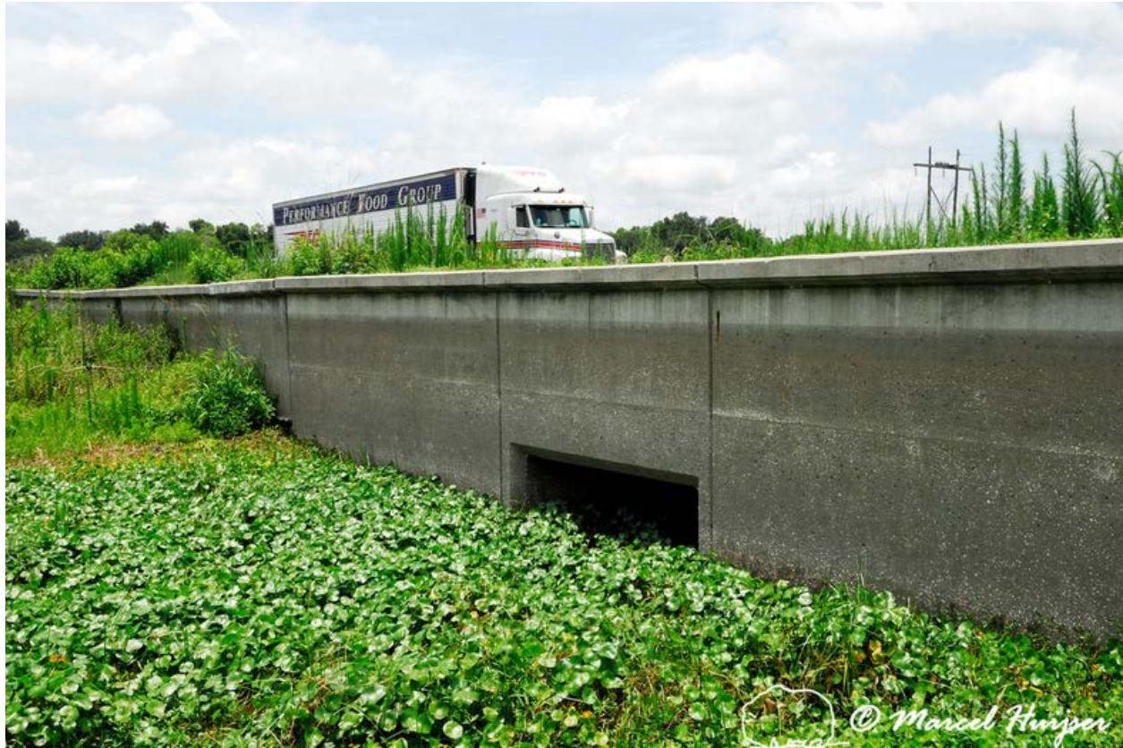
Figure 22: Underpass and barrier wall for reptiles, amphibians and small mammals, U.S. 441, Paynes Prairie Ecopassage, south of Gainesville, Florida, USA.
