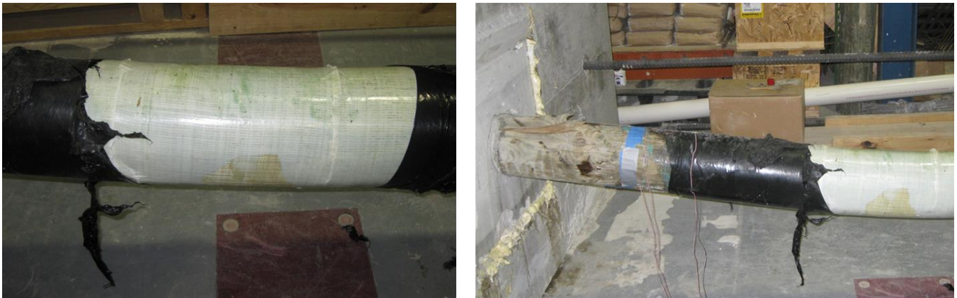
Figure 5.8: Failure of specimen 2 (1.5 inch deep damage filled with resin)
