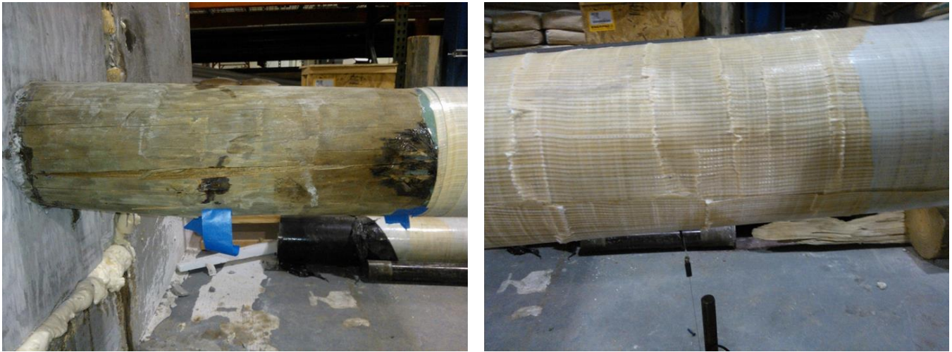
Figure 5.7: Failure of specimen 1 (1 inch deep damage filled with resin)
