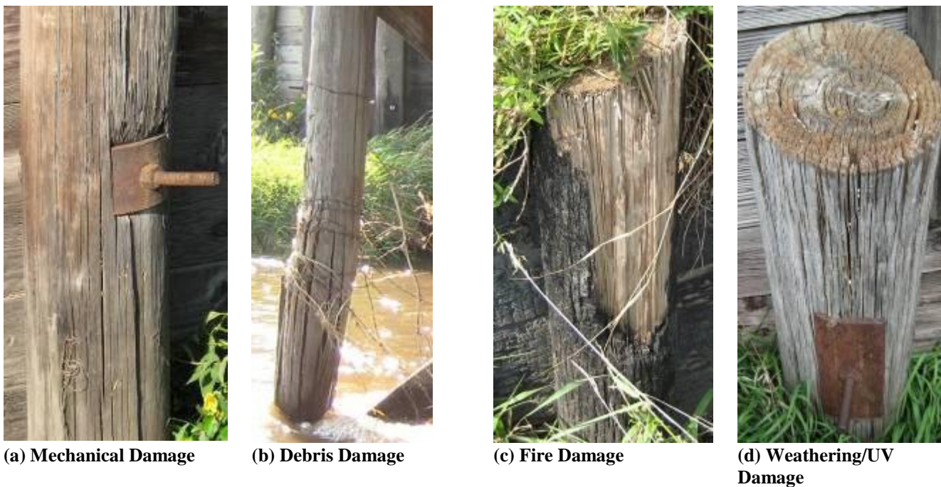
Figure 2.1 Breaks in preservative barriers by exterior damage leads to premature decay [2]
