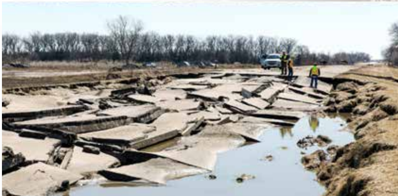
Damage from 2019 flooding in Nebraska.
