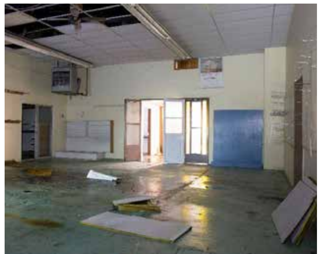
The building was in disrepair and sustained structural damage due to a leaky roof. Photo Credit: Kimball Co. Transit
