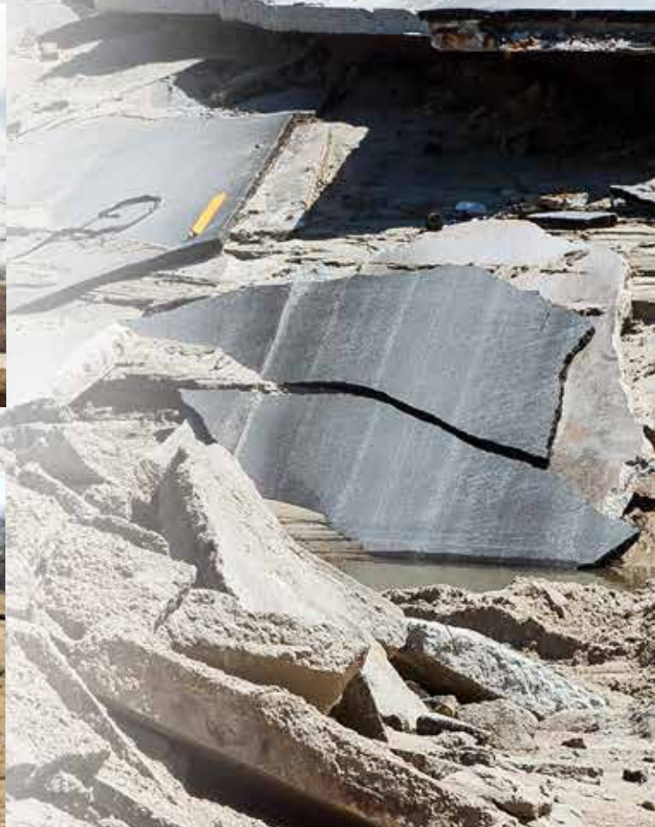
Damage from 2019 flooding in Nebraska on Highway 30.
