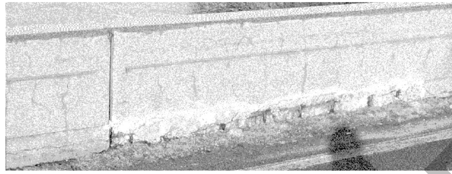
C2 Repair bottom of Curb as required
