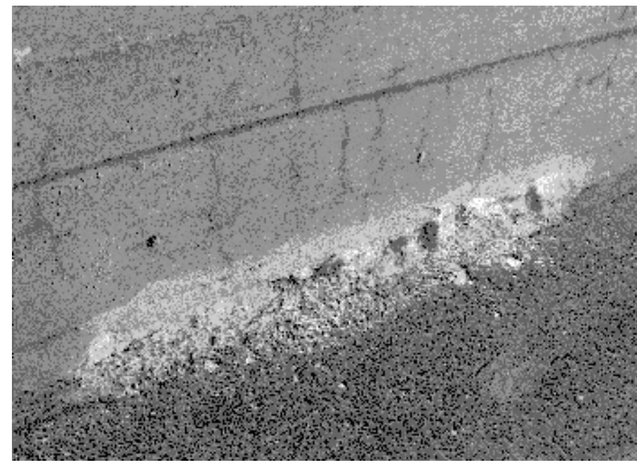
C1 Repair bottom of Curb as required
