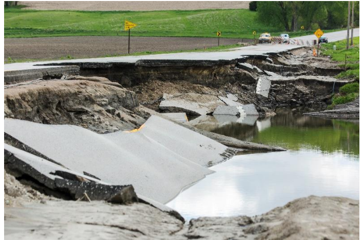
Figure 4-4: Highway 91 Flood Damage
