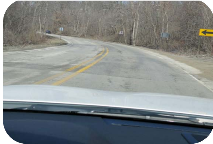
Manual Visual Ratings (Cracking Distress)
