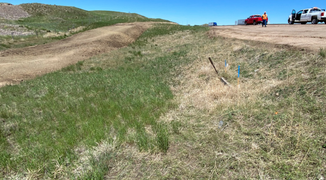
Pictured: Good example of a soil berm used for perimeter control.
