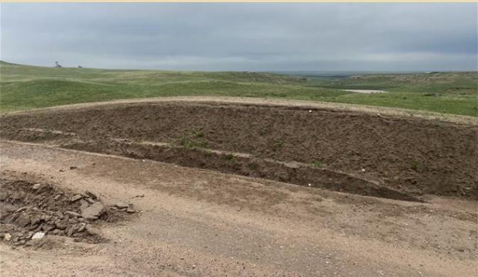
Pictured: Poor example of stockpile management. Protect stockpiles with silt fence or other BMPs and seed if left undisturbed for more than 14 days.
