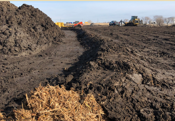
Pictured: Good use of soil berm around stockpile. The soil berm is being mulched and at least 6 feet from toe of pile. Stockpiles must be stabilized if left undisturbed for more than 14 days.
