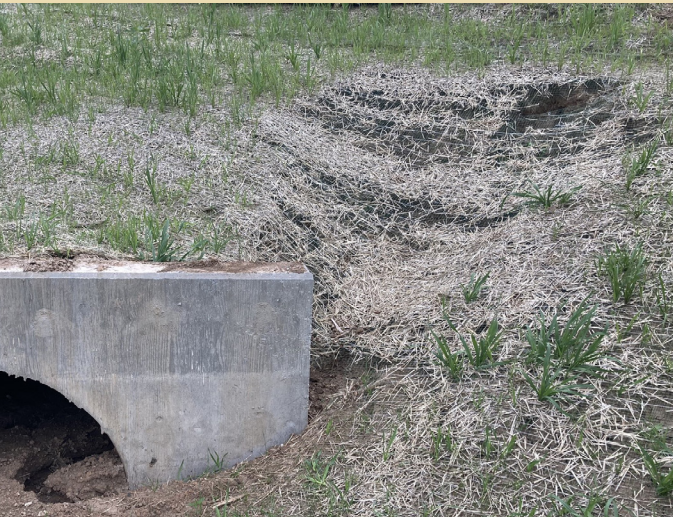
Pictured: Example of gully erosion from poor installation.
