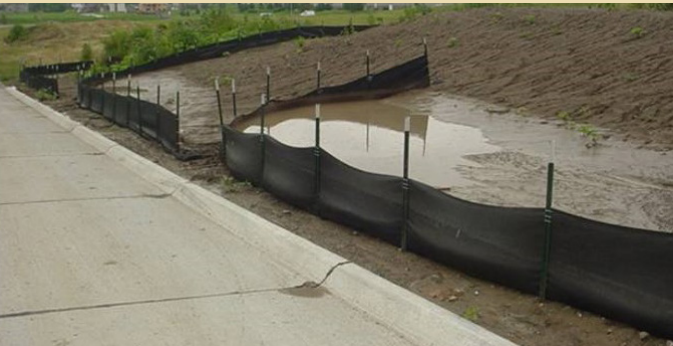
Pictured: The ponding created with this installation allows sediment to settle and be deposited.
