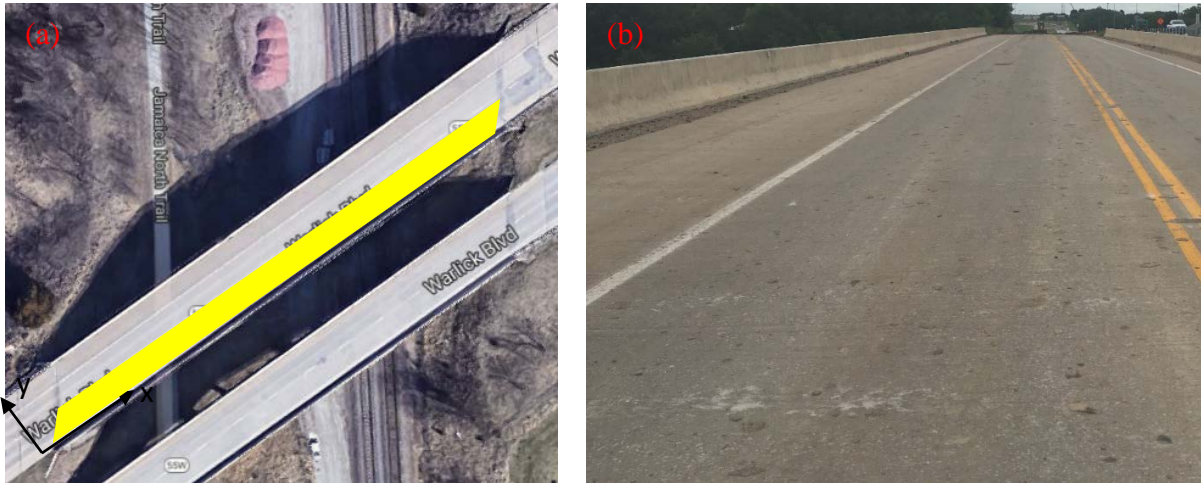
Figure 5-13 Bridge 1 (left lane): (a) Google map and the scanned area in 2017, (b) Deck surface conditions
