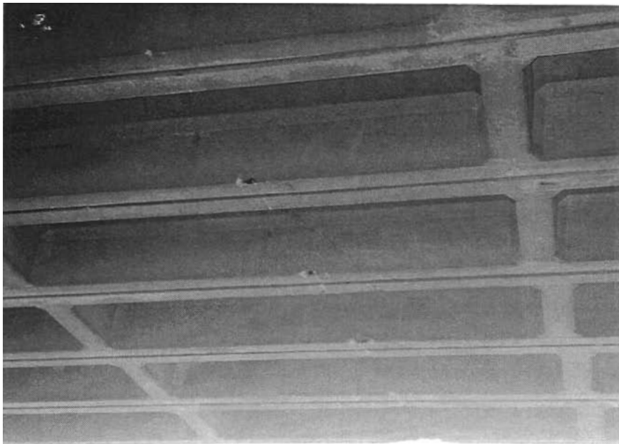
Figure 1: Minor damage, courtesy of Feldman et al., 1996
