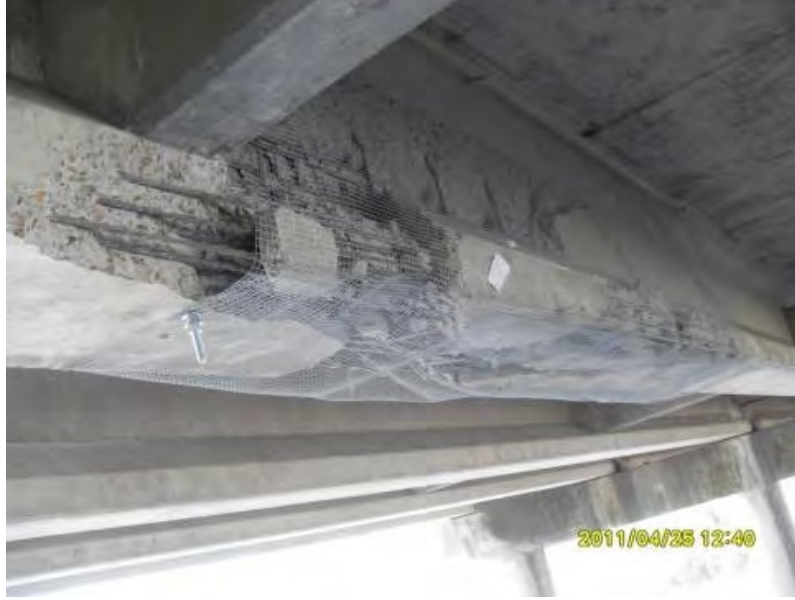
Figure 8: AASHTO I-girder; reportedly repaired, courtesy of Harries et al., 2012
