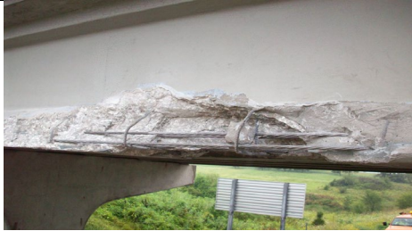
Figure 4: Moderate damage, exposed intact strands, Iowa DOT, 2014
