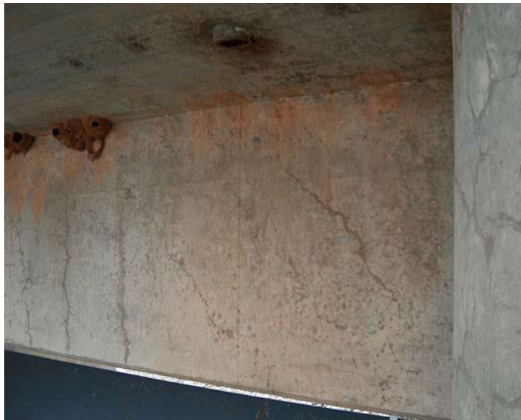
Figure 42: Condition State Fair, cracking on concrete bridge girder, courtesy of WisDOT, 2018
