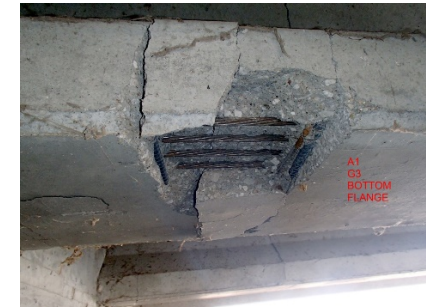
Figure 12: Severe damage, exposed strands, severe cracks or fractures, NDOT Alma South Bridge
