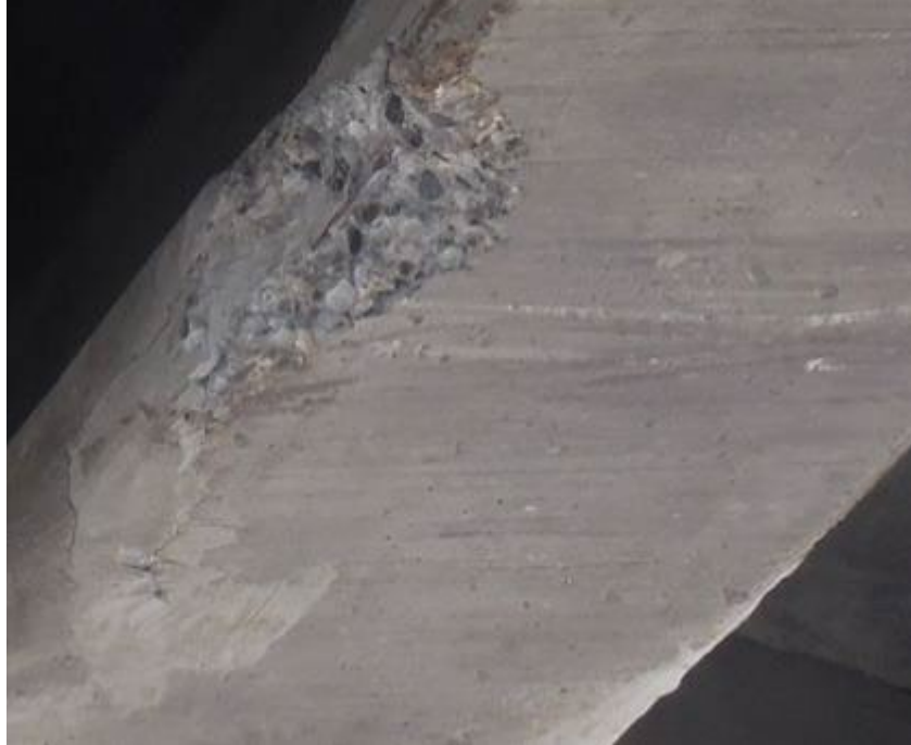
Figure 43: Condition State Fair, exposed strand on concrete bridge girder, courtesy of WisDOT, 2018
