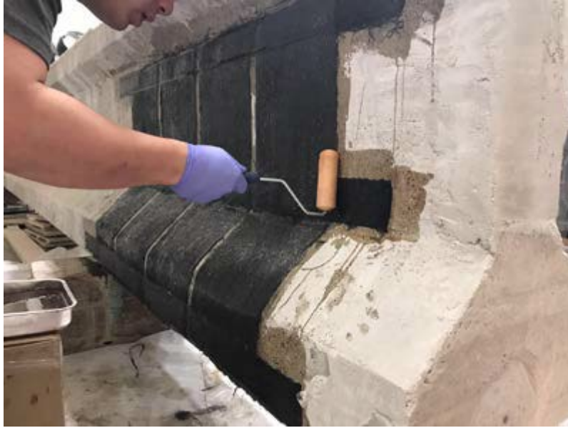
Figure 54: Applying shear CFRP to full-scale prestressed girder end, courtesy of Andrawes et al., 2018
