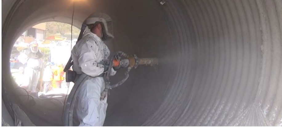
Figure 61: UHPC shotcrete to renovate a deteriorated metal culvert suffering from corrosion damage, obtained from Ductal website
