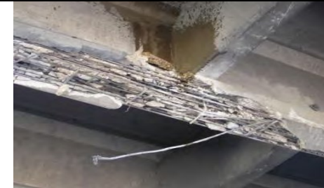
Figure 9: Severe I damage, one severed strand, Harries et al., 2012
