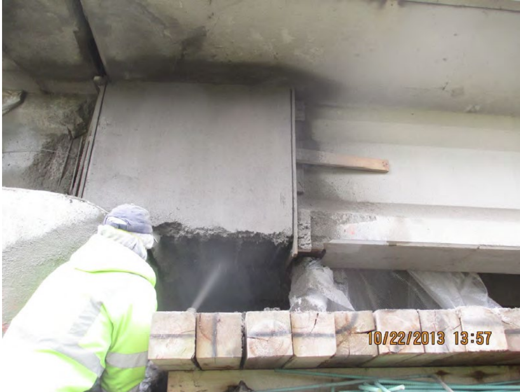
Figure 52: Shotcreting the bottom surface of the repair at girder end, MN/RC 2018-07 Report
