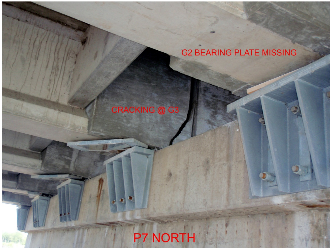
Figure 114: Damage at girder end, Kearney South Platte River Bridge, courtesy of NDOT
