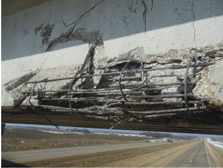
Figure 12: Heavy damage with web cracking and severed mild reinforcing and prestressing strands, courtesy of Iowa DOT, 2014
