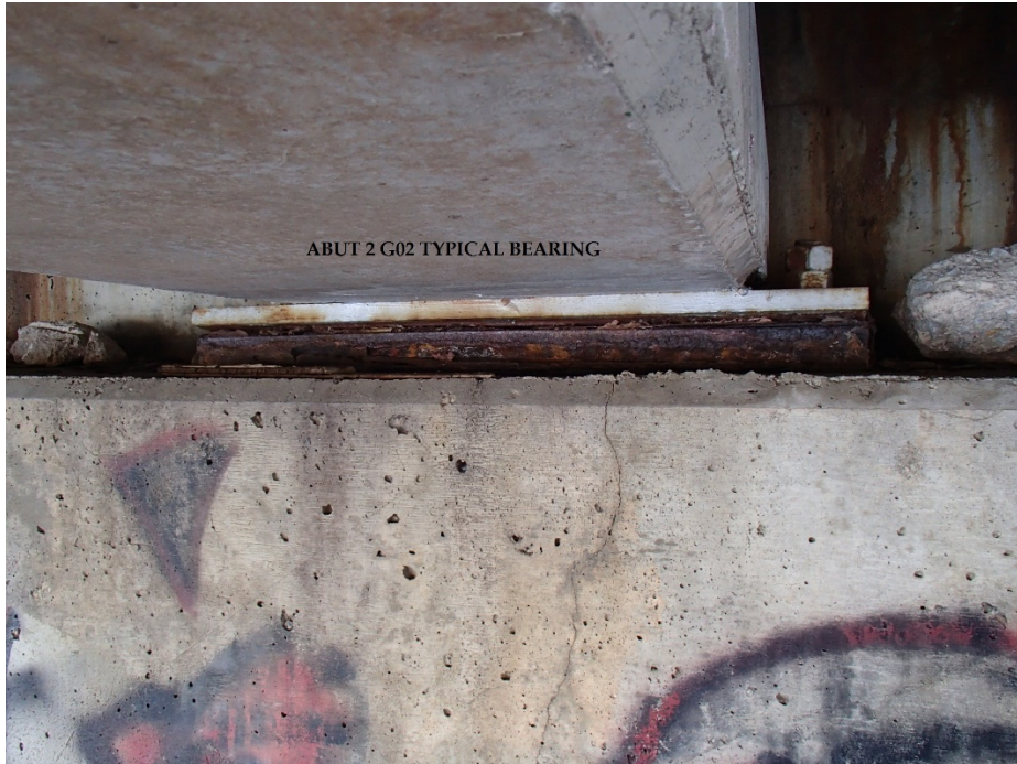
Figure 107: Corrosion damage at bearing assemble, Platte River Bridge East of Grand Island, courtesy of NDOT
