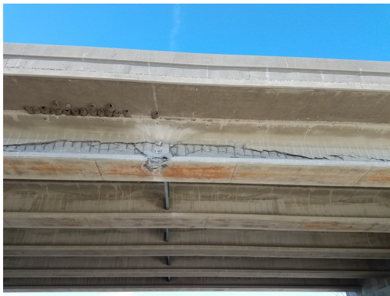
Figure 70: Level of damage, Schuyler Bridge, courtesy of NDOT
