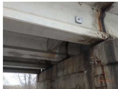
Figure 11: Severe damage, exposed strands, NDOT Platte River South Bridge
