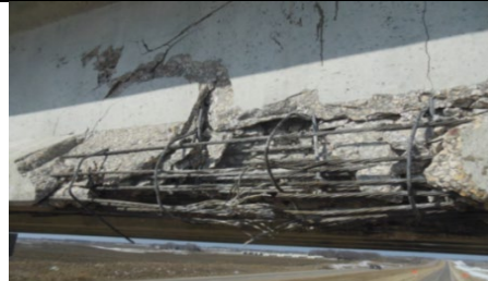
Figure 14: Severe III damage, several damaged strands, Iowa DOT, 2014
