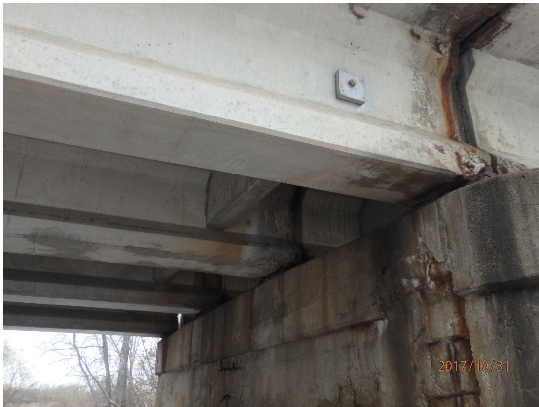
Figure 123: Damage at girder ends, Platte River South Bridge, courtesy of NDOT
