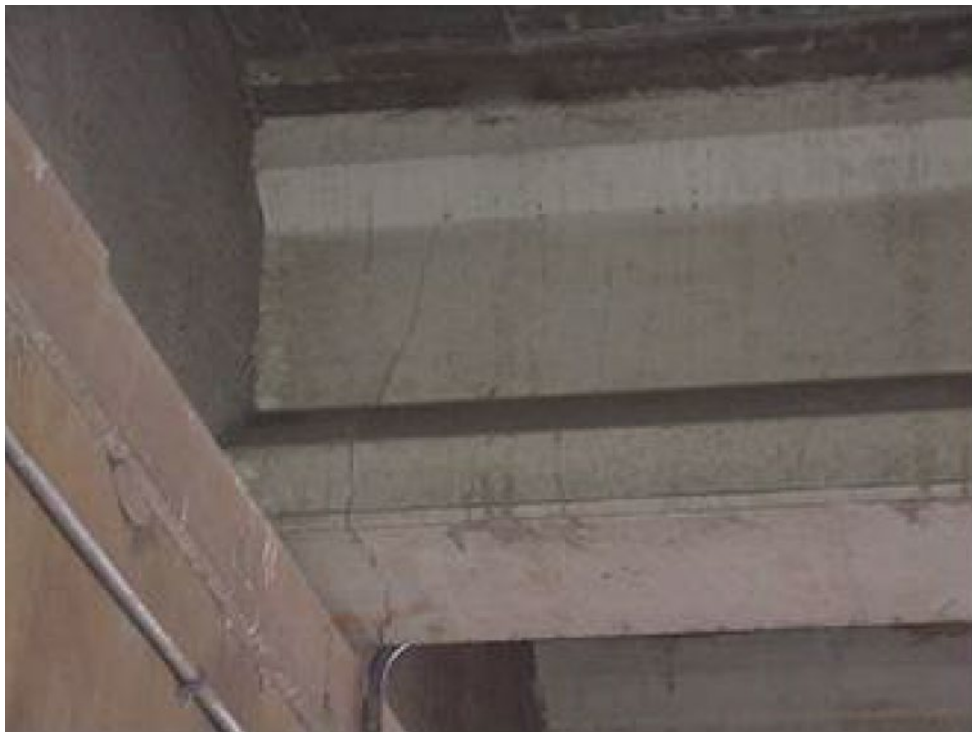
Figure 49: Severe class corrosion damage at girder end causing severe cracks, courtesy of Choo et al., 2013
