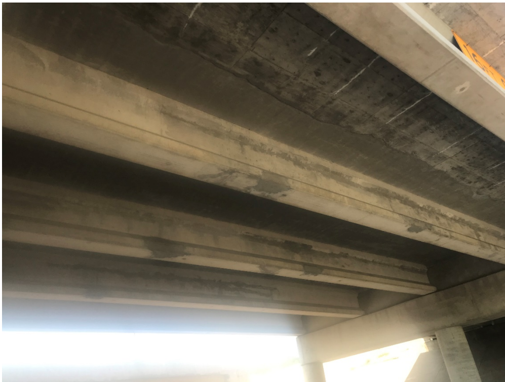
Figure 103: Replaced girder and girders with patching and epoxy injection works, I-680 over US-75 Bridge, courtesy of NDOT
