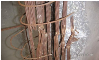
Figure 10: Severe II damage, five severed strands, NDOT Wood River Interchange Bridge Girder (E)
