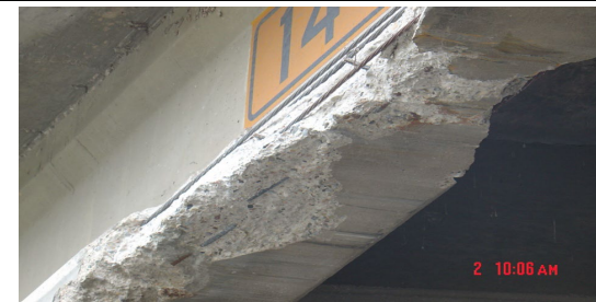
Figure 6: Moderate damage, exposed intact strands, Pantelides et al., 2010
