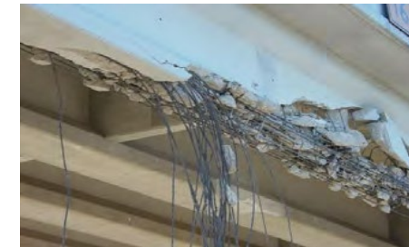
Figure 15: Severe III damage, several damaged strands, Harries et al., 2012
