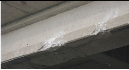
Figure 1: Minor damage, bottom flange spalling, Iowa DOT, 2014
