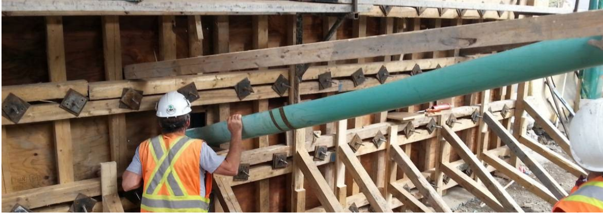
Figure 60: Casting UHPC for a thin jacket for a bridge pier from middle openings in the formwork, CN Rail bridge, Quebec, Canada, obtained from Ductal website
