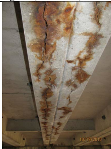
Figure 7: Extensive damage, delamination, and rust staining a precast concrete channel girder, MnDOT, 2019
