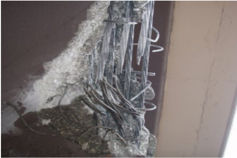
Figure 20: Severe II damage, three severed strands, NDOT Scottsbluff Gering Bypass Bridge, courtesy of NDOT
