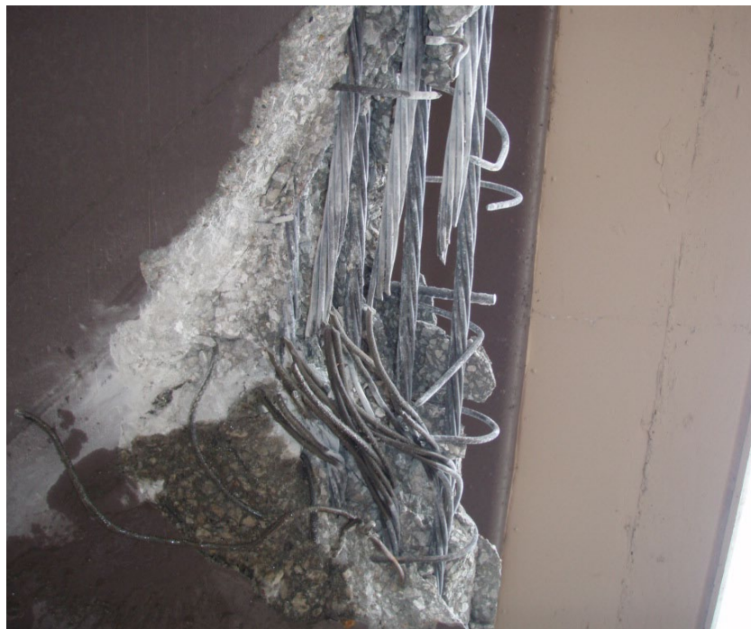
Figure 76: Level of damage, Scottsbluff Gering Bypass Bridge, courtesy of NDOT
