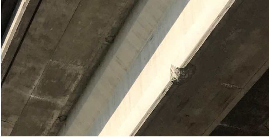
Figure 13: Minor damage, NDOT York Bridge East, courtesy of NDOT
