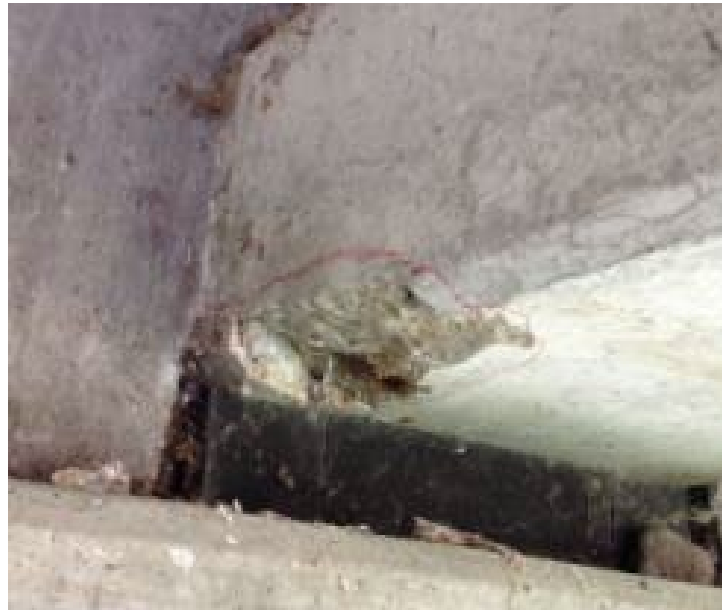
Figure 41: Condition State Poor, spalling on concrete bridge girder, courtesy of WisDOT, 2018
