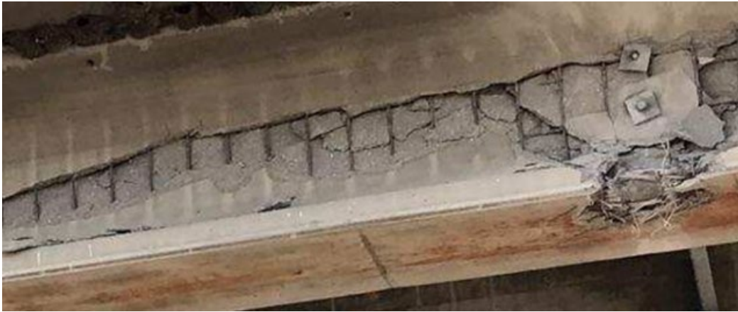
Figure 21: Severe III damage, several damaged strands, NDOT Schuyler Bridge, courtesy of NDOT
