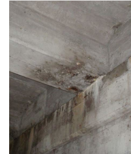
Figure 6: Extensive damage, water saturation, rust staining, and spalling on a cast-in-place concrete T-girder, MnDOT, 2019
