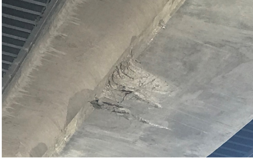
Figure 86: Damage at the patched area on Girder E, Wood River Interchange Bridge, courtesy of NDOT
