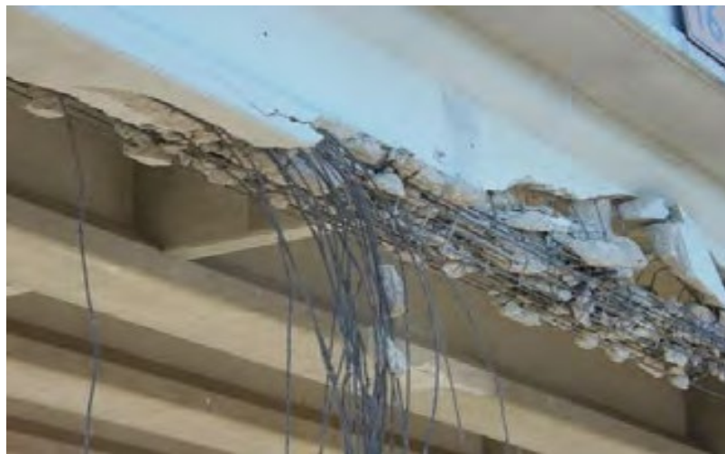
Figure 23: Severe III damage, several damaged strands, courtesy of Harries et al., 2012
