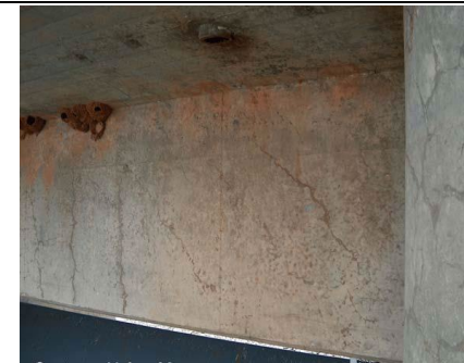
Figure 3: Moderate damage, hairline cracks, WisDOT, 2018
