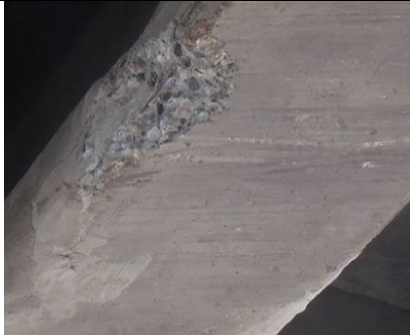
Figure 4: Moderate damage, one exposed strand on concrete bridge girder, WisDOT, 2018
