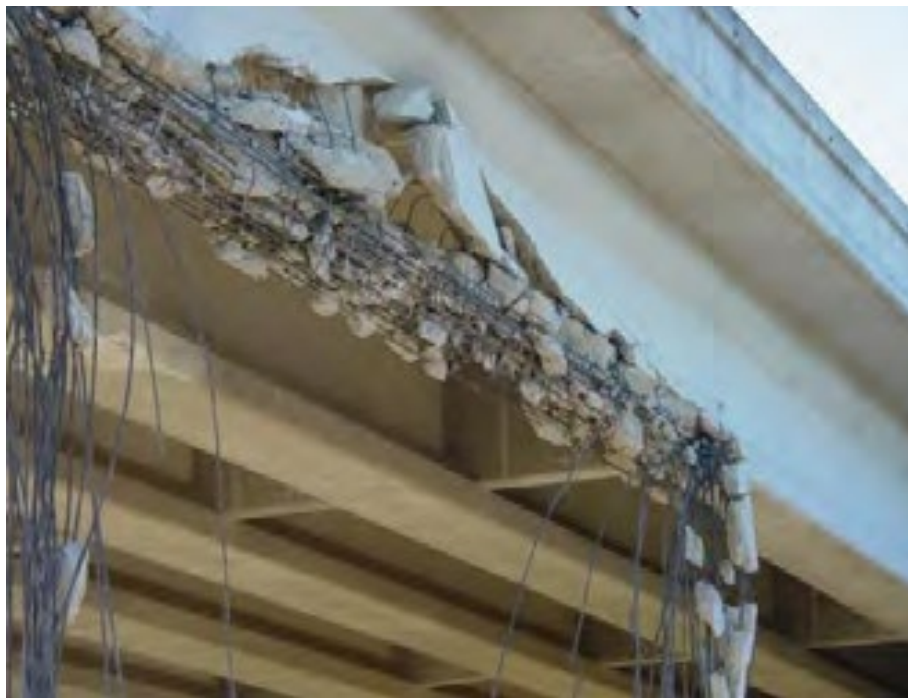
Figure 9: Exterior girder FM479 over Kerr Road, San Antonio TX. AASHTO I-girders; reported that the entire bridge was demolished and replaced, courtesy of Harries et al., 2012
