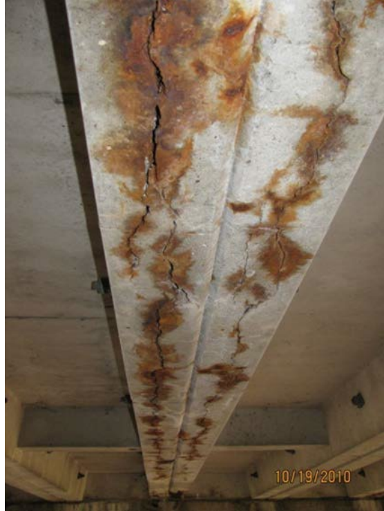
Figure 47: Condition State 3 cracking, delamination, and rust staining a precast concrete channel girder, courtesy of MnDOT, 2019
