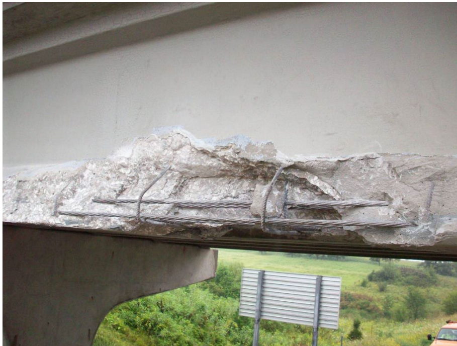
Figure 11: Bottom flange damage with mild reinforcing and prestressing strands intact, courtesy of Iowa DOT, 2014
