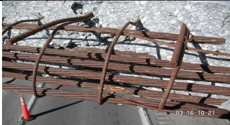
Figure 7: Severe I damage, one severed strand, NDOT Wood River Interchange Bridge Girder (A)
