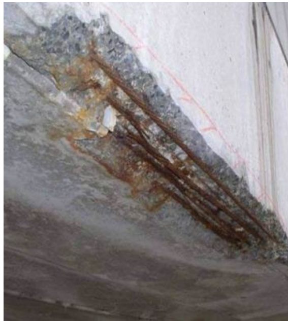
Figure 44: Condition State Poor, exposed strands on concrete bridge girder, courtesy of WisDOT, 2018
