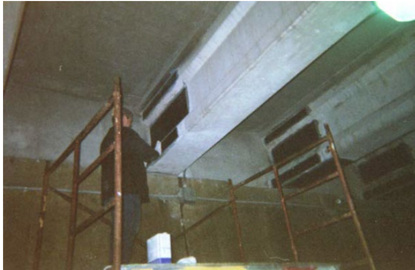
Figure 53: CFRP fabrics installation on I-65 expressway bridge girders, courtesy of Choo et al., 2013
