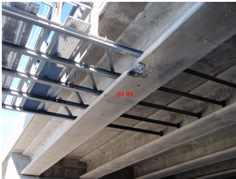
Figure 64: Level of damage, 168 th St. over West Dodge Road Bridge, courtesy of NDOT
