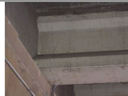
Figure 9: Severe damage, severe cracks, Choo et al., 2013
