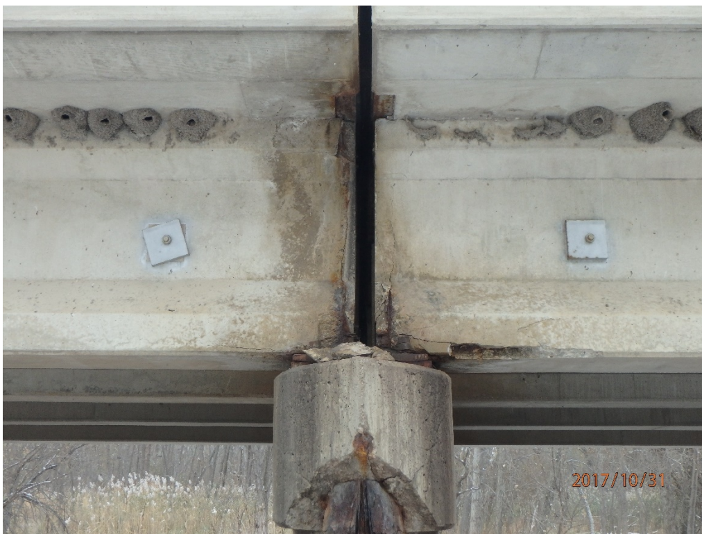
Figure 125: Damage at girder ends, Platte River South Bridge, courtesy of NDOT
