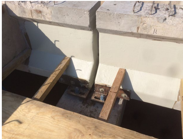
Figure 110: Girder end after CFRP confinement and bearing assemble replacement, Platte River Bridge East of Grand Island, courtesy of NDOT
