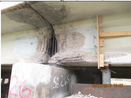
Figure 10: Severe damage, exposed strands > 15 %, MN/RC 2018-07 Report
