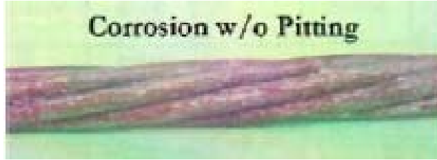
Figure 2: Moderate damage, exposed strands having corrosion without pitting, Naito et al., 2006
