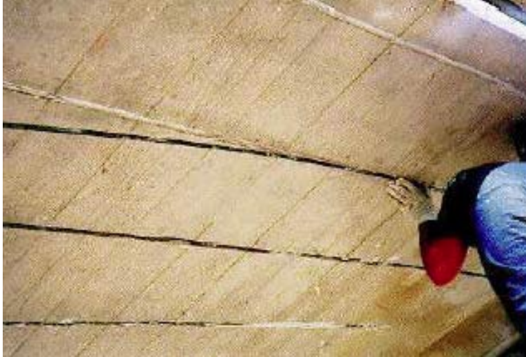
Figure 39: Use of near-surface mounted C-FRP in bridge decks, courtesy of Parretti et al 2004
