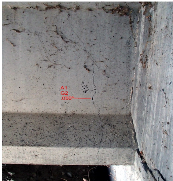
Figure 130: Cracking at girder end, Alma South Bridge, courtesy of NDOT
