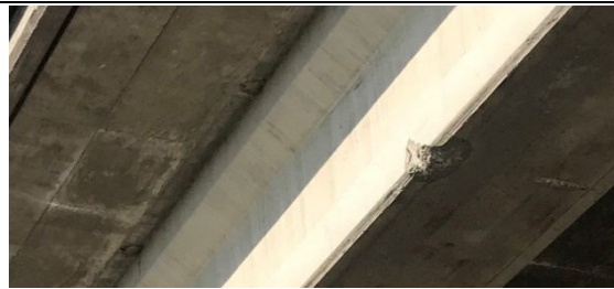
Figure 2: Minor damage, NDOT York Bridge East
