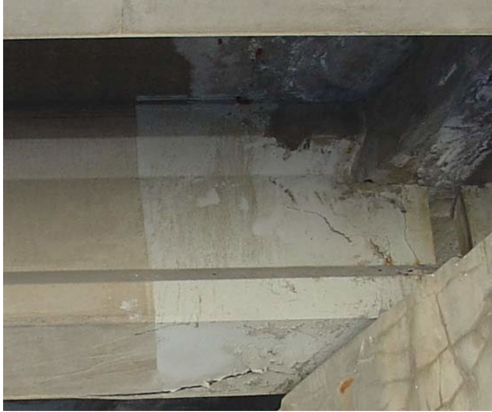
Figure 48: Severe class corrosion damage at girder end causing severe cracks, courtesy of Pantelides et al., 2010
