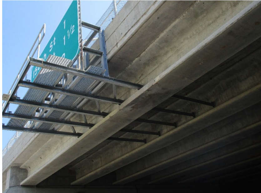
Figure 67: Repaired girder with no notable deficiencies, 168 th St. over West Dodge Road Bridge, courtesy of NDOT
