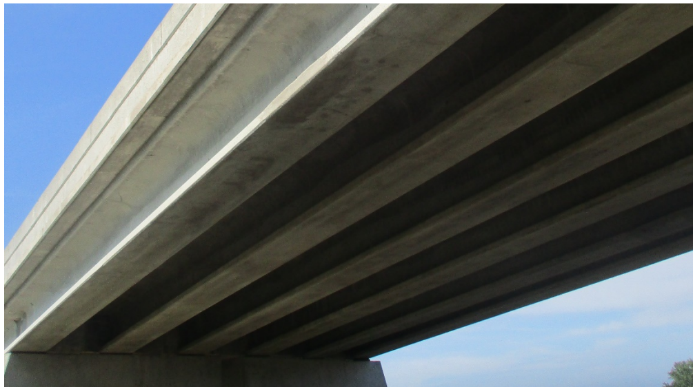
Figure 87: Patched area on Girder A, Wood River Interchange Bridge, courtesy of NDOT
