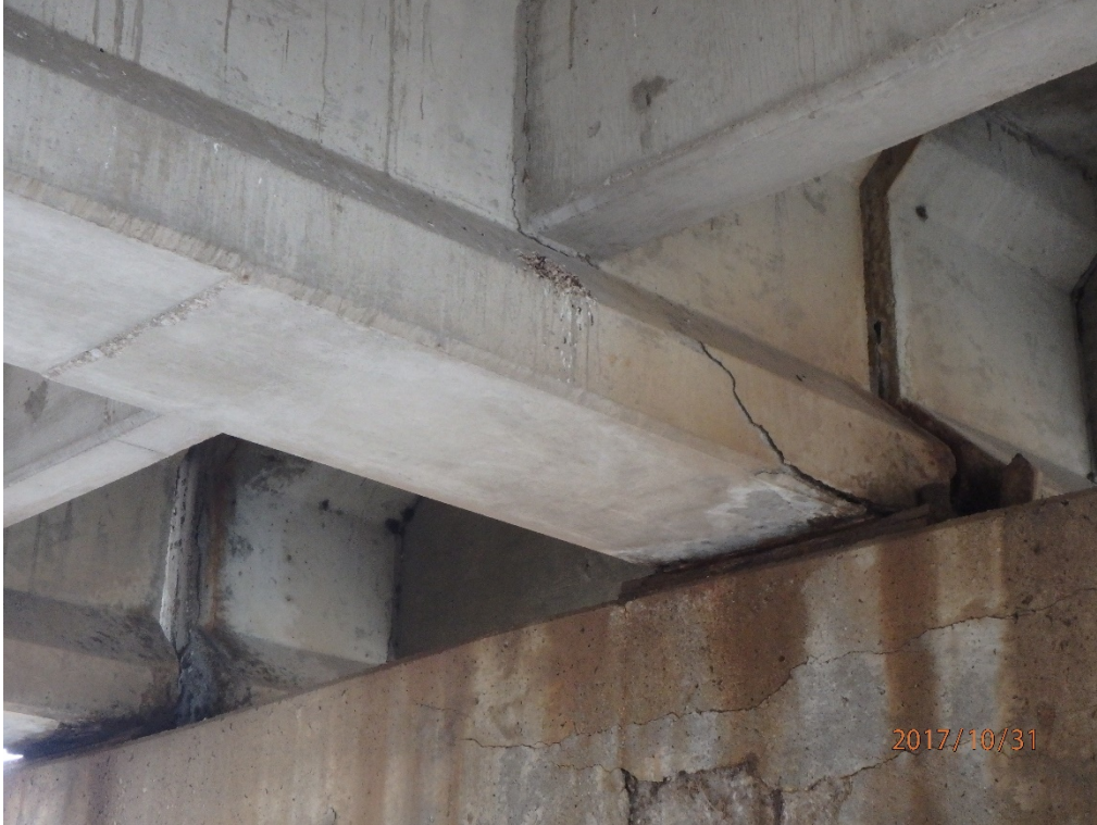
Figure 124: Damage at girder ends, Platte River South Bridge, courtesy of NDOT
