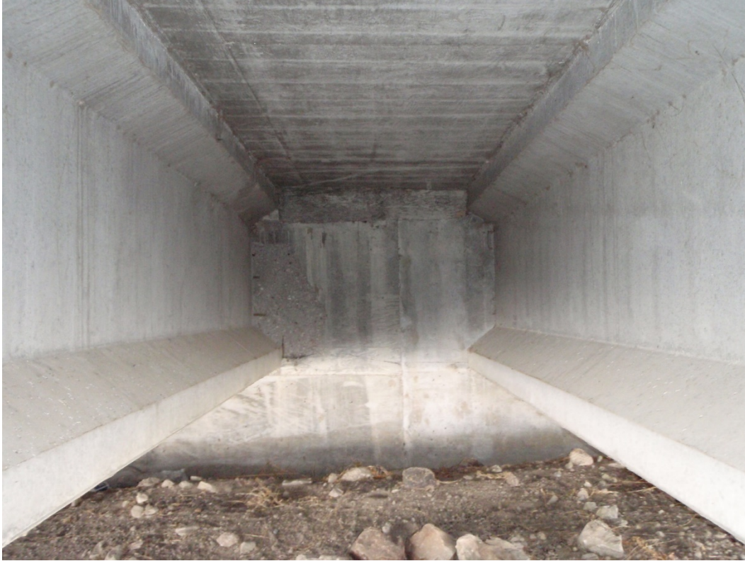
Figure 129: Exposed reinforcement at the abutment, Alma South Bridge, courtesy of NDOT
