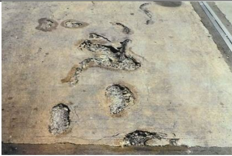
Figure 1: Minor damage, surface spalling with no exposed reinforcement, Naito et al., 2006
