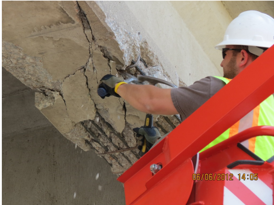
Figure 90: Removing all loose concrete immediately from the girder, York East Bridge, courtesy of NDOT
