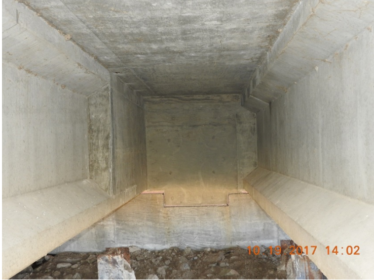
Figure 133: Repaired girder end with a concrete encasement, Alma South Bridge, courtesy of NDOT
