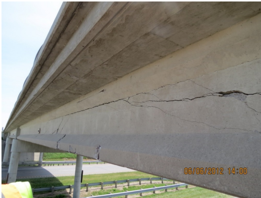
Figure 89: Level of damage, York East Bridge, courtesy of NDOT
