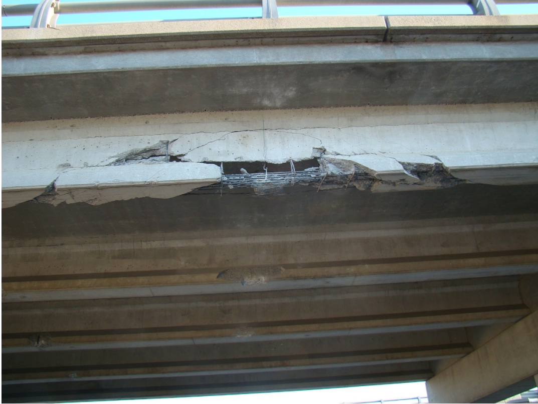
Figure 97: Level of damage, I-680 over US-75 Bridge, courtesy of NDOT
