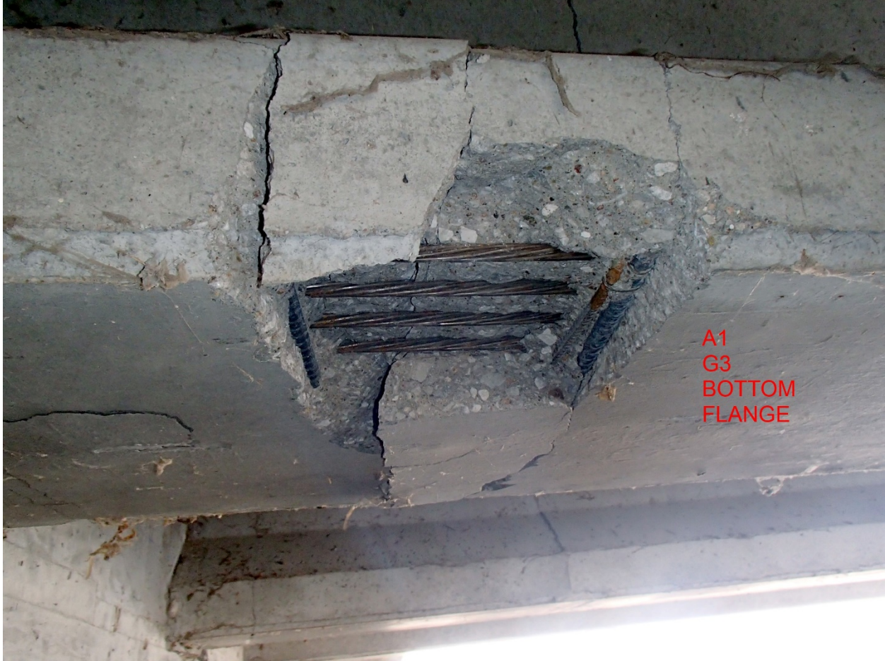
Figure 131: Exposed strands at bottom flange, Alma South Bridge, courtesy of NDOT
