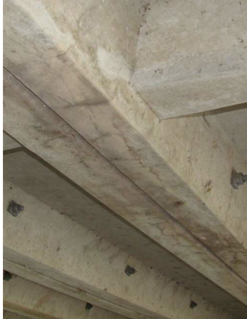
Figure 45: Condition State 2 cracking on precast concrete channel girders, courtesy of MnDOT, 2019
