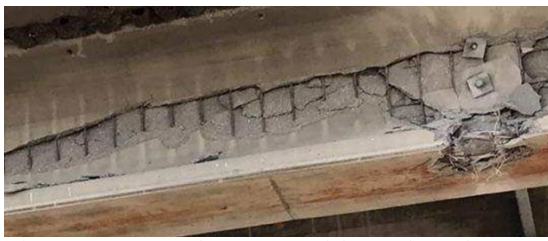
Figure 13: Severe III damage, several damaged strands, NDOT Schuyler Bridge
