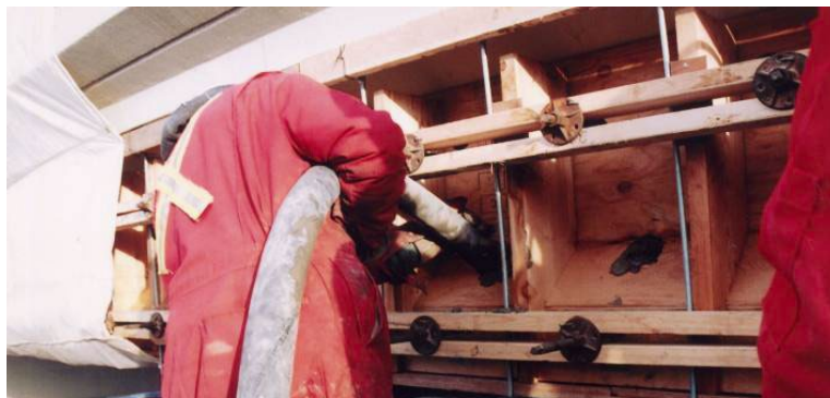
Figure 28: Pumping concrete into plywood formed section, courtesy of Alberta Infrastructure and Transportation, 2005
