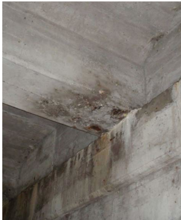
Figure 46: Condition State 3 water saturation, rust staining, and spalling on a cast-in-place concrete T-girder, courtesy of MnDOT, 2019
