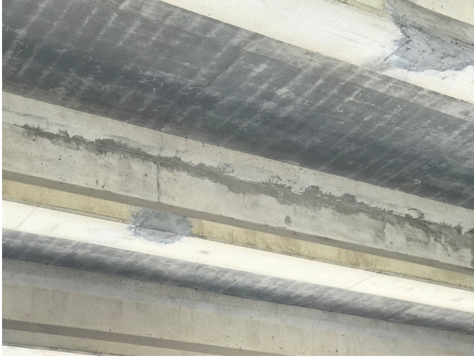
Figure 102: Girders with patching and epoxy injection works, I-680 over US-75 Bridge, courtesy of NDOT
