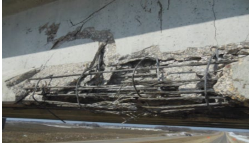
Figure 22: Severe III damage, several damaged strands, courtesy of Iowa DOT, 2014
