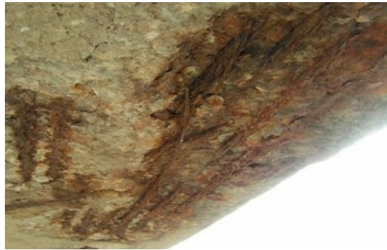
G: Complete loss of strand area
