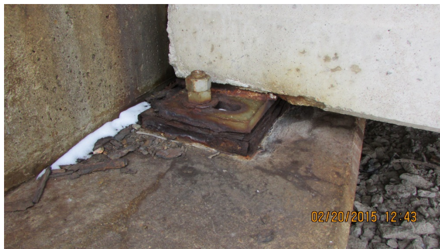
Figure 106: Corrosion damage at bearing assembly, Platte River Bridge East of Grand Island, courtesy of NDOT
