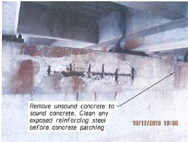
Figure 105: Corrosion damage at girder end and abutment, Platte River Bridge East of Grand Island, courtesy of NDOT
