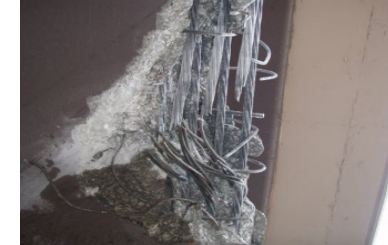
Figure 12: Severe II damage, three severed strands, NDOT Scottsbluff Gering Bypass Bridge
