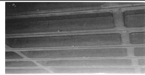
Figure 3: Minor damage, bottom flange cracks, Feldman et al., 1996
