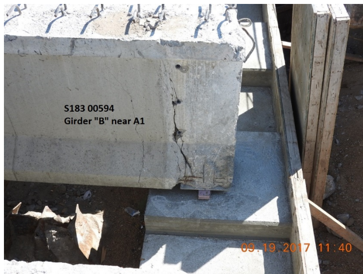
Figure 132: Heavy cracking at girder end, Alma South Bridge, courtesy of NDOT
