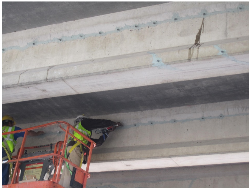
Figure 24: Epoxy injection process done in I-680 over US-75 Bridge, courtesy of NDOT
