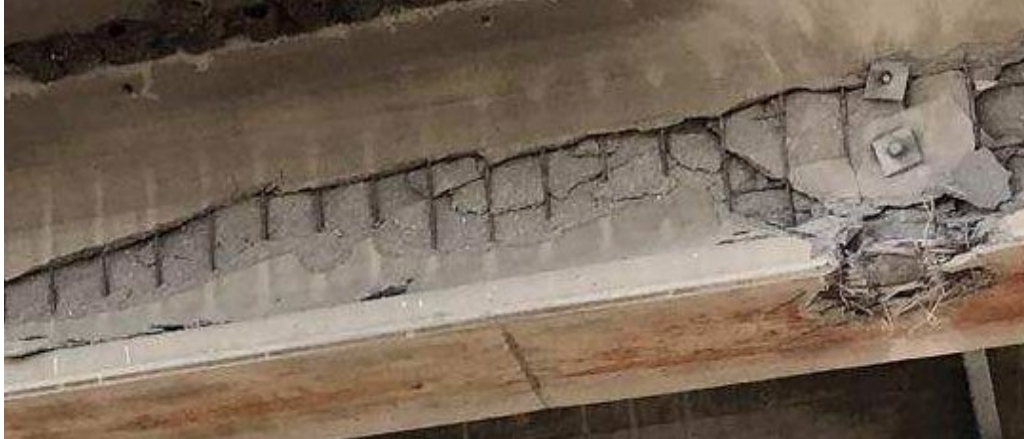
Figure 71: Level of damage, Schuyler Bridge, courtesy of NDOT
