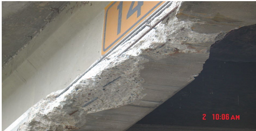
Figure 14: Moderate damage, exposed intact strands, courtesy of Pantelides et al., 2010
