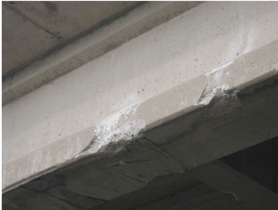
Figure 10: Minor bottom flange spalling, courtesy of Iowa DOT, 2014
