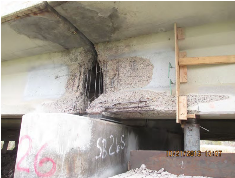
Figure 50: Severe class corrosion damage at girder end, MN/RC 2018-07 Report
