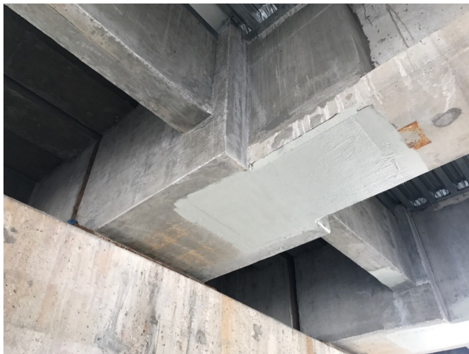
Figure 118: Girder end encasement and CFRP layers, visible crack at the diaphragm, Kearney South Platte River Bridge, courtesy of NDOT
