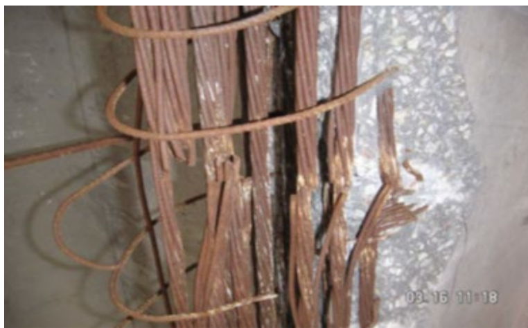
Figure 18: Severe II damage, five severed strands, NDOT Wood River Interchange Bridge Girder (E), courtesy of NDOT
