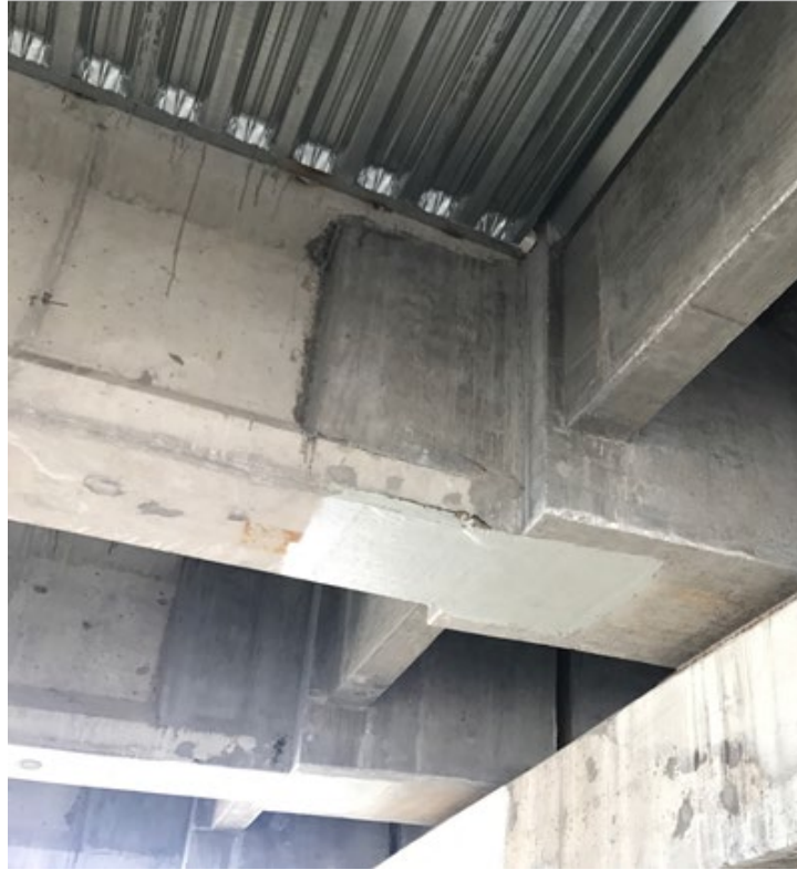
Figure 117: Girder end encasement and CFRP layers, Kearney South Platte River Bridge, courtesy of NDOT
