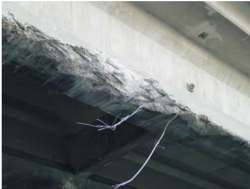
Figure 7: AASHTO I-girder; reportedly repaired, courtesy of Harries et al., 2012
