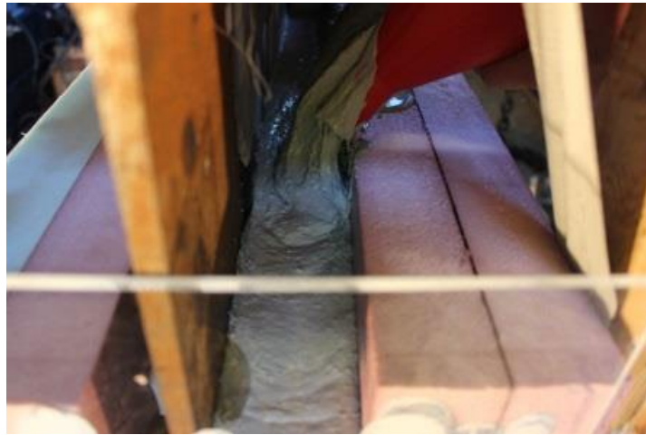
Figure 58: Casting UHPC at a steel girder end from the top of formwork, courtesy of Zmetra, 2015
