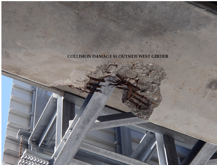
Figure 65: Level of damage, 168 th St. over West Dodge Road Bridge, courtesy of NDOT
