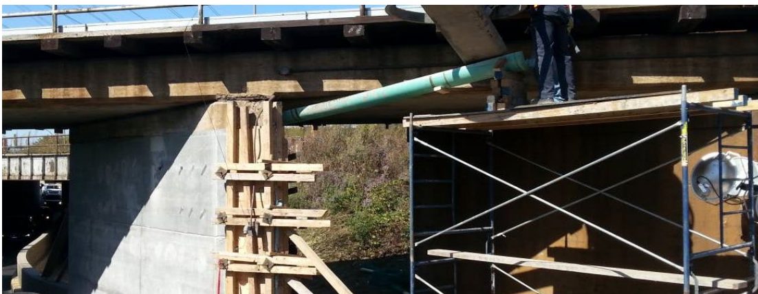
Figure 59: Casting UHPC for a thin jacket for a bridge pier from the top of formwork, CN Rail bridge, Quebec, Canada, obtained from Ductal website
