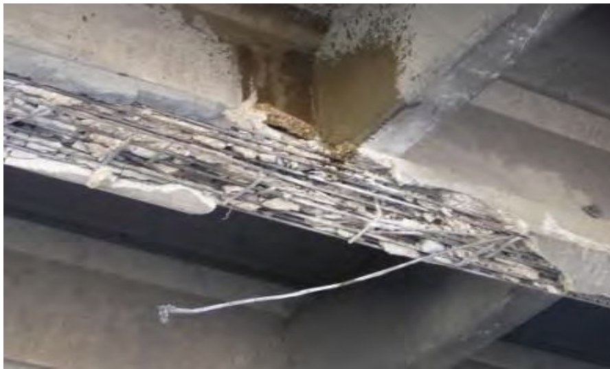
Figure 17: Severe I damage, one severed strand, courtesy of Harries et al., 2012
