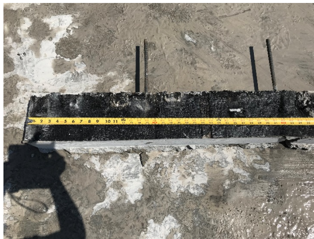
Figure 27. Segment B1: Perfect Membrane 0-22” and 2” Gap 22-23”.
