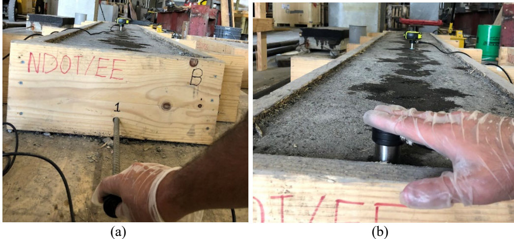
Figure 18. Two longitudinal continuous test setups: (a) UGWL Method application. Transmitter on the end of rebar and receivers along the middle line on the asphalt surface ( Results in Figure 19 ). (b) Indirect UPV Application. Transmitter on the asphalt surface 2 inches from the edge and receivers along the middle line on the asphalt surface ( Results in Figures 20-21 ).
