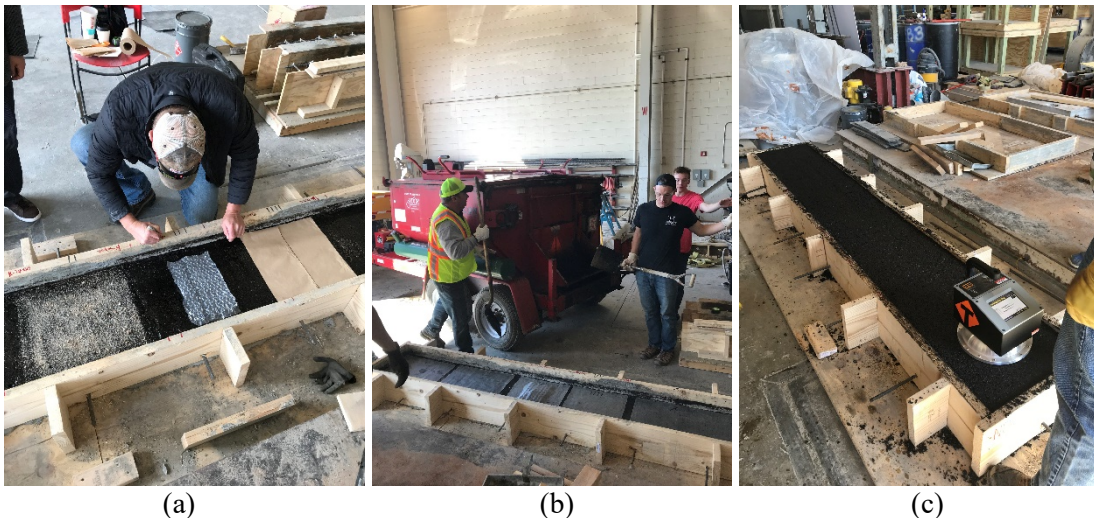
Figure 6. (Casting of Specimen B: (a) Placement of gravel (B2), bubble wrap (B3), and paper towel (B4) between primer and membrane; (b) Image after membranes are placed; (c) In-situ Density measurements
