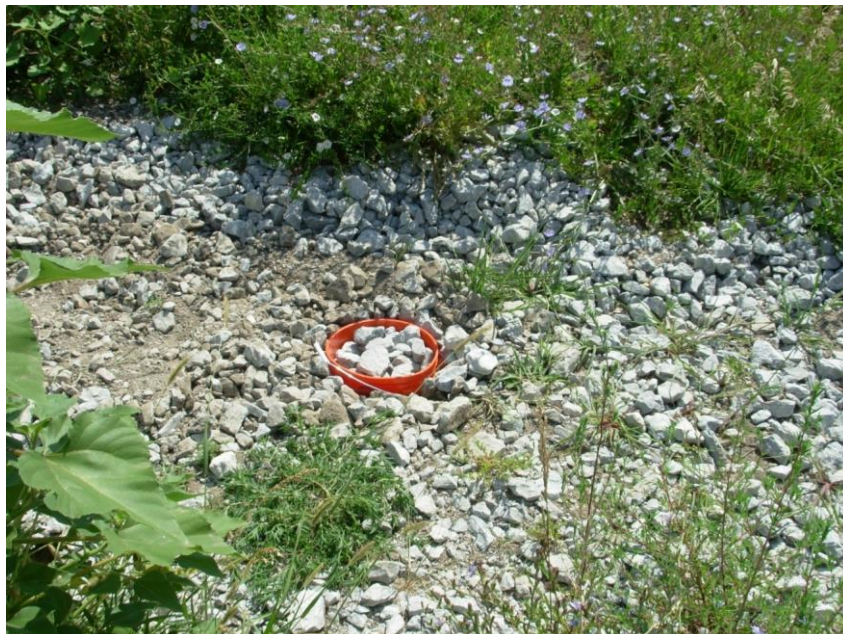
Figure B.11 Sediment bucket in infiltration trench
