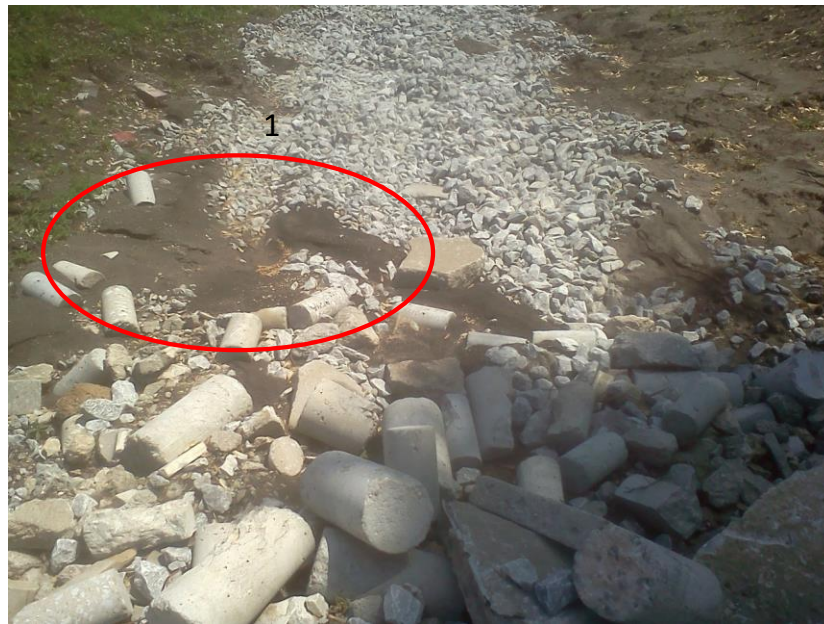
Figure 2.21 Filter trench sediment buildup on armorings and check dams
