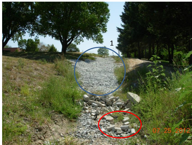
Figure 2.24 Filter trench added 1-3 inch rock at beginning and check dam material migration (water flow direction: from the top to bottom of the picture)
