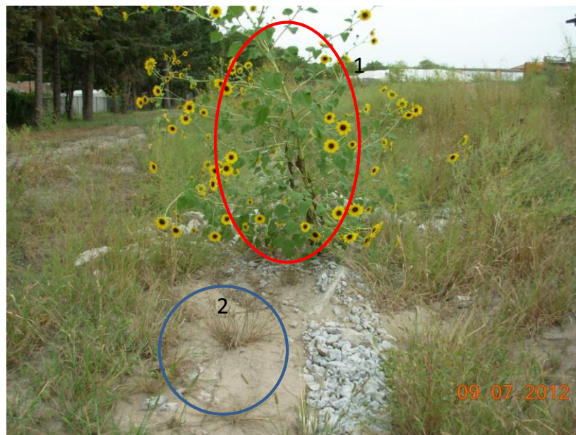
Figure 2.22 Filter trench sediment buildup and vegetative growth
