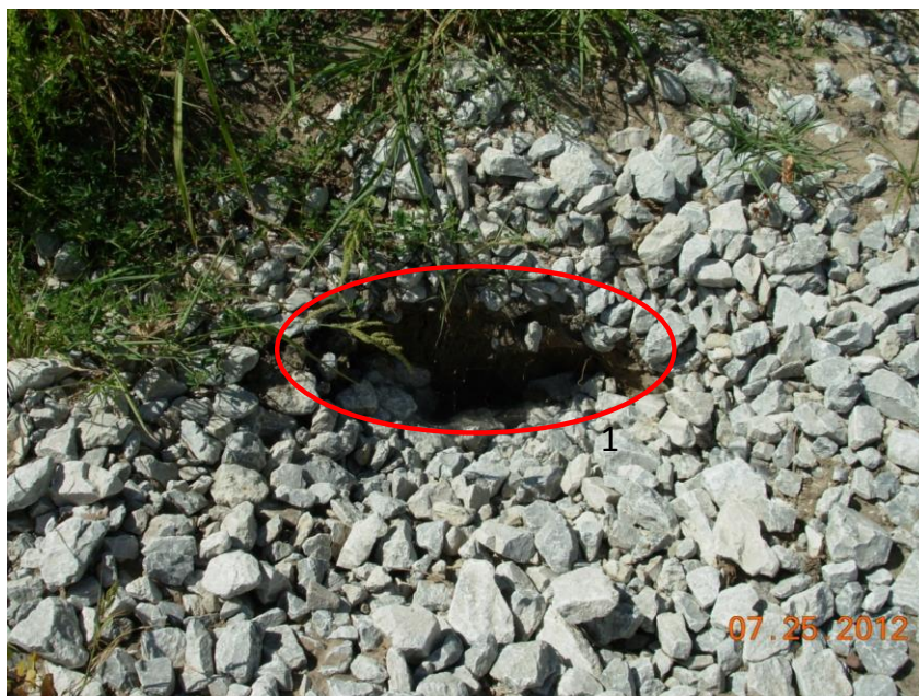
Figure 2.25 Filter trench undermining hole along trench
