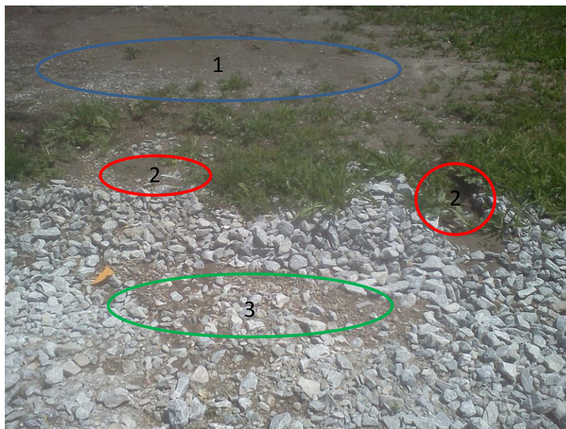
Figure 2.19 Infiltration trench clogging
