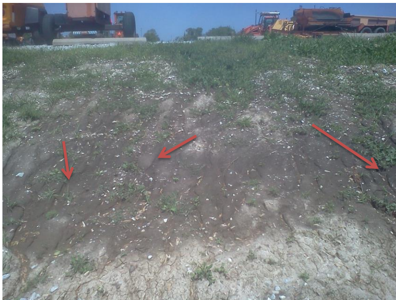
Figure 2.20 Filter trench side slope rills
