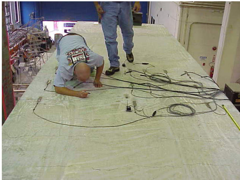
Figure 7-8: Mapping of Initial Cracks
