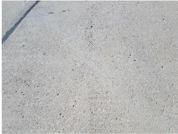
Figure A.90: Deck cracks on bridge SS66C00220.
