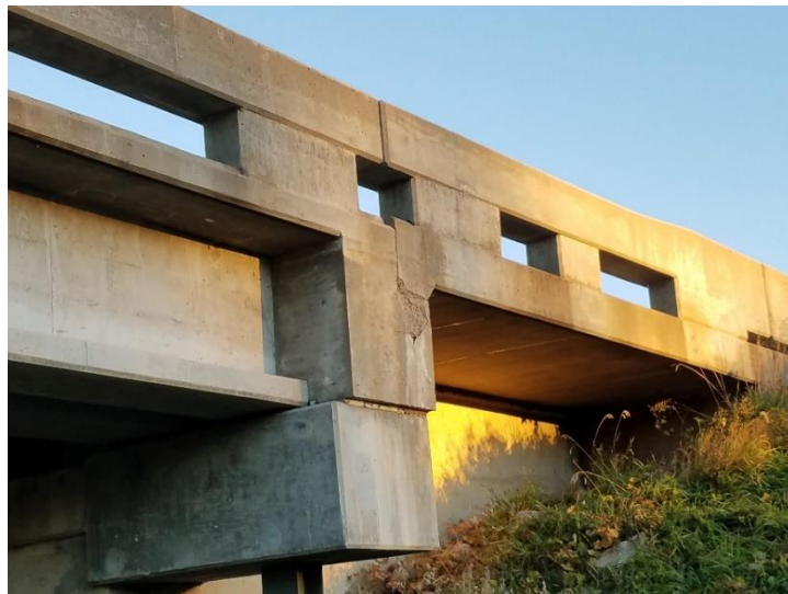
Figure A.80: Damaged abutment on bridge S103 02465.
