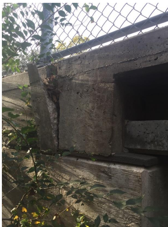
Figure A.53: Damaged east abutment on bridge S058 00994.
