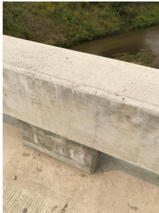
Figure A.111: Cracked rail on bridge C004931110.
