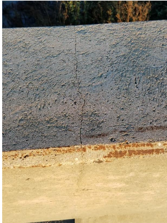
Figure A.83: Cracked rail on bridge S103 02465.
