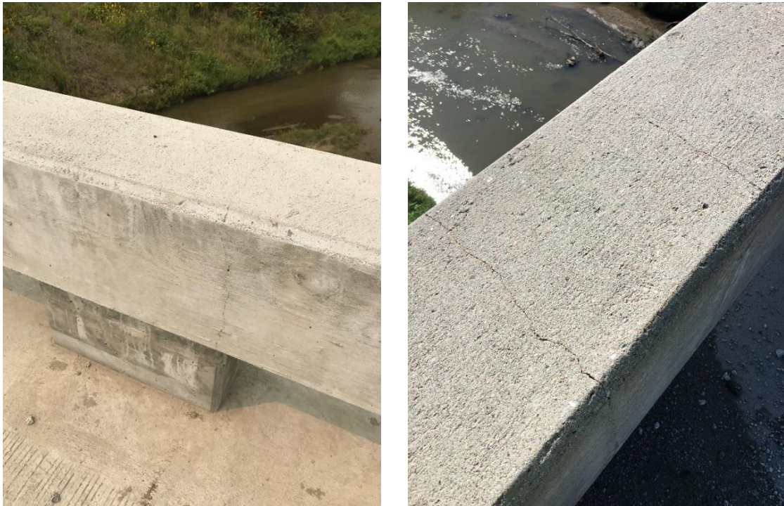
(a) (b) Figure 3.12: Examples of cracked bridge rails.
