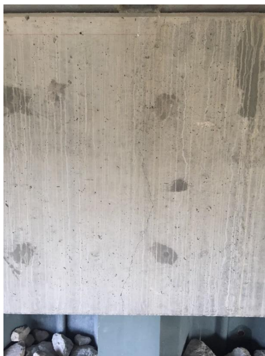
Figure A.45: Cracked abutment cap on bridge S050 06686.
