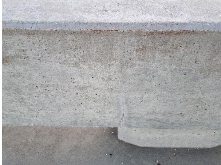
Figure A.35: Cracked rail on bridge S034 31644.
