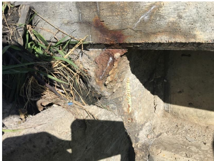
Figure A.87: Damaged abutment on bridge S275 18587.
