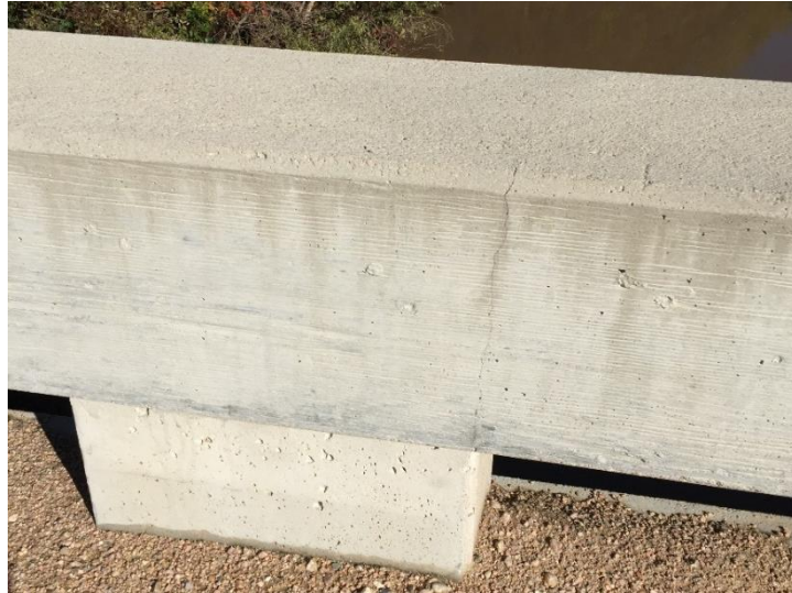
Figure A.102: Cracked rail on bridge C008504145.
