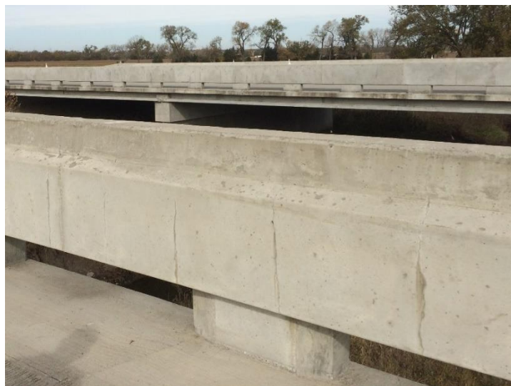
Figure A.65: Cracked rail on bridge S080 40927R.
