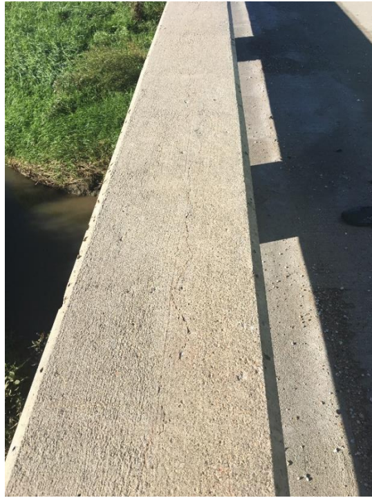
Figure A.19: Cracked rail on bridge S006 34277.
