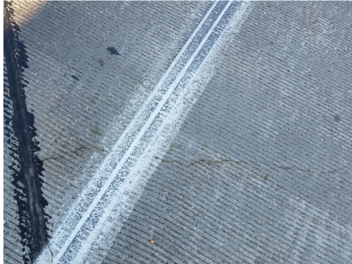
Figure A.22: Deck crack on bridge S009 00888.
