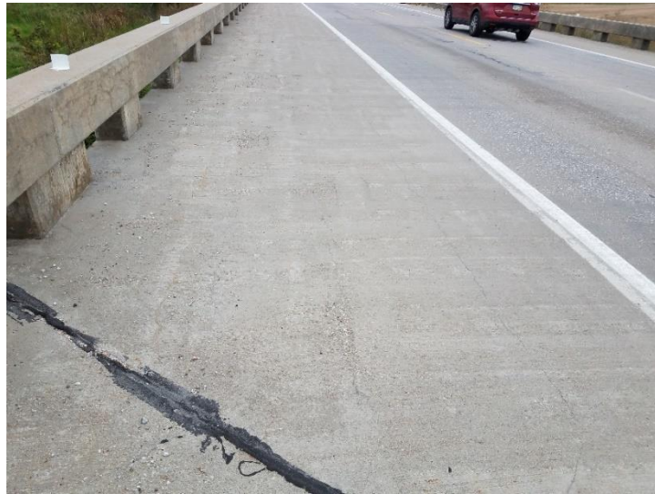
Figure A.11: Deck cracks on bridge S006 34277.
