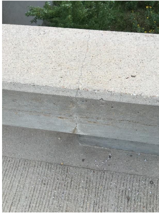
Figure A.40: Cracked rail on bridge S050 04149.
