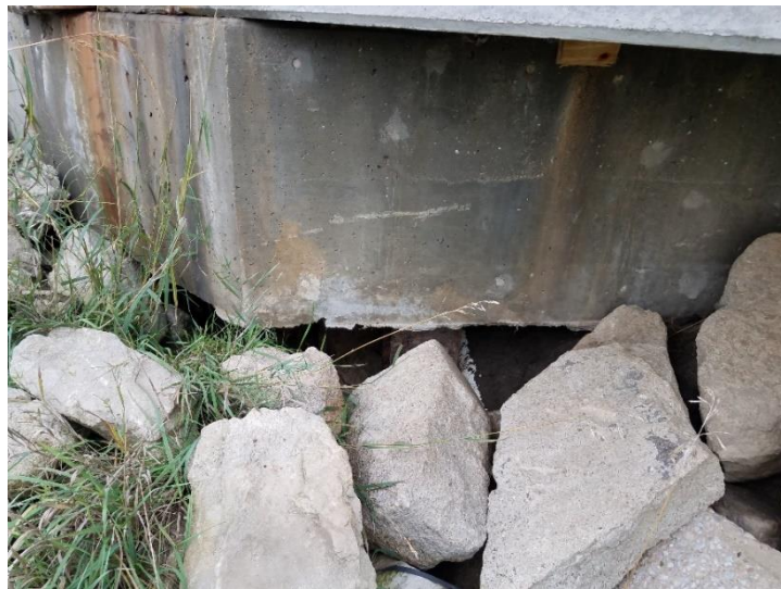
Figure A.18: Washout under south abutment on bridge S006 34277.
