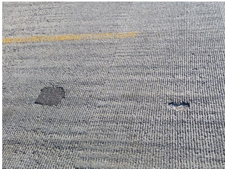
Figure A.23: Small deck potholes on bridge S009 00888.
