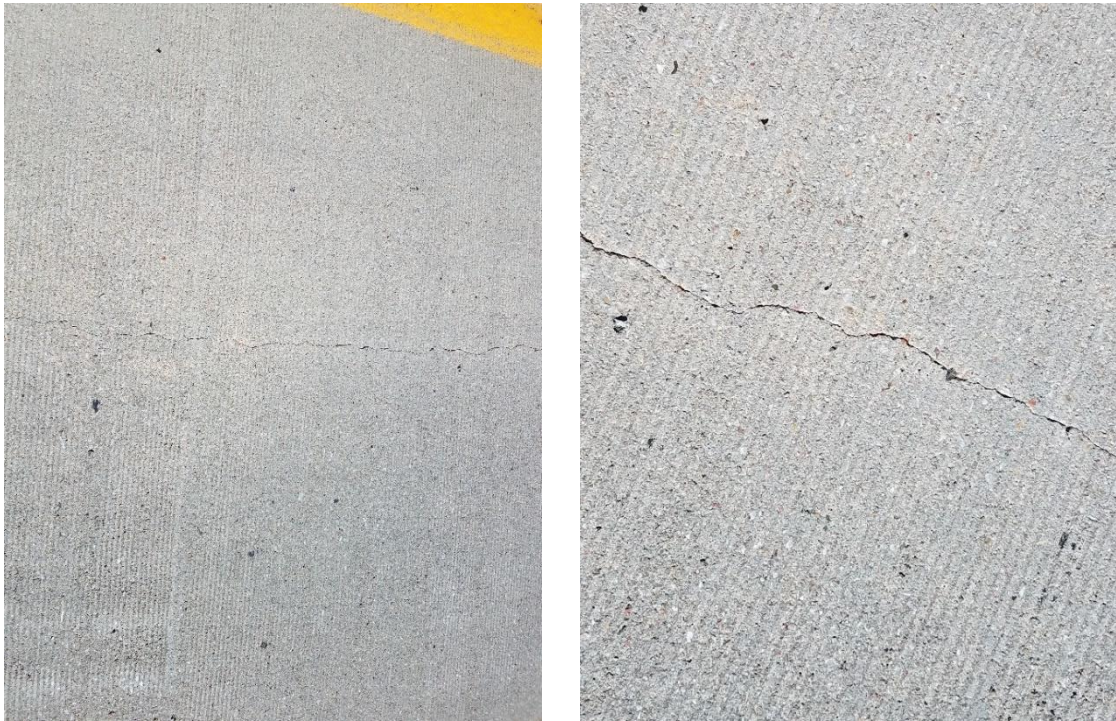
(a) (b) Figure A.3: Deck cracks on bridge S006 26001.
