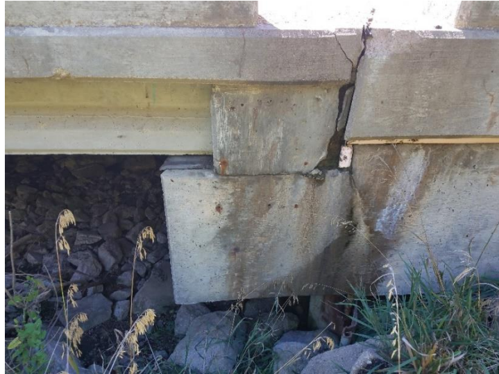
Figure A.7: Damaged northwest abutment on bridge S006 26001.
