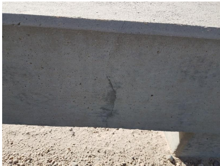
Figure A.106: Cracked rail on bridge M011022220.
