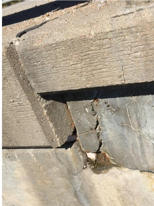
Figure A.5: Damaged southwest abutment on bridge S006 26001.
