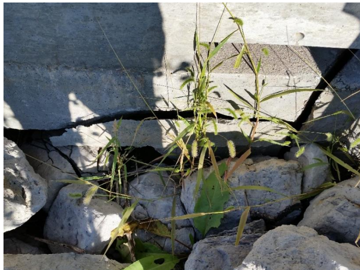
Figure A.16: Damaged north abutment on bridge S006 34277.
