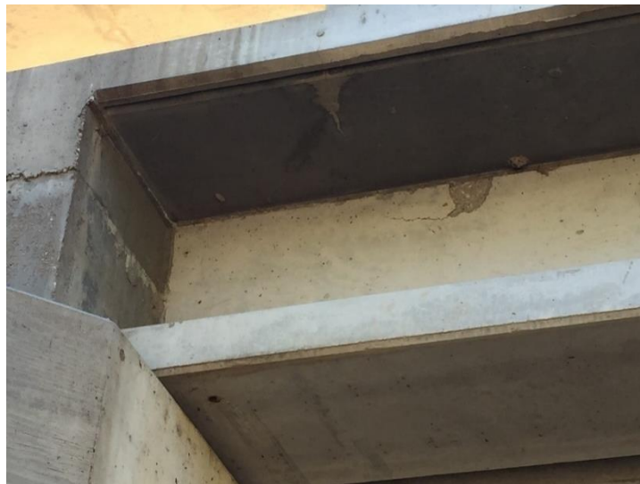
Figure A.101: Chipped girder on bridge C008504145.
