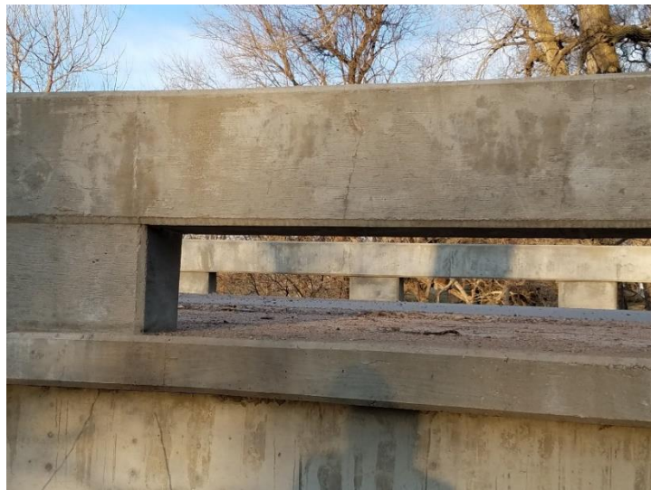
Figure A.97: Cracked rail on bridge C002408505.
