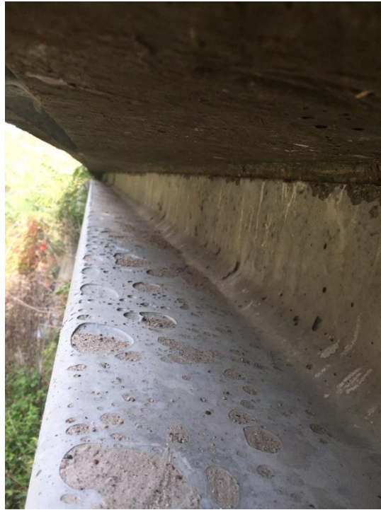
Figure A.55: Damaged girder flange caused by water entrapment in concrete forms on bridge S058 00994.
