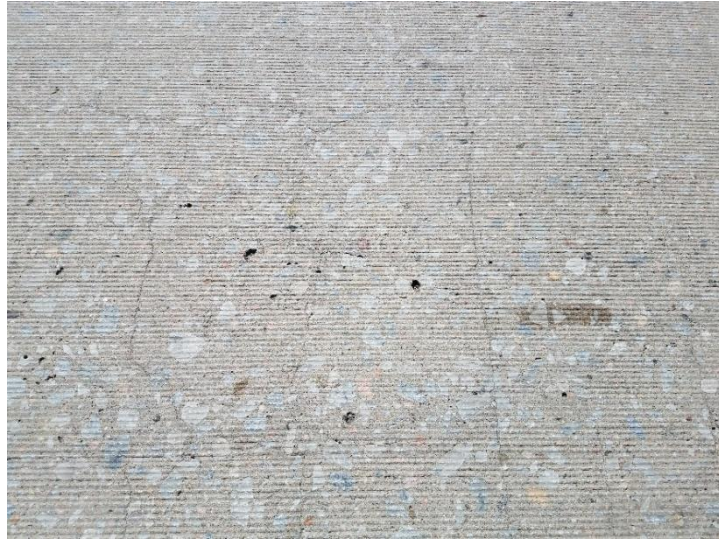
Figure A.72: Deck cracks on bridge S089 06047.
