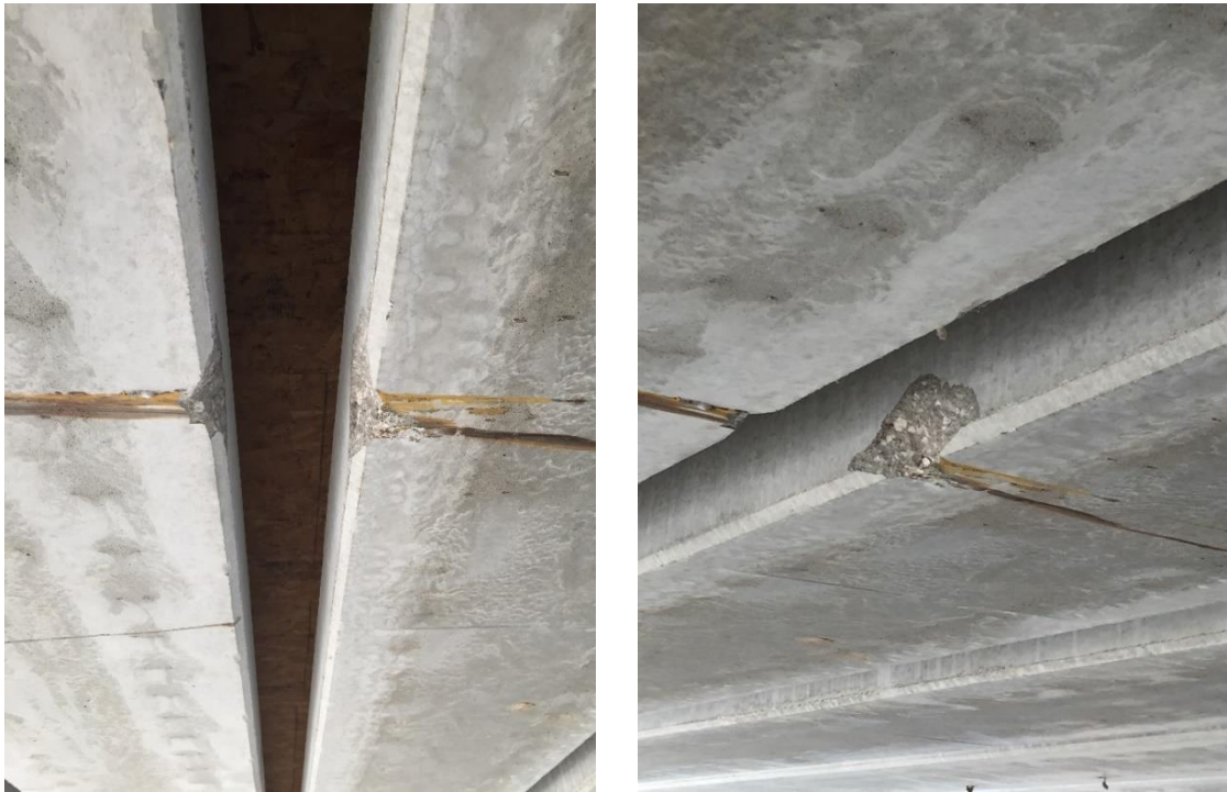
(a) (b) Figure A.47: Chipped girders on bridge S050 06686.
