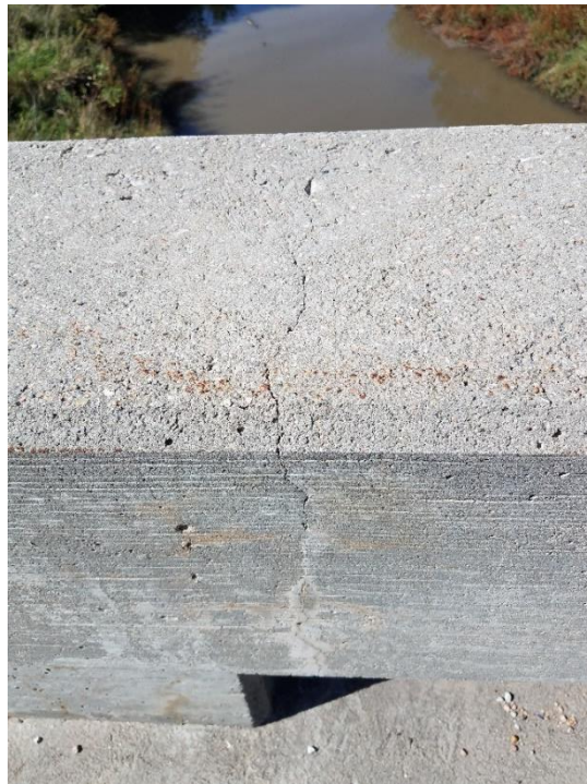
Figure A.69: Cracked rail on bridge S081 05152L.
