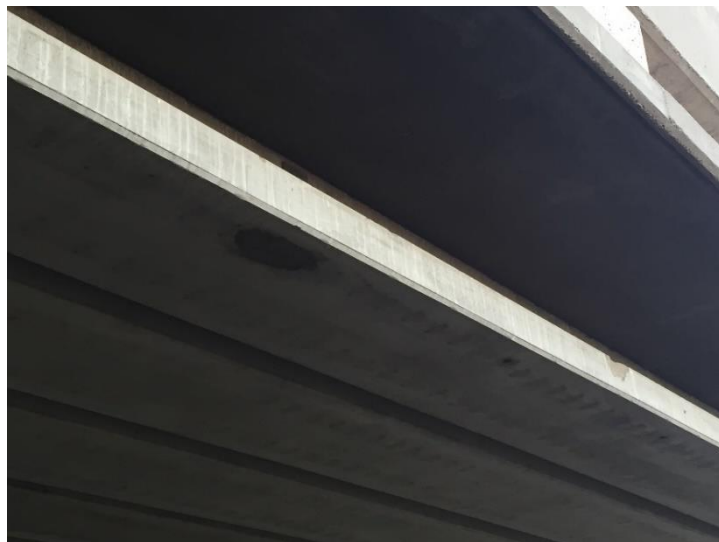
Figure A.34: Chipped and patched girder on bridge S034 31644.
