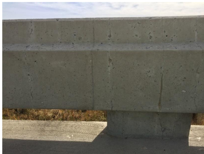
Figure A.61: Cracked rail on bridge S080 40872R.
