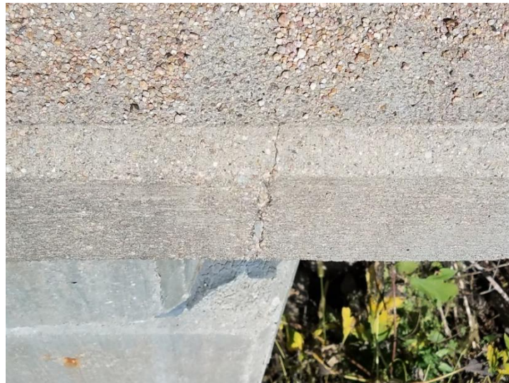
Figure A.4: Full-depth deck crack on bridge S006 26001.
