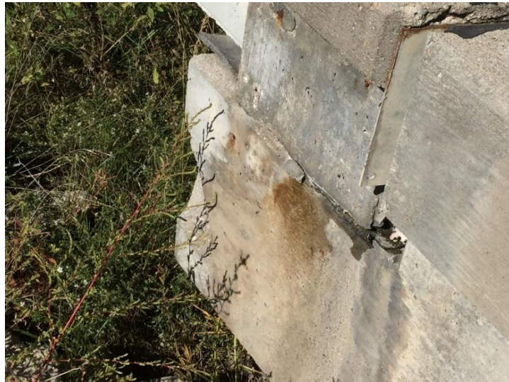
Figure A.6: Damaged southeast abutment on bridge S006 26001.
