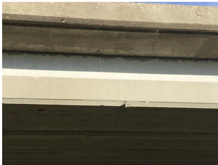
Figure A.27: Chipped girder on bridge S009 00888.
