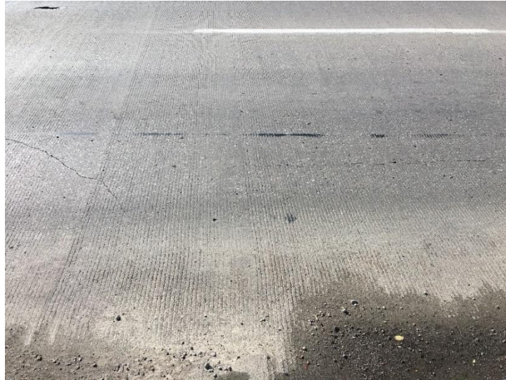
Figure A.86: Deck cracks on bridge S275 18587.
