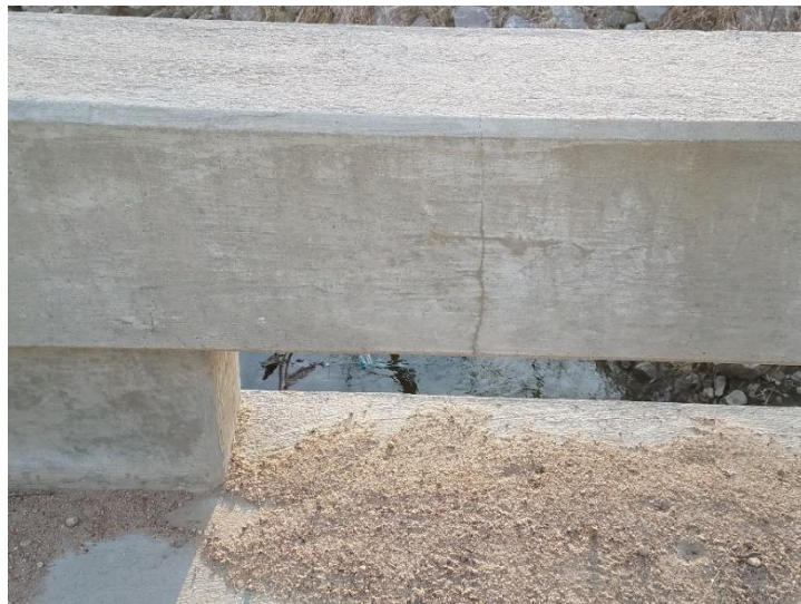
Figure A.73: Cracked rail on bridge S089 06047.
