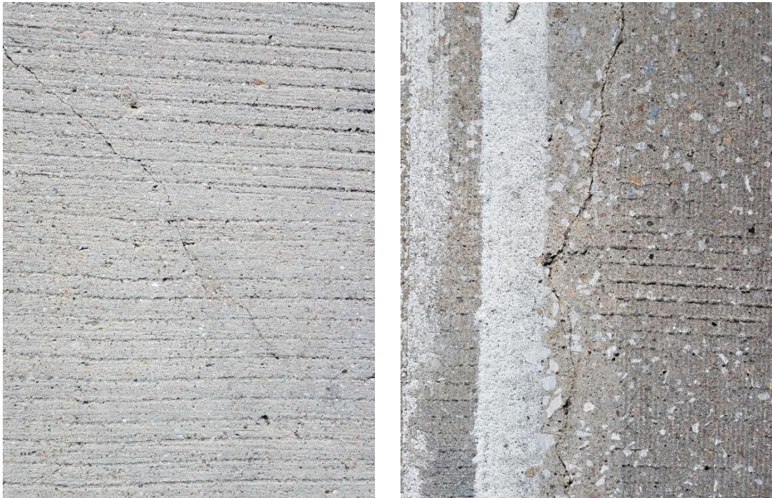
(a) (b) Figure A.68: Deck cracks on bridge S081 05152L.
