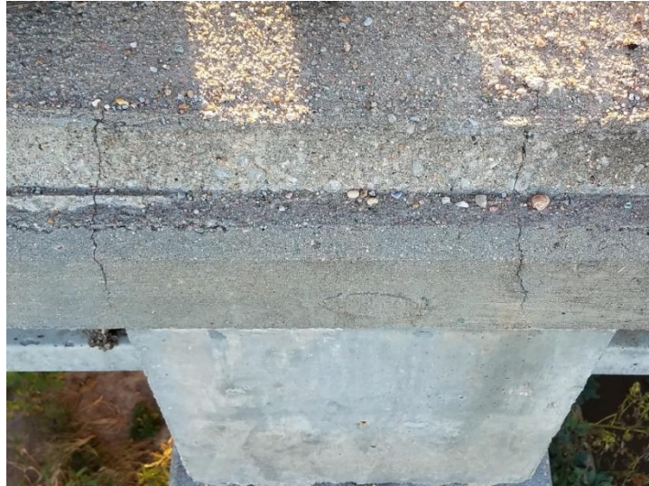
Figure A.79: Full-depth deck crack on bridge S103 02465.
