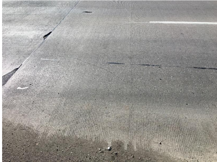
Figure 3.5: Example of diagonal deck cracking.
