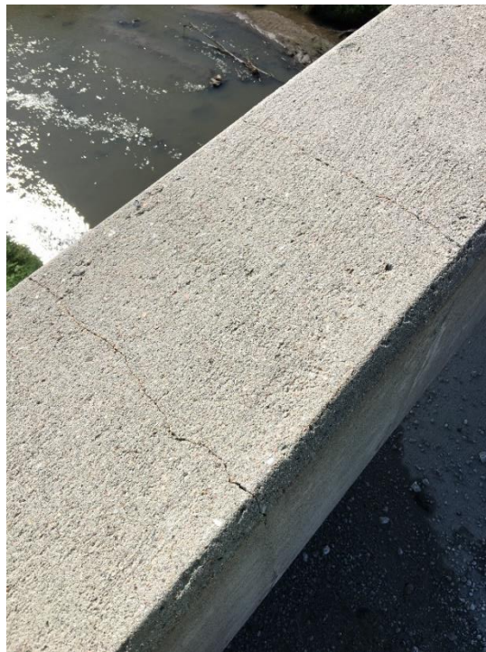
Figure A.48: Cracked rail on bridge S050 06686.
