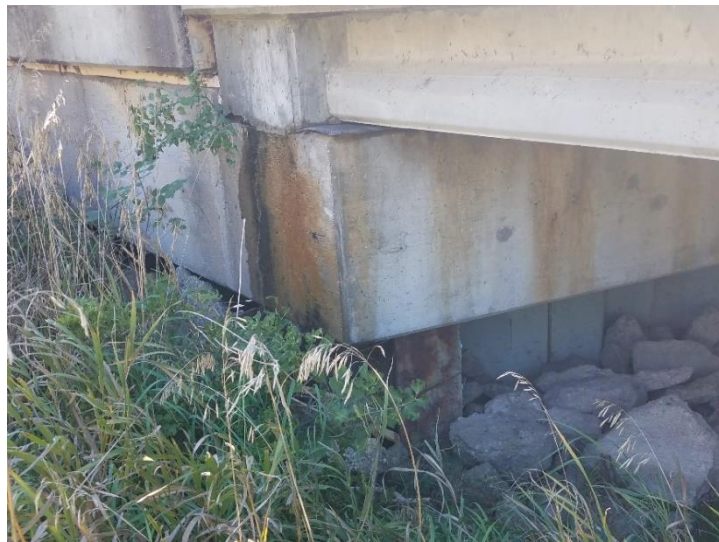
Figure A.8: Damaged northeast abutment on bridge S006 26001.
