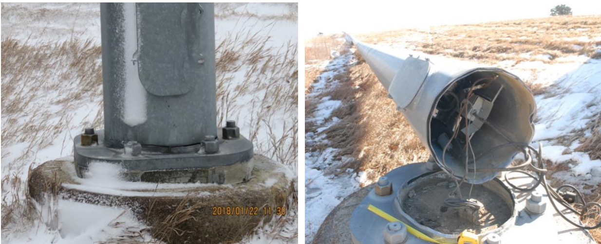
(a) High Mast Tower Base Plate, Anchor, Non-shrink Grout, and Cast-in-Place Foundation (b) High Mast Tower Failure (Milford, Nebraska, January, 2018)
