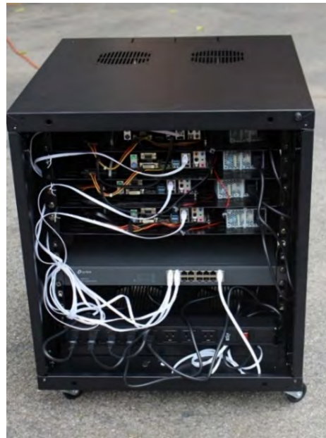
Fig. 2.2. Modular data collection system in which the SBCs are placed at the top of the rack, the network switch is in the middle of the rack, and power distribution and batteries are at the bottom of the rack
