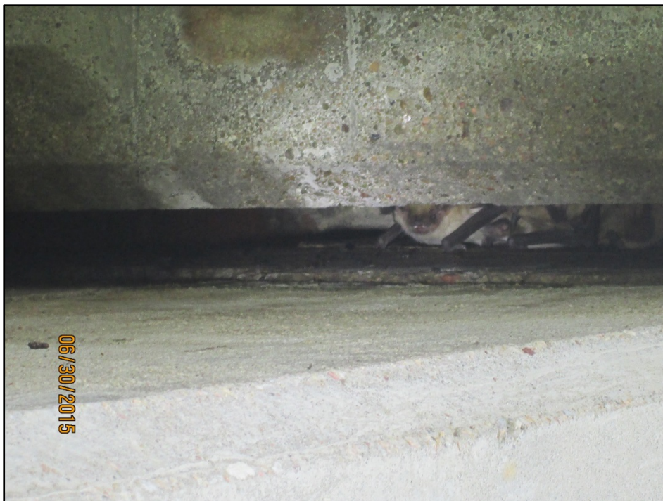
Photo 8: Bats in crevice of bridge. Orientation: South
