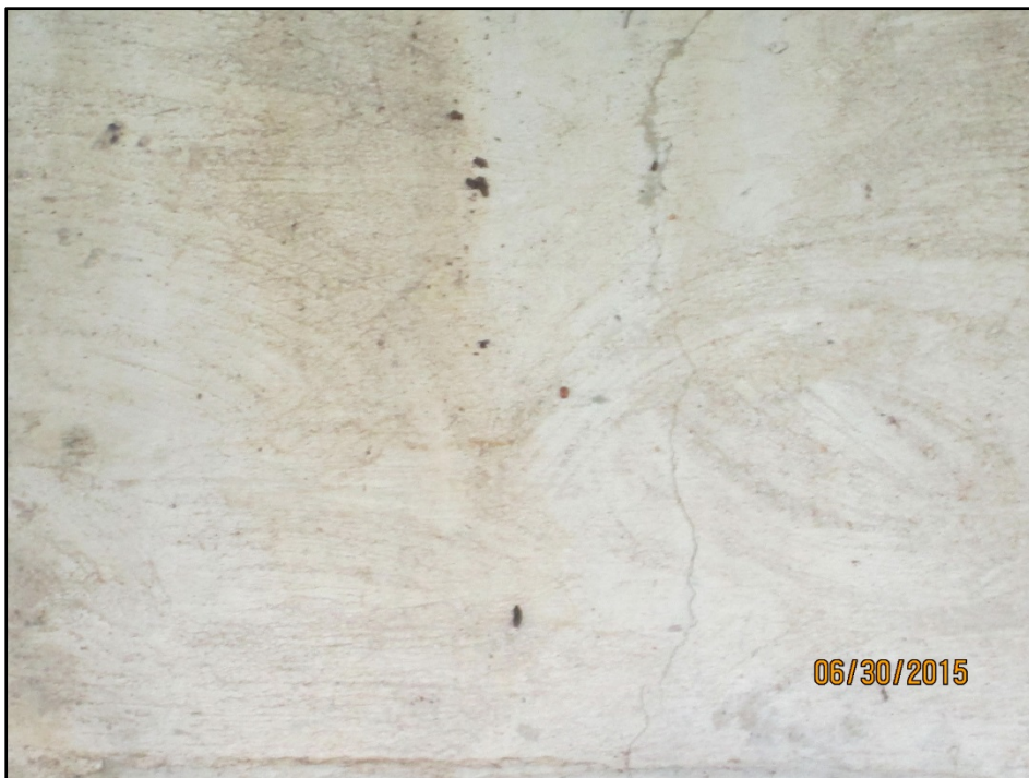
Photo 4: Bat guano on bridge side. Orientation: West
