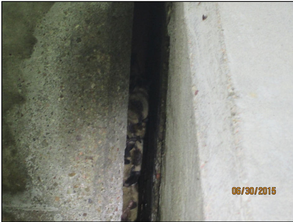
Photo 5: Bats in crevice of bridge. Orientation: South
