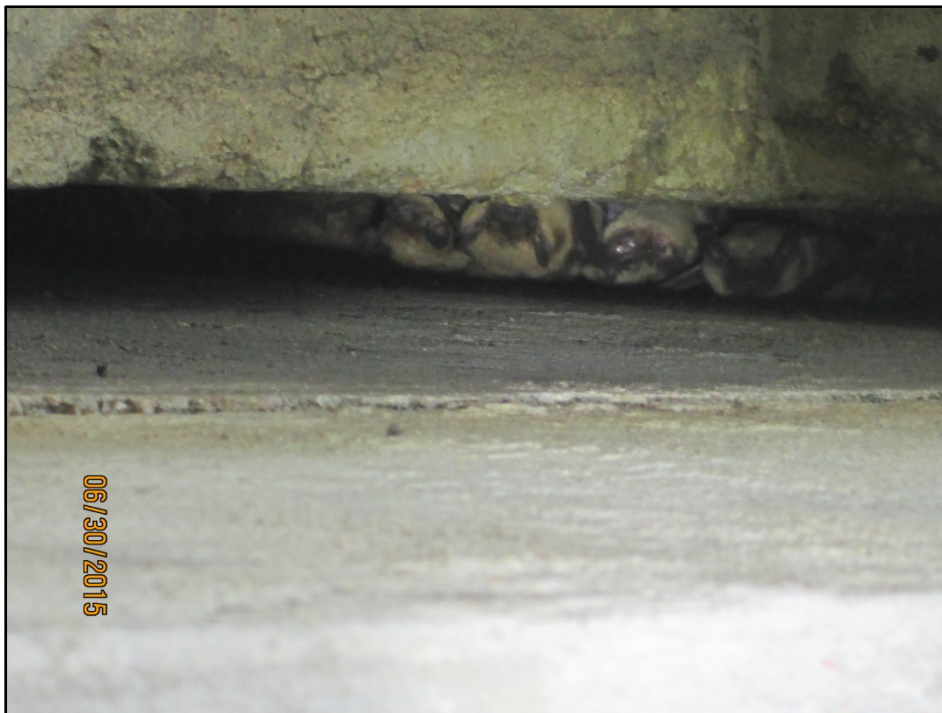
Photo 7: Bats in crevice of bridge. Orientation: South
