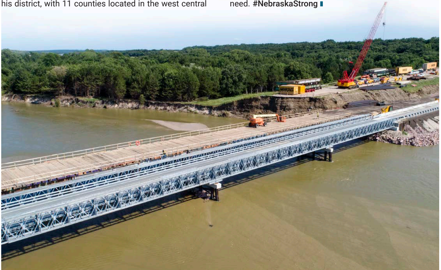
Governor Pete Ricketts joined the NDOT and others on July 29 to celebrate the opening of a temporary bridge on US-281 over the Niobrara River. The roadway was destroyed when the river broke the levee and dam south of Spencer in March.
