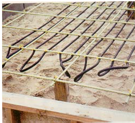
Figure 2.6 Deck heating system on approaches of a pedestrian overpass in Lincoln, Nebraska, 1993
