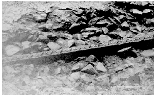
Figure 2.2 Spalling of concrete surface, exposing a reinforcing bar
