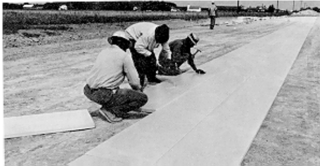
Figure 2.4 Styrofoam insulating layer used on graded subgrade for flexible pavement in Michigan (1962)
