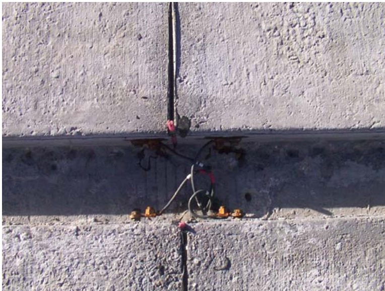
Figure 6-6 Power Chord and Angle Iron Connection
