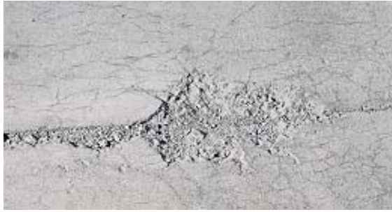
Figure 2.1 D-line cracking spreading from sidewalk joint
