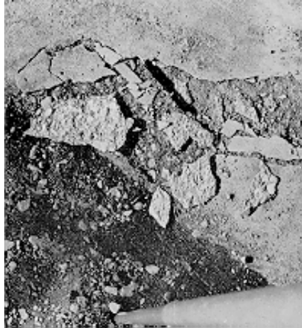
Figure 2.3 Scaling of concrete slab surface
