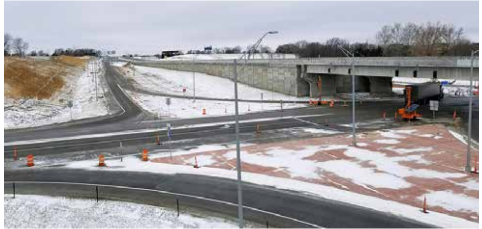
Photo by Chris Hasenbank, Tecumseh Construction Office The eastbound Highway 2 off ramp in the background connects eastbound Highway 2 with Highway 73/75 north and south, part of the Nebraska City Southeast project.
